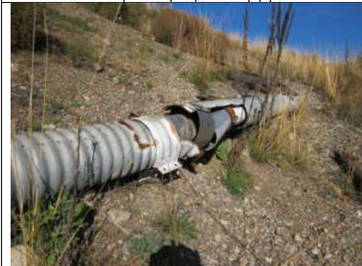
9 – Broken pipeline at junction between above and underground
