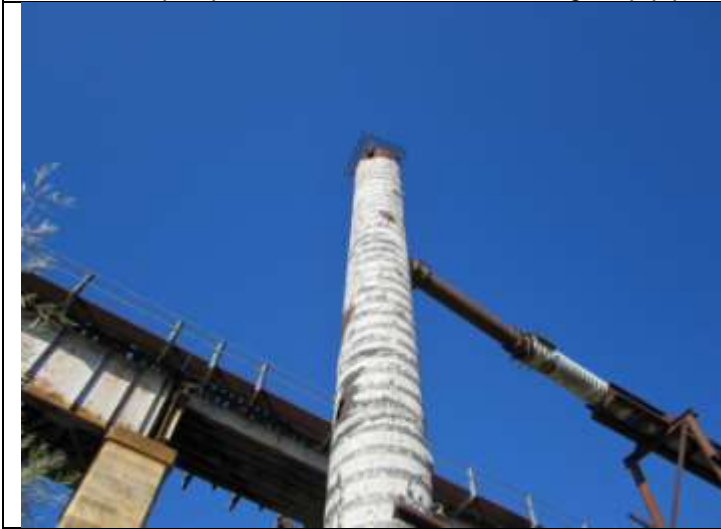
5 – Close-up – top of drop pipe
