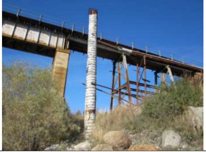
4 – Close-up of drop pipe
