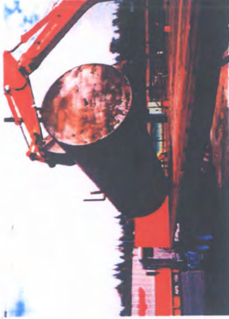
UST contents inerted with CO2 and transported to the PSC Tacoma Facility
