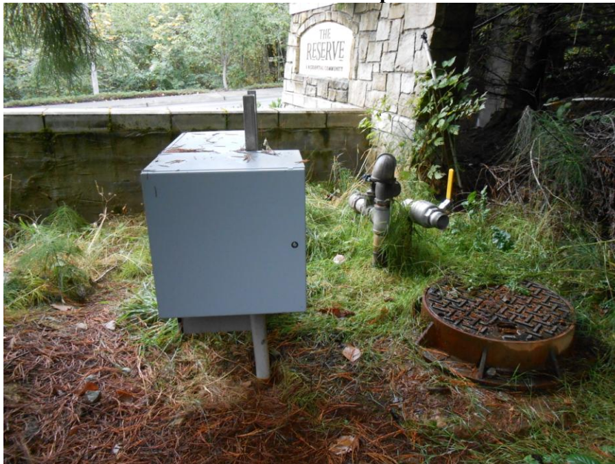
Photo 6: Leachate Pump Station
