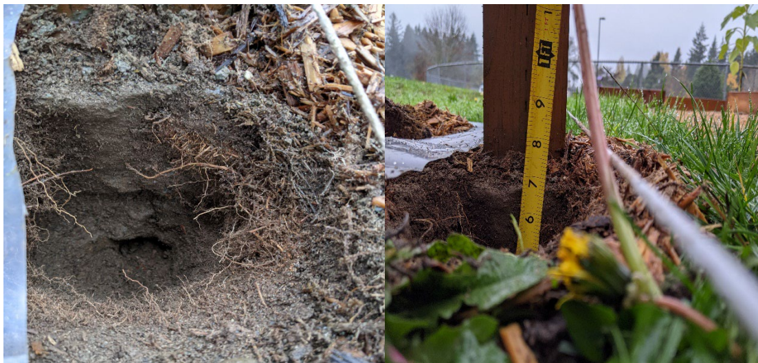
Photograph 2. Depth of post holes and concrete.
