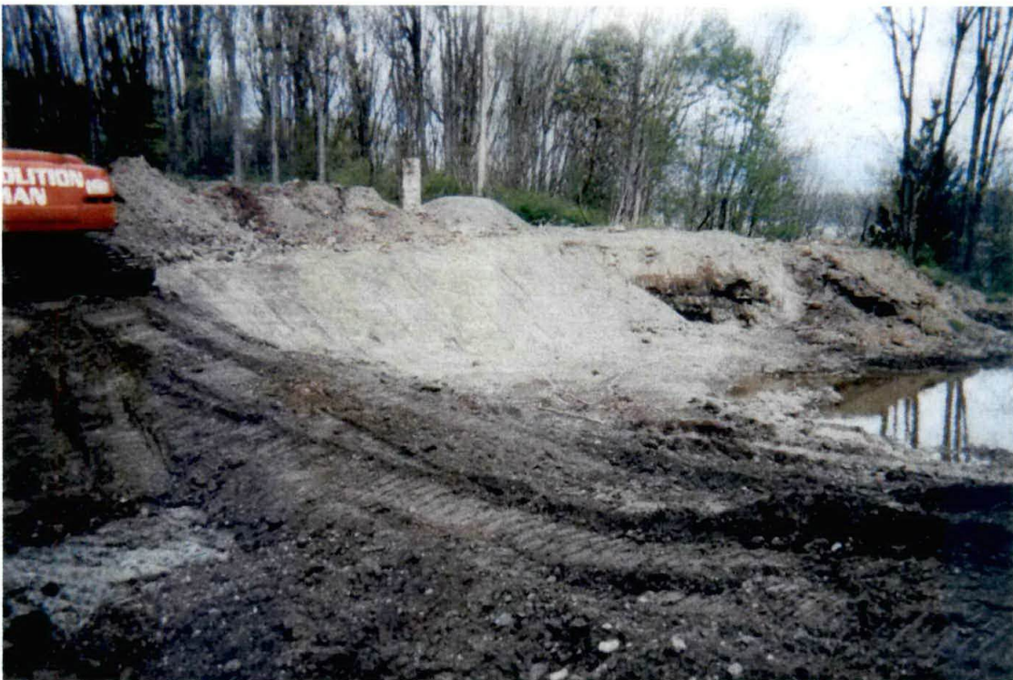
Photograph #14 – View after battery casing material was excavated and the overburden was used to reduce erosion from the excavation area.
