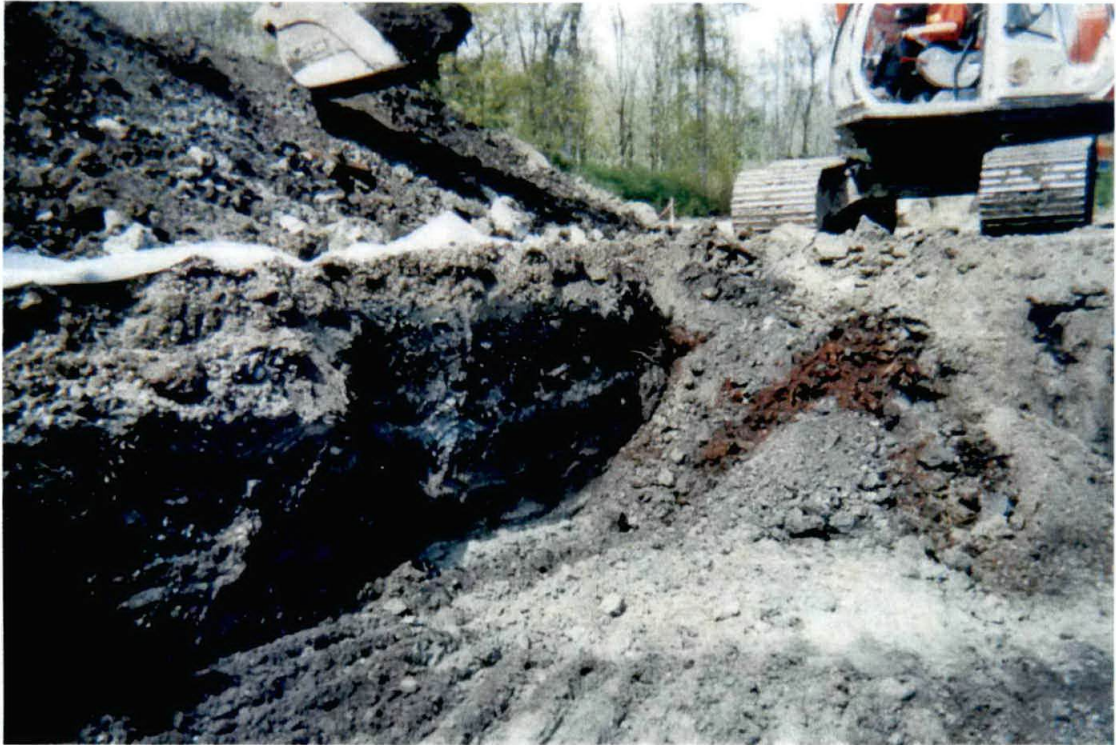
Photograph #13 – Final excavated area, gray material on left (west) side of the pile is clay soil.
