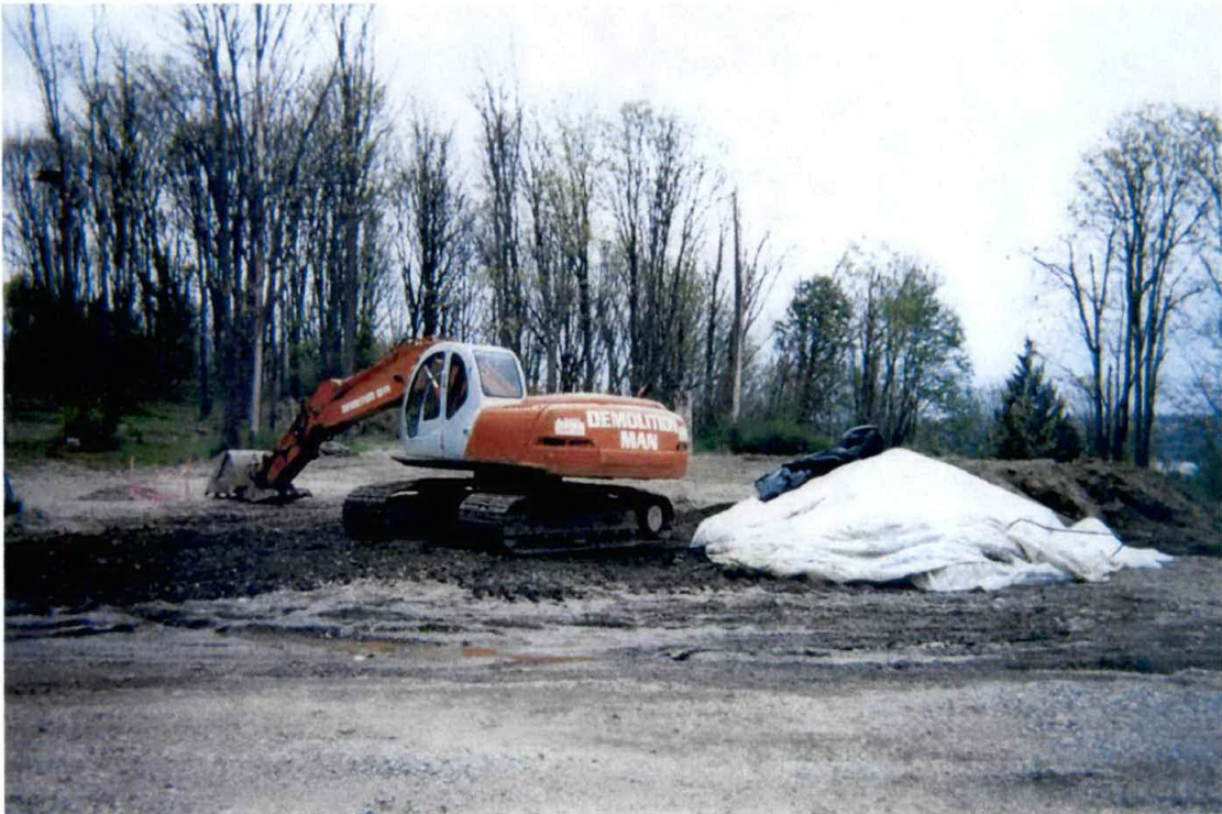
Photograph #20 – Small pile of CKD material left to be removed on Friday April 14, 2006.
