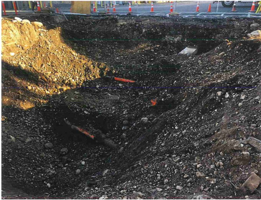
Photograph 13. Highbay area excavation of PAH contaminated soil. SES marked daylighted utilities with orange paint.
