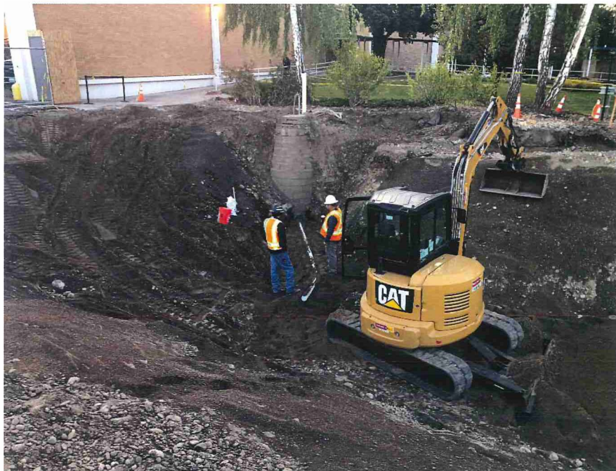
Photograph 16. SES plumbs liner drain pipe into stormwater system manhole found on the east side of the highbay area, looking Northeast.
