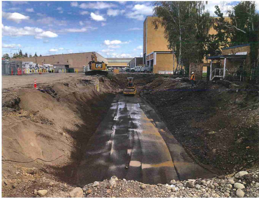
Photograph 15. SES begins backfill and compaction of select fill in base of excavation, looking North.
