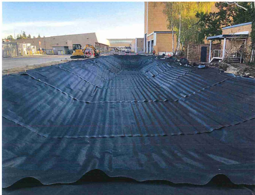
Photograph 18. ACF West places 40-mil thick LLDPE geosynthetic liner over fabric, looking North.
