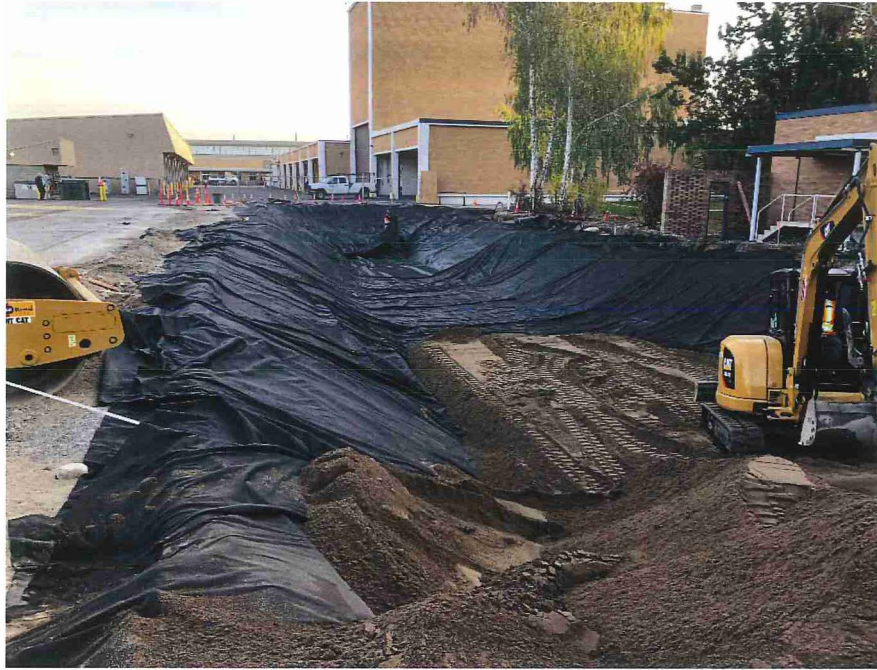
Photograph 21. SES begins placing geotextile fabric and bedding sand over the geosynthetic liner, looking North.
