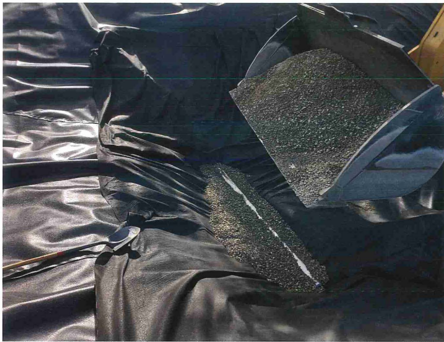
Photograph 23. SES constructs the liner drain with 3/4-inch drain rock around drain pipe and wrapped in geotextile fabric, looking East.
