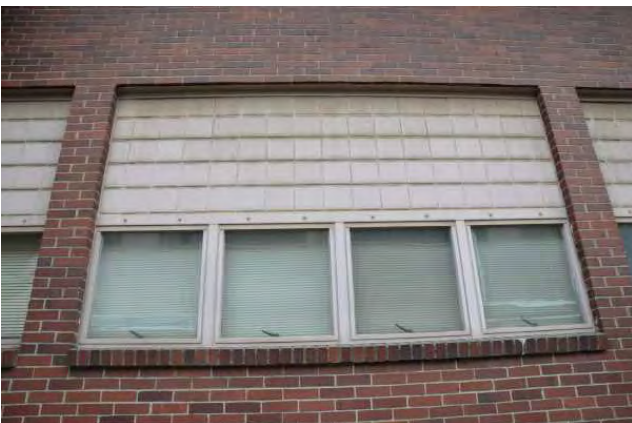
Window opening on south side of building, showing extent of infill, view to the north.
