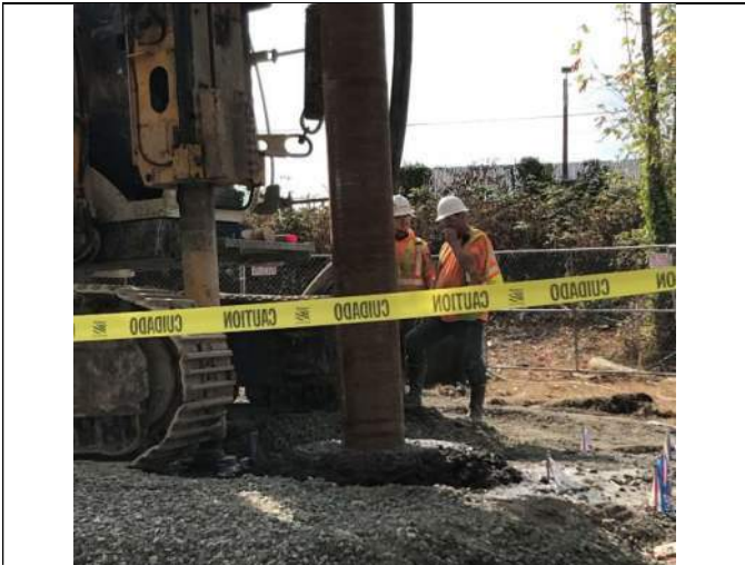
Picture Date: Thursday 09/23/2021 Picture Taken By: Haley Provinsal Picture Location: Puyallup, Washington Project Name: USG Puyallup Site Project Description: Mixing ISS-1
