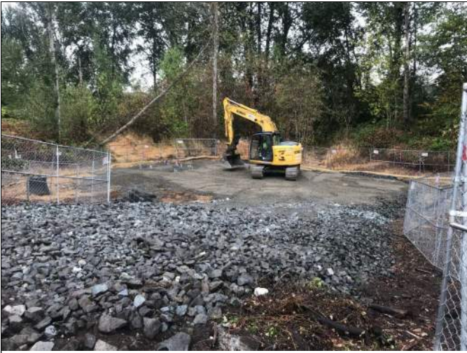
Picture Date: Friday 09/17/2021 Picture Taken By: Haley Provinsal Picture Location: Puyallup, Washington Project Name: USG Puyallup ISS Pilot Study Project Description: Placement of rock ballast and rock/gravel pad
