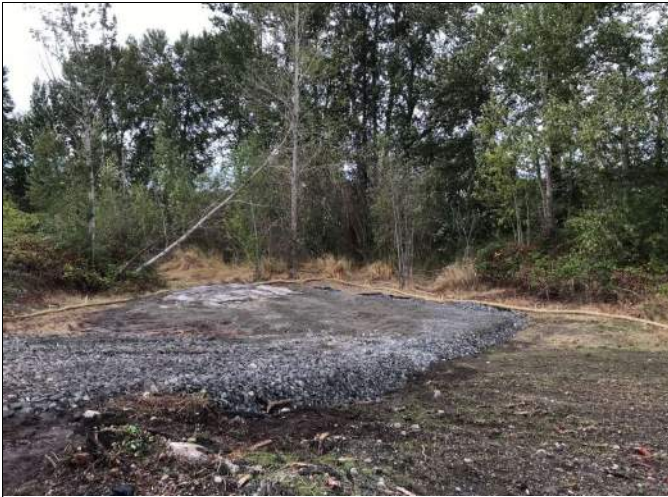
Picture Date: Monday 09/27/2021 Picture Taken By: Haley Provinsal Picture Location: Puyallup, Washington Project Name: USG Puyallup ISS Pilot Study Project Description: Status of site following field work
