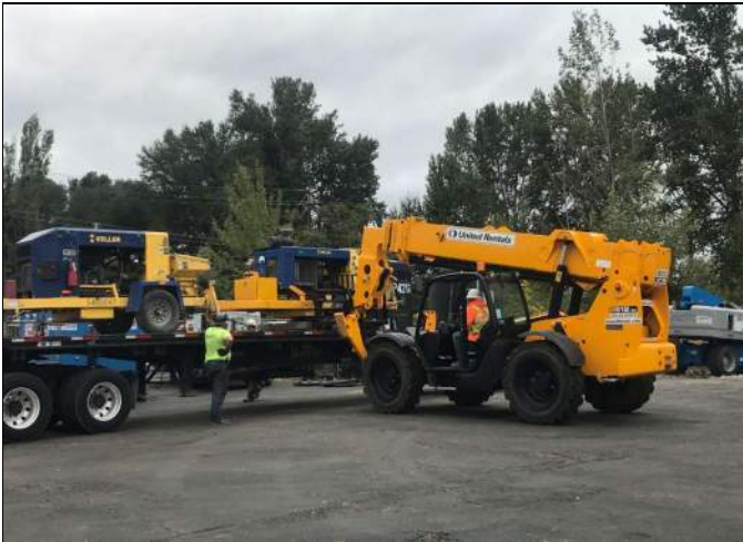
Picture Date: Wednesday 09/22/2021 Picture Taken By: Haley Provinsal Picture Location: Puyallup, Washington Project Name: USG Puyallup ISS Pilot Study Project Description: Unloading a pump off the trailer
