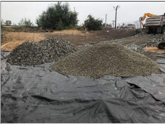
Picture Date: Friday 09/17/2021 Picture Taken By: Haley Provinsal Picture Location: Puyallup, Washington Project Name: USG Puyallup ISS Pilot Study Project Description: Gravel and rock delivery
