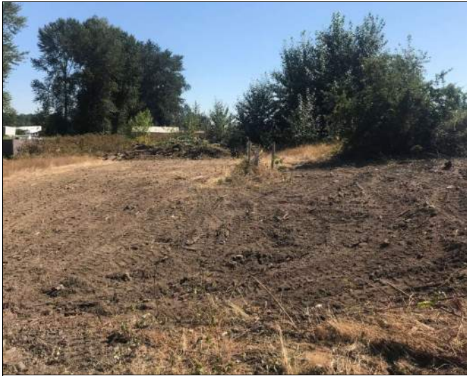
Picture Date: Saturday 08/28/2021 Picture Taken By: Haley Provinsal Picture Location: Puyallup, Washington Project Name: USG Puyallup ISS Pilot Study Project Description: Land clearing
