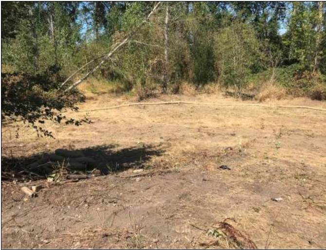
Picture Date: Saturday 08/28/2021 Picture Taken By: Haley Provinsal Picture Location: Puyallup, Washington Project Name: USG Puyallup ISS Pilot Study Project Description: Land clearing with installation of straw waddles
