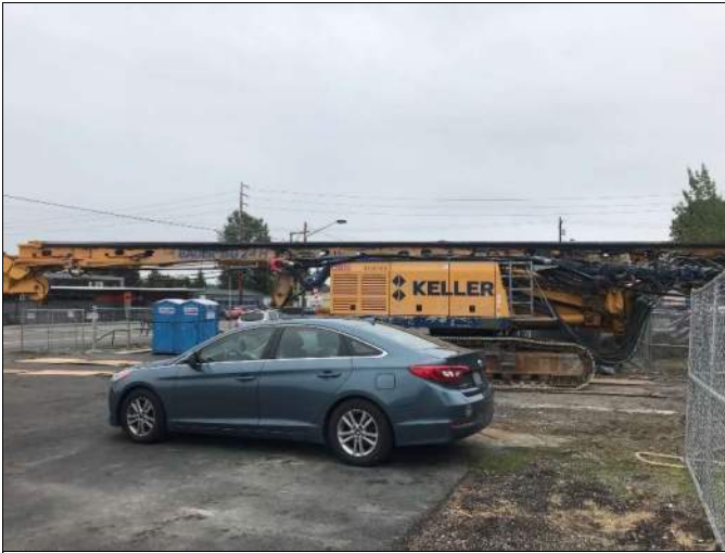
Picture Date: Wednesday 09/29/2021 Picture Taken By: Haley Provinsal Picture Location: Puyallup, Washington Project Name: USG Puyallup Site Project Description: Equipment remaining on site - Drill rig
