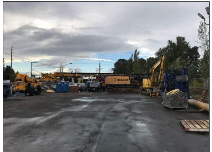
Picture Date: Monday 09/27/2021 Picture Taken By: Haley Provinsal Picture Location: Puyallup, Washington Project Name: USG Puyallup ISS Pilot Study Project Description: Drill rig staged for transport
