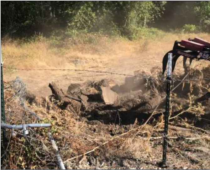
Picture Date: Saturday 08/28/2021 Picture Taken By: Haley Provinsal Picture Location: Puyallup, Washington Project Name: USG Puyallup ISS Pilot Study Project Description: Debris found near asphalt and fence (contained large blocks of cement, bricks, and trash)
