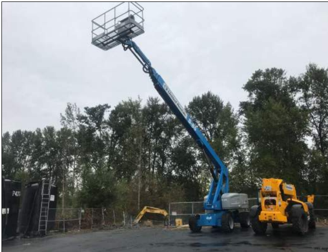
Picture Date: Friday 09/17/2021 Picture Taken By: Haley Provinsal Picture Location: Puyallup, Washington Project Name: USG Puyallup ISS Pilot Study Project Description: Equipment on site
