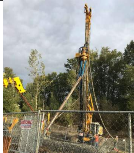
Picture Date: Monday 09/27/2021 Picture Taken By: Haley Provinsal Picture Location: Puyallup, Washington Project Name: USG Puyallup Site Project Description: Removing pipe from drill rig for transport
