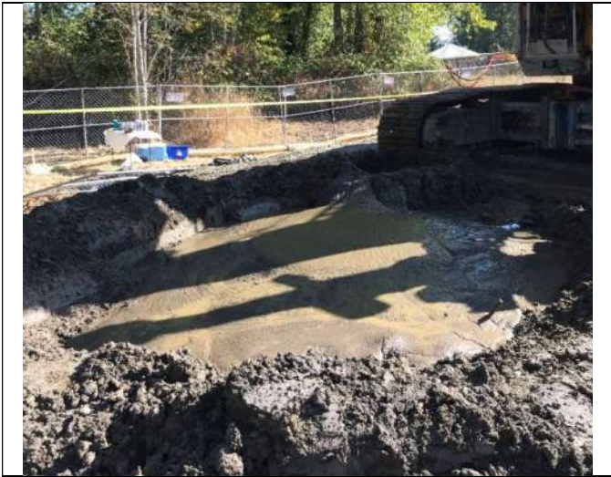
Picture Date: Thursday 09/23/2021 Picture Taken By: Haley Provinsal Picture Location: Puyallup, Washington Project Name: USG Puyallup Site Project Description: Spoils pile following ISS-2
