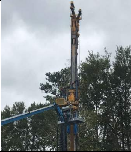
Picture Date: Wednesday 09/22/2021 Picture Taken By: Haley Provinsal Picture Location: Puyallup, Washington Project Name: USG Puyallup ISS Pilot Study Project Description: Working on the connections on the drill rig
