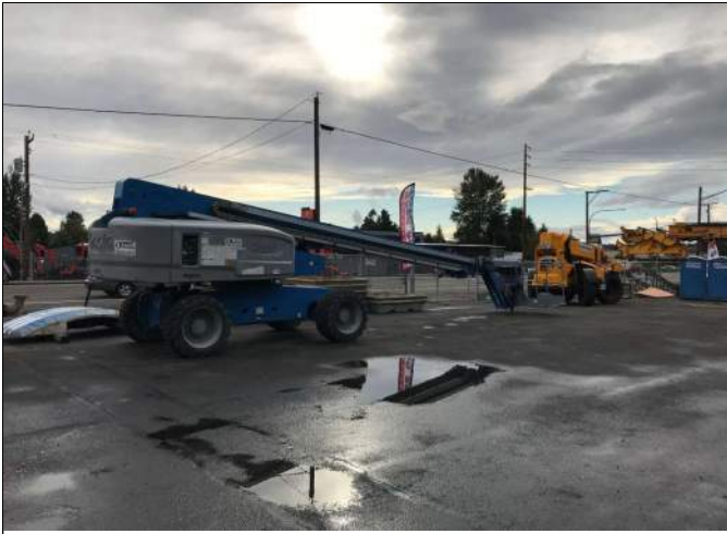
Picture Date: Monday 09/27/2021 Picture Taken By: Haley Provinsal Picture Location: Puyallup, Washington Project Name: USG Puyallup Site Project Description: Equipment remaining on site
