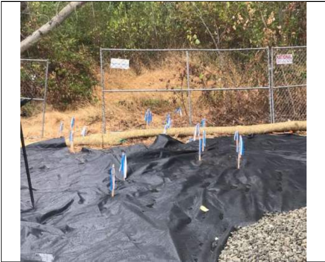
Picture Date: Friday 09/17/2021 Picture Taken By: Haley Provinsal Picture Location: Puyallup, Washington Project Name: USG Puyallup ISS Pilot Study Project Description: Surveyed locations for 5 columns (includes 5 column bundle, 2 column bundle, and offsets for each column)
