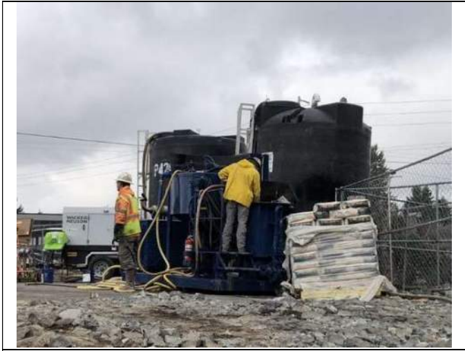
Picture Date: Thursday 09/23/2021 Picture Taken By: Matt Schultz Picture Location: Puyallup, Washington Project Name: USG Puyallup ISS Pilot Study Project Description: Mixing bentonite mixture
