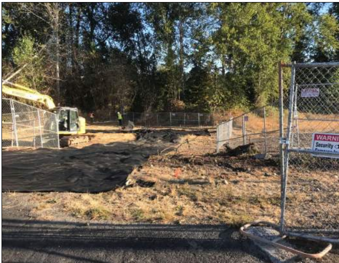
Picture Date: Thursday 09/16/2021 Picture Taken By: Haley Provinsal Picture Location: Puyallup, Washington Project Name: USG Puyallup ISS Pilot Study Project Description: Laying down liner in preparation of gravel and rock delivery for rock ballast and working pad
