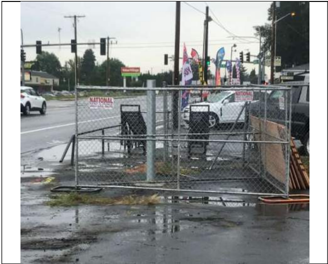
Picture Date: Thursday 09/17/2021 Picture Taken By: Haley Provinsal Picture Location: Puyallup, Washington Project Name: USG Puyallup ISS Pilot Study Project Description: New post for new gate on western side of River Road entrance
