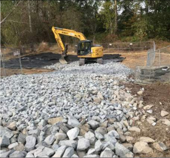
Picture Date: Thursday 09/16/2021 Picture Taken By: Haley Provinsal Picture Location: Puyallup, Washington Project Name: USG Puyallup ISS Pilot Study Project Description: Placement of rock ballast
