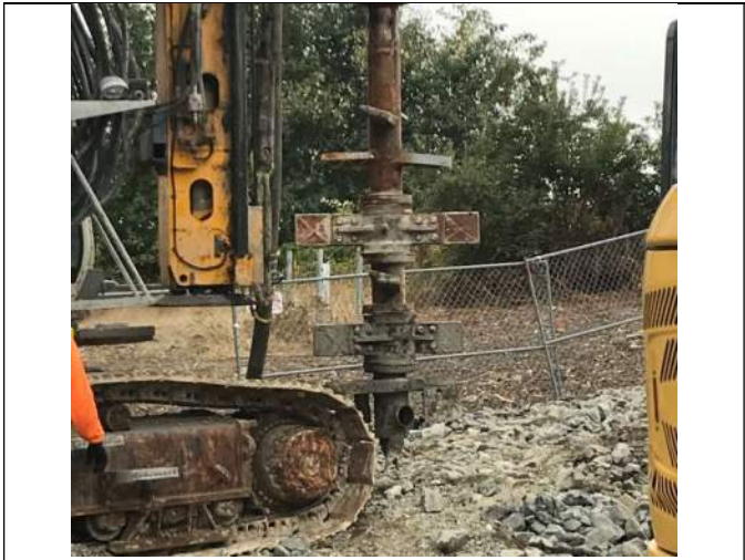
Picture Date: Thursday 09/23/2021 Picture Taken By: Haley Provinsal Picture Location: Puyallup, Washington Project Name: USG Puyallup Site Project Description: Drill head and port
