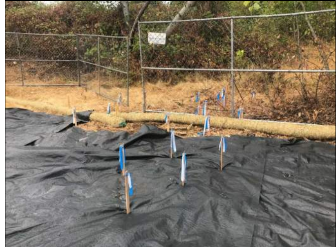
Picture Date: Friday 09/17/2021 Picture Taken By: Haley Provinsal Picture Location: Puyallup, Washington Project Name: USG Puyallup ISS Pilot Study Project Description: Surveyed locations for 5 columns (includes 5 column bundle and offsets for each column)
