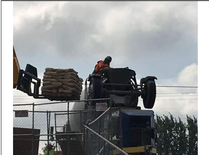
Picture Date: Thursday 09/23/2021 Picture Taken By: Haley Provinsal Picture Location: Puyallup, Washington Project Name: USG Puyallup ISS Pilot Study Project Description: Mixing Ferrous Sulfate Heptahydrate into the cement truck
