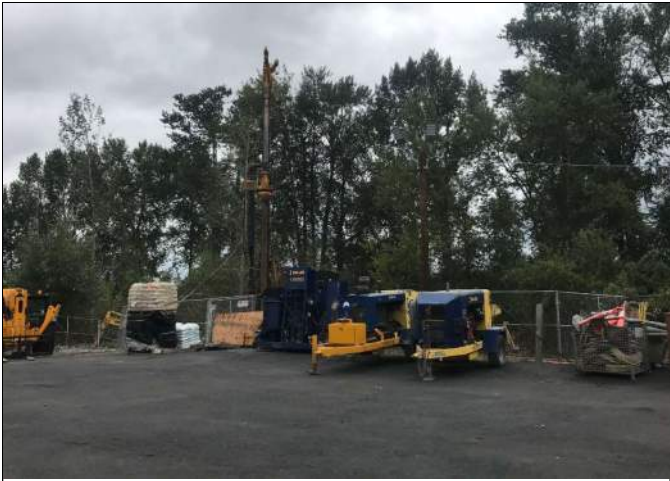
Picture Date: Wednesday 09/22/2021 Picture Taken By: Haley Provinsal Picture Location: Puyallup, Washington Project Name: USG Puyallup Site Project Description: Placement of equipment and materials at the end of the day
