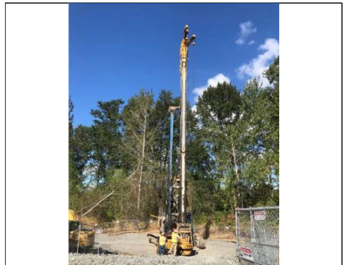
Picture Date: Monday 09/20/2021 Picture Taken By: Haley Provinsal Picture Location: Puyallup, Washington Project Name: USG Puyallup ISS Pilot Study Project Description: Setting up the drill rig
