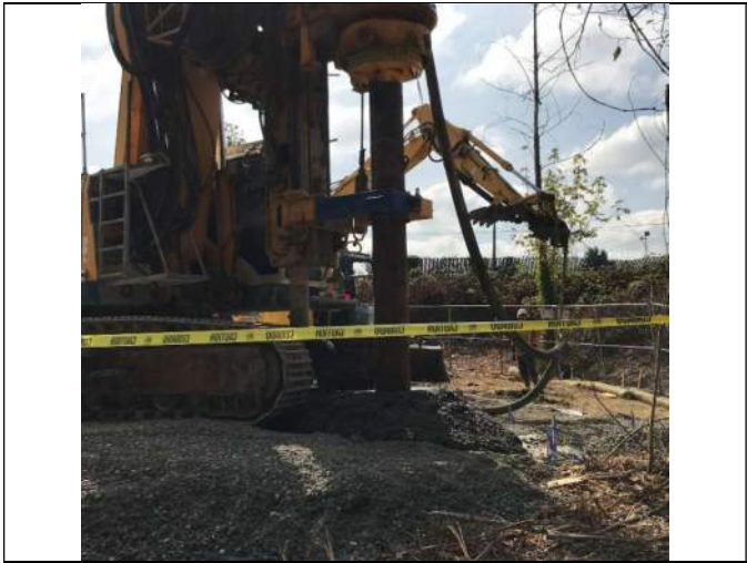
Picture Date: Thursday 09/23/2021 Picture Taken By: Haley Provinsal Picture Location: Puyallup, Washington Project Name: USG Puyallup Site Project Description: Final spoils for ISS-1
