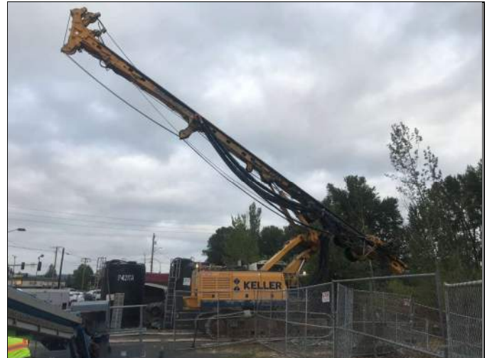
Picture Date: Monday 09/20/2021 Picture Taken By: Haley Provinsal Picture Location: Puyallup, Washington Project Name: USG Puyallup ISS Pilot Study Project Description: ISS Drill Rig arrived on site
