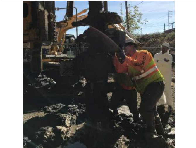
Picture Date: Thursday 09/23/2021 Picture Taken By: Haley Provinsal Picture Location: Puyallup, Washington Project Name: USG Puyallup ISS Pilot Study Project Description: Mounting the sampling box onto the rig
