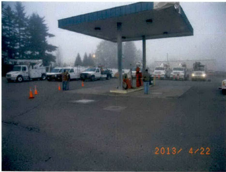
Fuel dispensers and transition sumps under canopy, monitoring well in foreground
