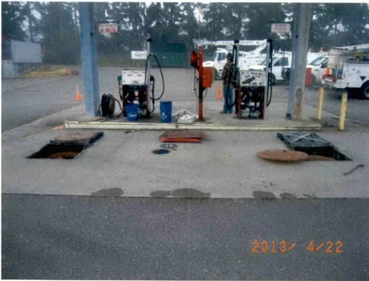
Transition sumps opened
