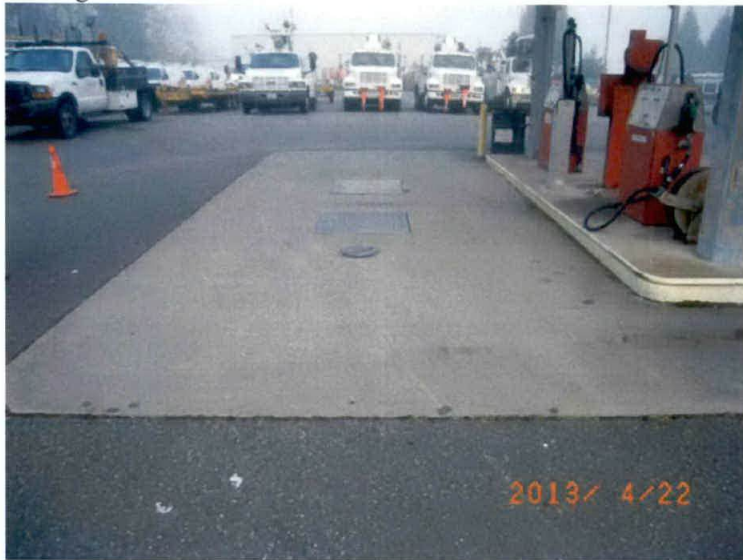
Transition sumps on either side of dispenser island
