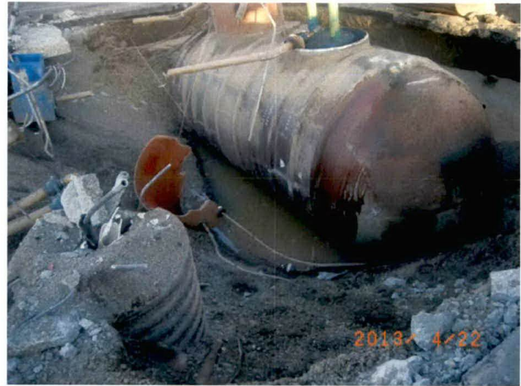
Ground water was encountered at approx. 8 feet depth; deadman strap failure caused the tank to rise buoyantly in the excavation.
