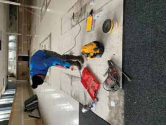
Using a Hilti roto-hammer to drill a 5/8-inch hole through the slab at SUB01 – NE building corner looking south.
