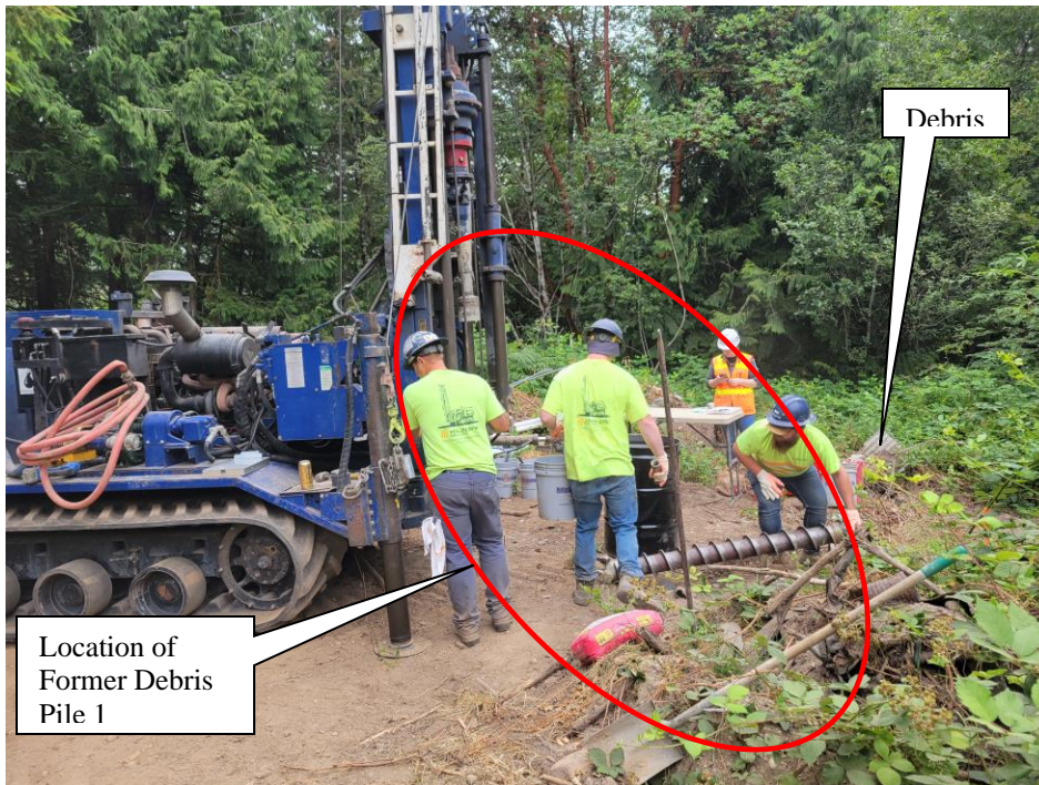
Photo 2: 7-13-21 Monitoring Well Installation – View showing the location of Monitoring Well 4 in the location of former Debris Pile 1.
