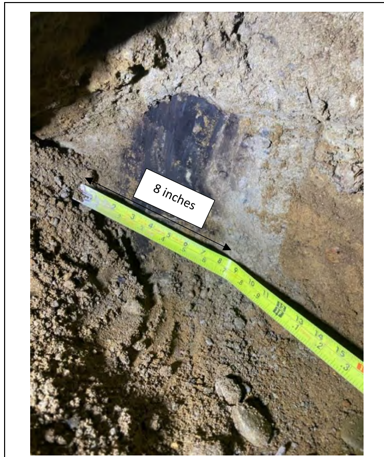
Plate 2. Observed Pile 2 condition. Timber pile is approximately 8 inches in diameter. Did not observe signs of decay on the existing timber pile. (12/31/2020)
