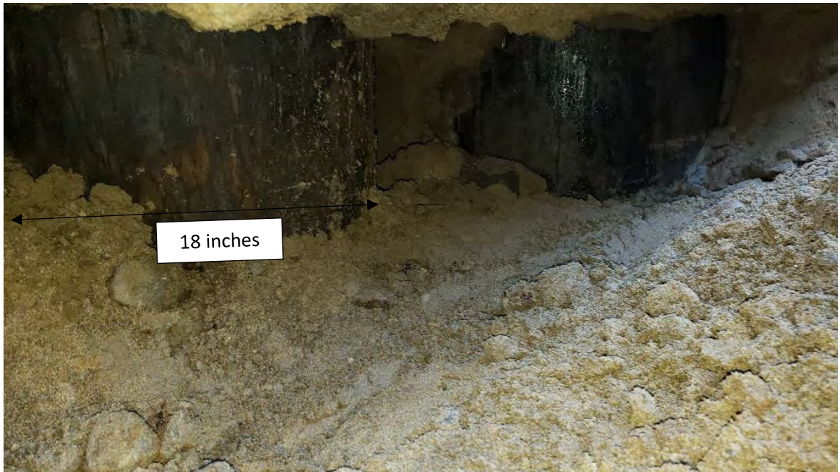
Plate 3. Piles observed in northwest corner of north loading dock by Urban Environmental Partners (UEP). Timber piles are approximately 18 inches in diameter. Photo provided by UEP. Do not observe signs of decay on the existing timber piles.
