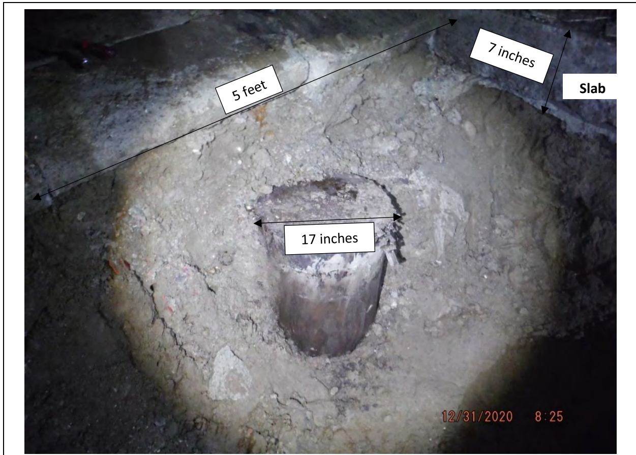
Plate 1. Excavation and pile condition at Pile 109. The existing concrete slab was poured directly on the existing timber pile. Top of timber pile is approximately 17 inches in diameter. Did not observe signs of decay on the existing timber pile. (12/31/2020)
