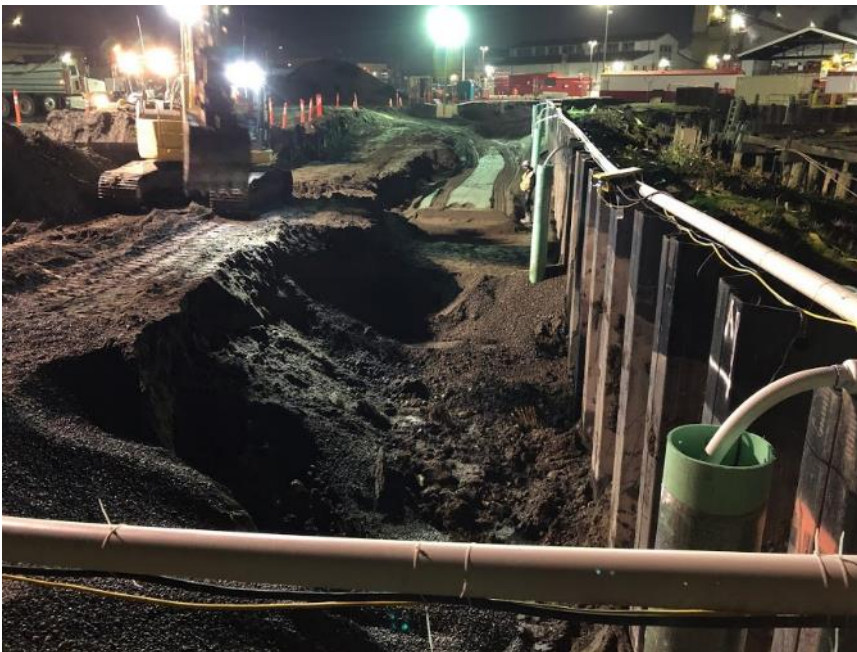
Photograph 12. 01/13/21: South facing view of excavation from North of cell A-1. Backfill through cell C-1 and open excavation in cells A-1, B-1.
