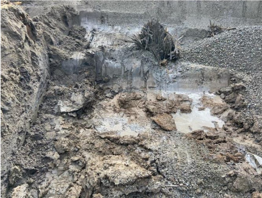
Photograph 15. 01/15/2021: Overexcavation to elevation 4.5 ft in cell K-1. Photo documents Estuarine Unit. Sheen and odor from creosote pile observed.
