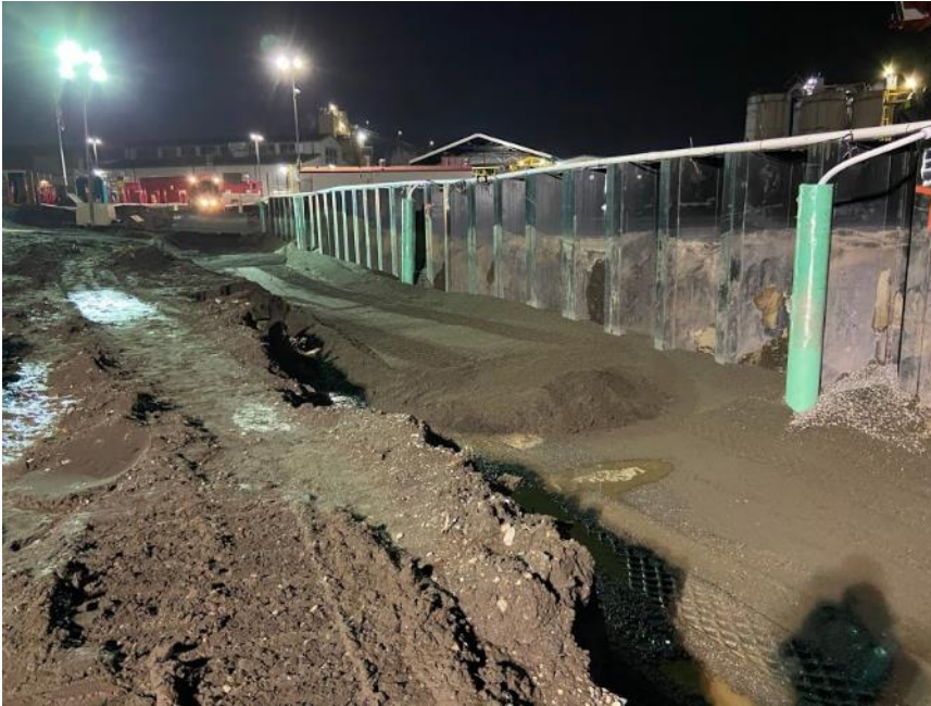
Photograph 11. 01/12/21: South facing view of completed excavation and partial backfill through cell C-1.
