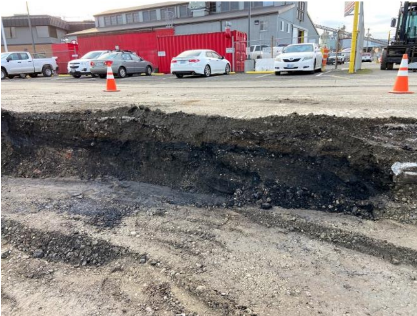
Photograph 19. South property boundary in cell M-3. Dark gray soil is coal beneath asphalt, not sand blast grit.
