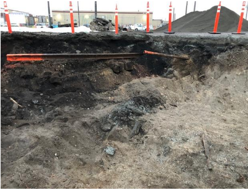
Photograph 3. 12/29/2020: East facing view of railroad tie and pipe in Cell K-2. Pure sandblast grit observed in sidewall at IAWP estimated extents.
