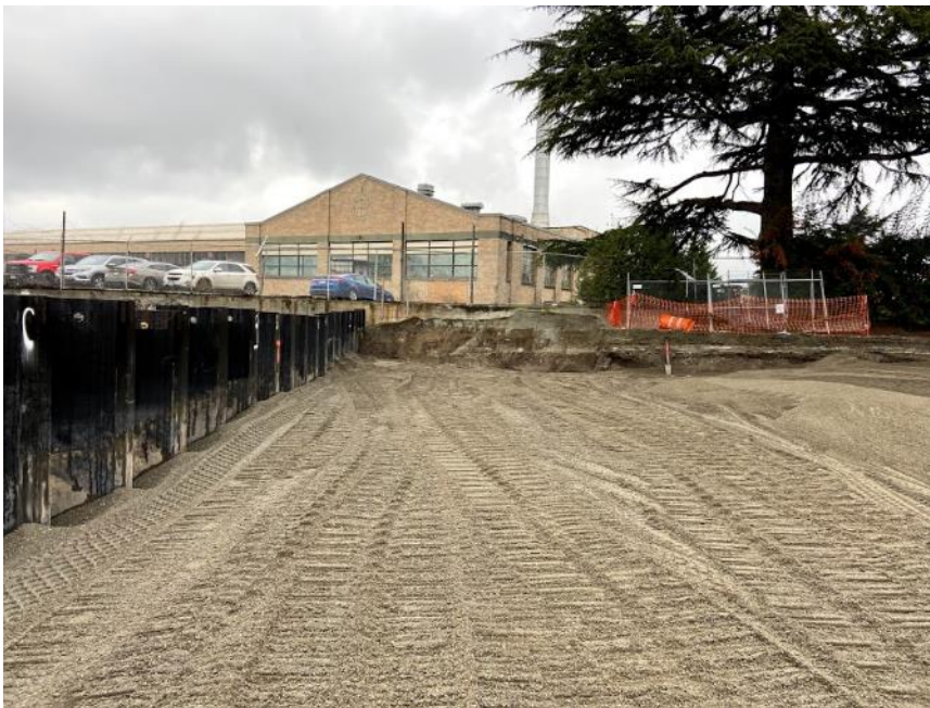
Photograph 18. 01/21/2021. North facing view of northern excavation limit. Cell A-1 is sloped away from retaining wall on property line down to elevation 12 ft.
