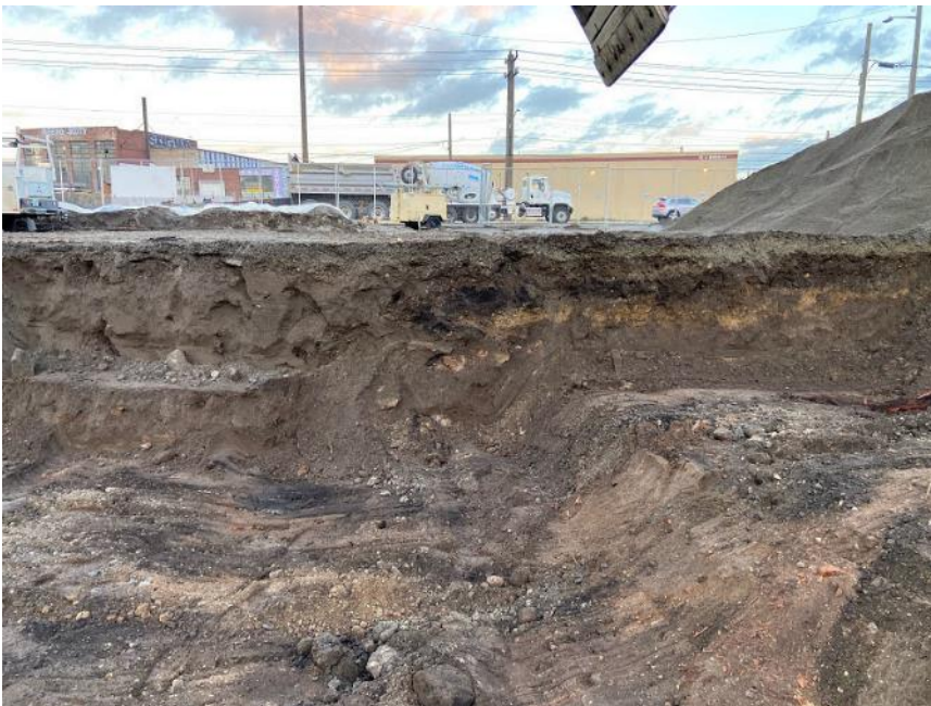
Photograph 16. 01/15/21: Seam of sandblast grit observed in eastern sidewall at K-3, elevation 15 ft, removed in overexcavation.
