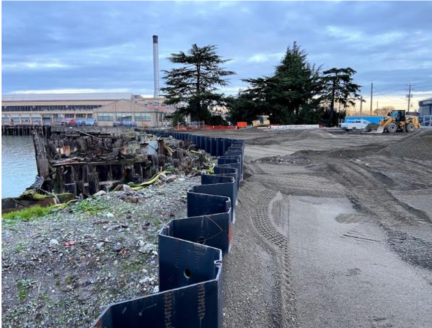
Photograph 21. 01/22/2021 North facing view from south end of site of backfilled excavation area.
