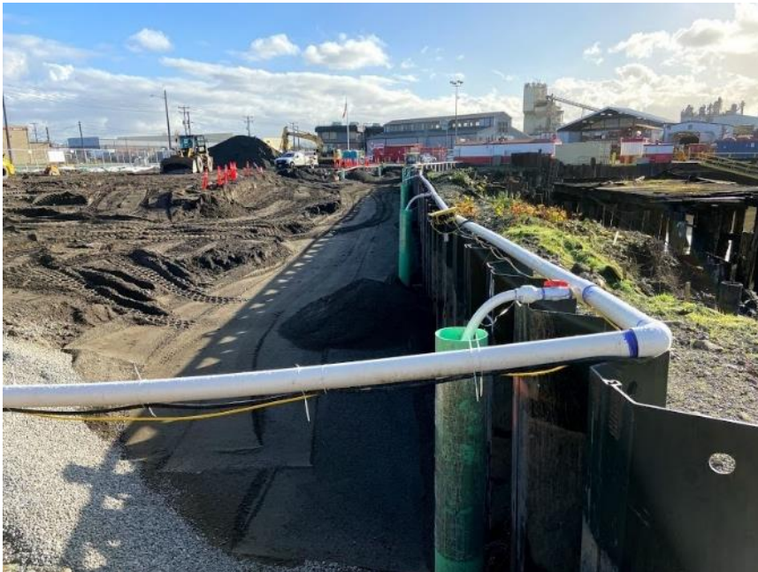
Photograph 14. 01/15/21: South facing view of excavation from Northern limit. Excavation has been backfilled to approximately elevation 10 ft.
