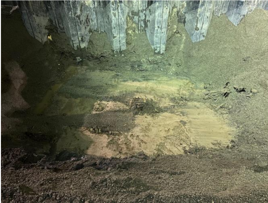
Photograph 13. 01/13/21: Over excavation in cell J-1 down to Estuarine Unit. Backfill removed and approximately 0.5 ft of Estuarine Unit removed to obtain new bottom sample.
