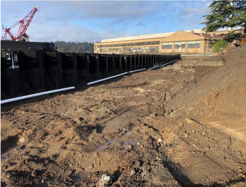
Photograph 5. 12/30/2020: Northwest facing view of excavation progress and dewatering header pipe from approximate location cell I-2.
