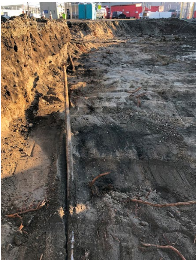
Photograph 2. 12/28/2020: Eastern excavation temporary cut wall excavated to elevation 12 feet (ft). Standing in Cell G-1 and facing south. Dark material in east cut slope is mixed fill, removed in overexcavation.
