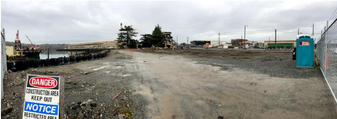
Photograph 1. 12/28/2020: North facing view of site from southwest corner of site, prior to excavation.
