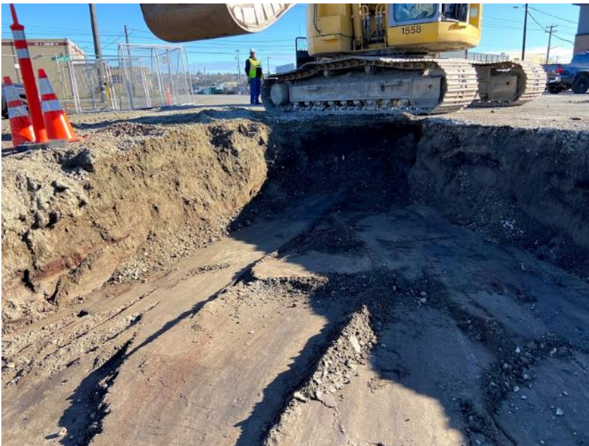
Photograph 20. SE facing view – reaching edge of excavation along building footprint and property line in cell N-5.
