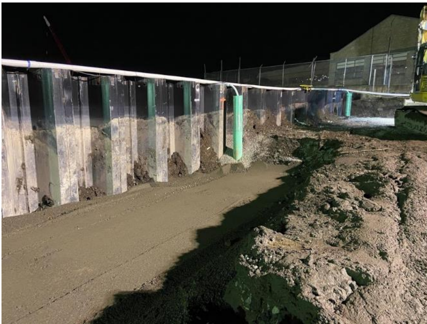
Photograph 10. 01/12/21: Northwest facing view of completed excavation and partial backfill through cell C-1.
