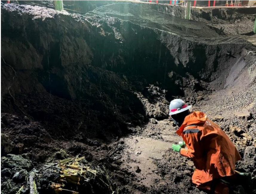
Photograph 9. 01/11/2021: Excavation extends bottom sampling in cell J-1, at elevation 4.5 ft in Estuarine Unit.
