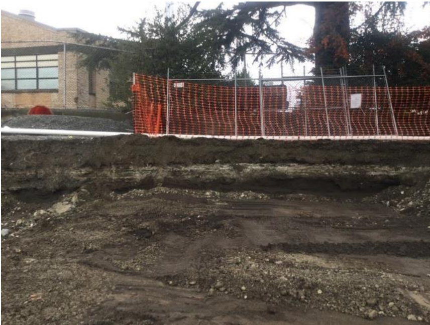
Photograph 6. 12/31/2020: Northern sidewall extended past planned excavation boundary approximately 5 to 8 ft further north.
