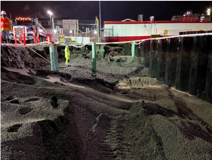
Photograph 8. 01/11/2021: South facing view of first 40 ft of saturated excavation in cells L-1 and K-1, backfilled with Type 26.
