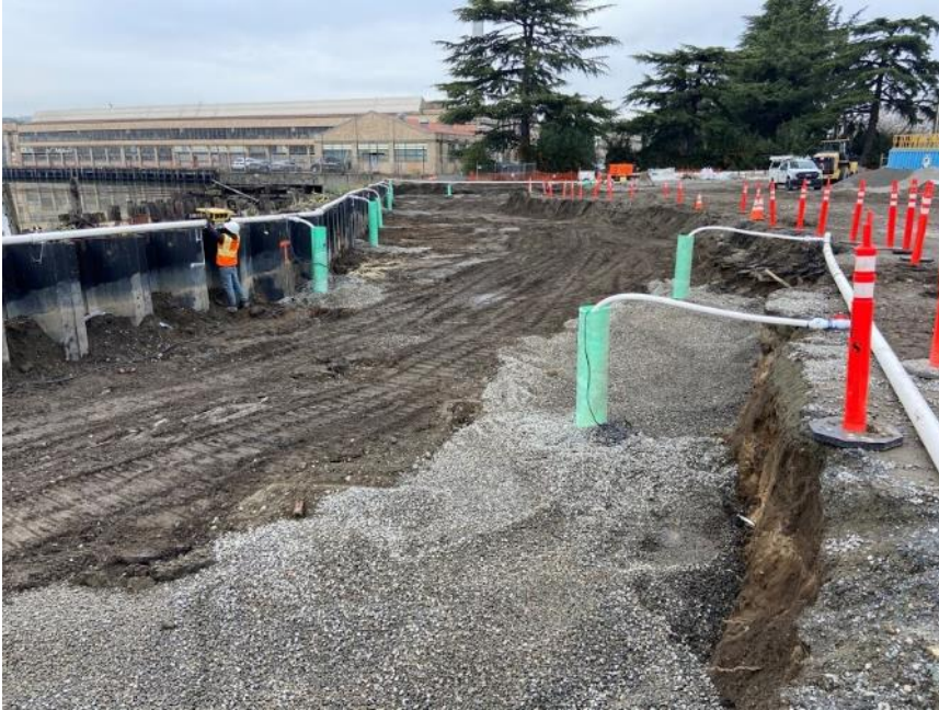
Photograph 7. 01/07/2021: Northwest facing view of dewatering system installation. Sumps along shoring and in trenches on north and south ends of site, backfilled with gravel. Excavation currently at elevation 12 ft.
