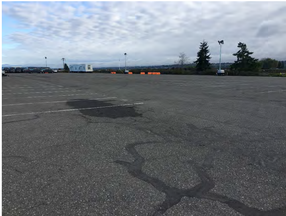
Photo 5. Facing northeast at the east portion of the asphalt cap. Repaired cracks are observed here.
