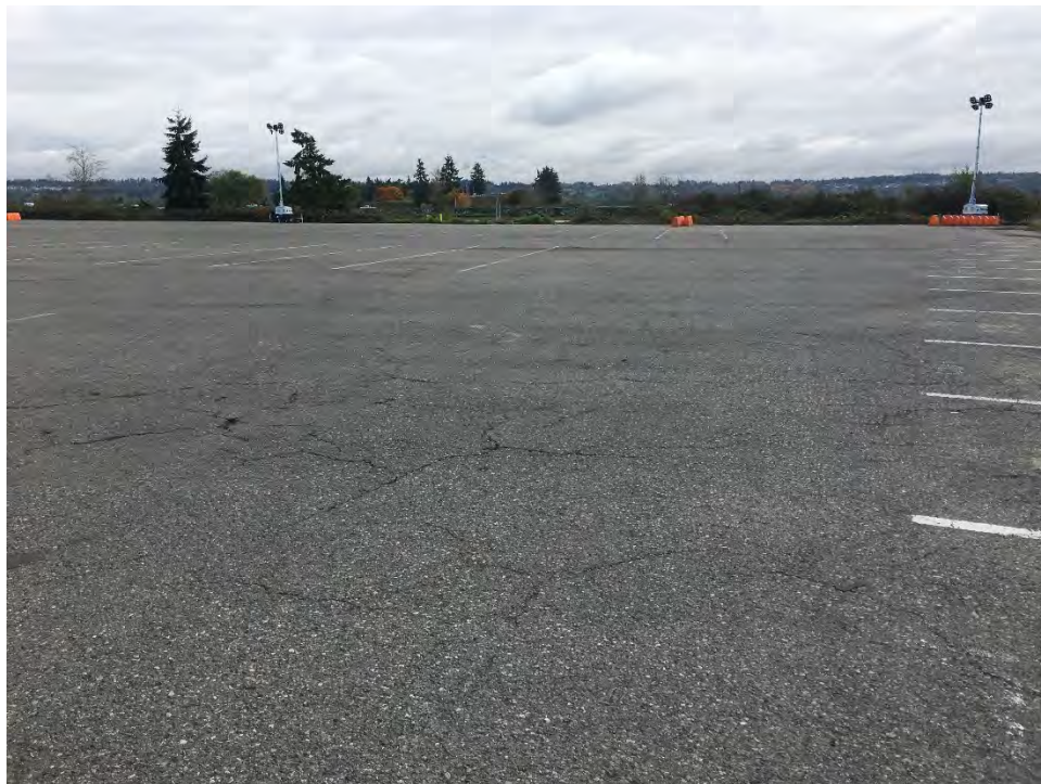
Photo 4. Observing minor cracking on the surface of the asphalt cap in the south portion of the asphalt cap.
