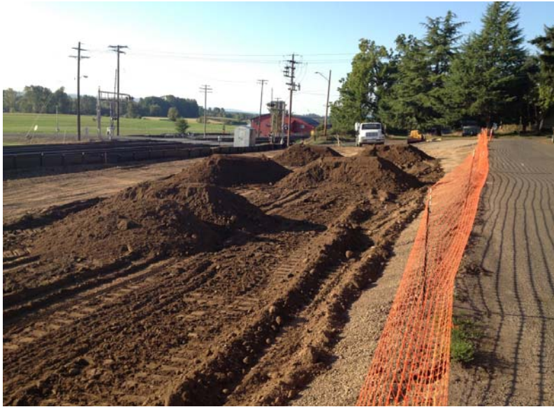
Photo 1: Material cut from high areas at the South Bench of the Railroad Avenue Site.
