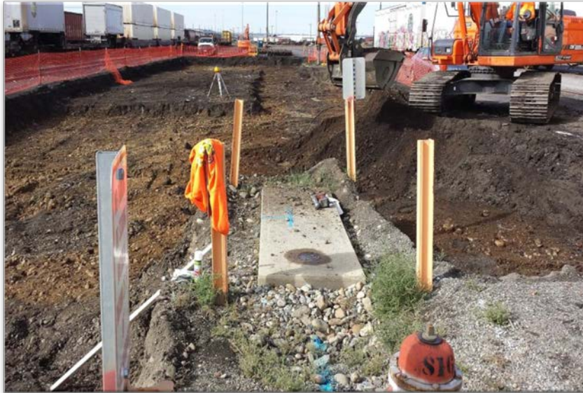
Photograph 5- Over excavation - Looking to west.
