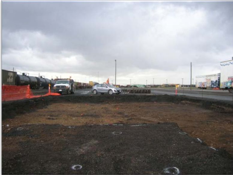
Photograph 3 – Over excavation - Looking to west.
