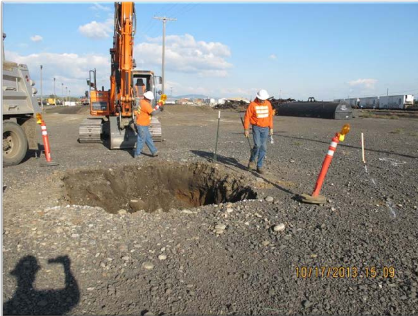
Photograph 5- Over excavation at location GTP-36B.
