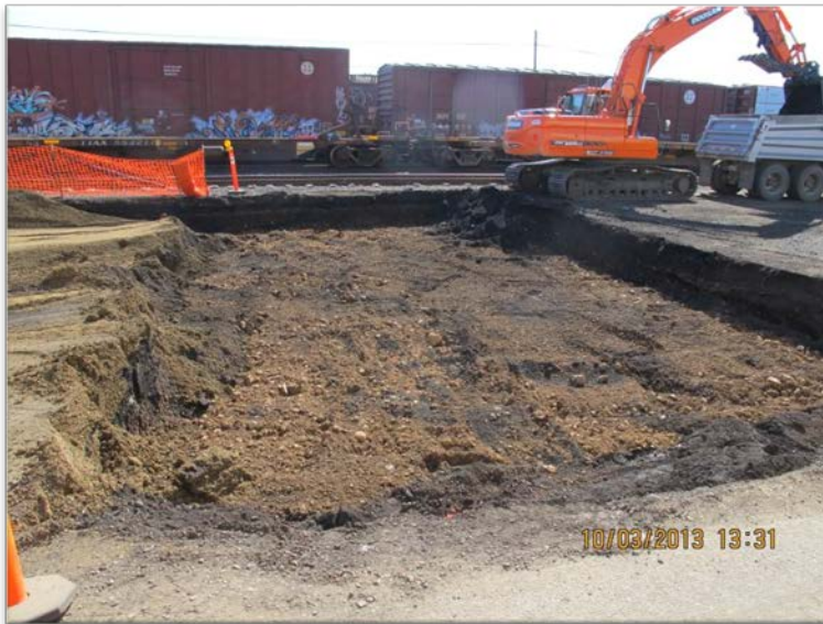
Photograph 7- Over excavation on west end - Looking to southwest.
