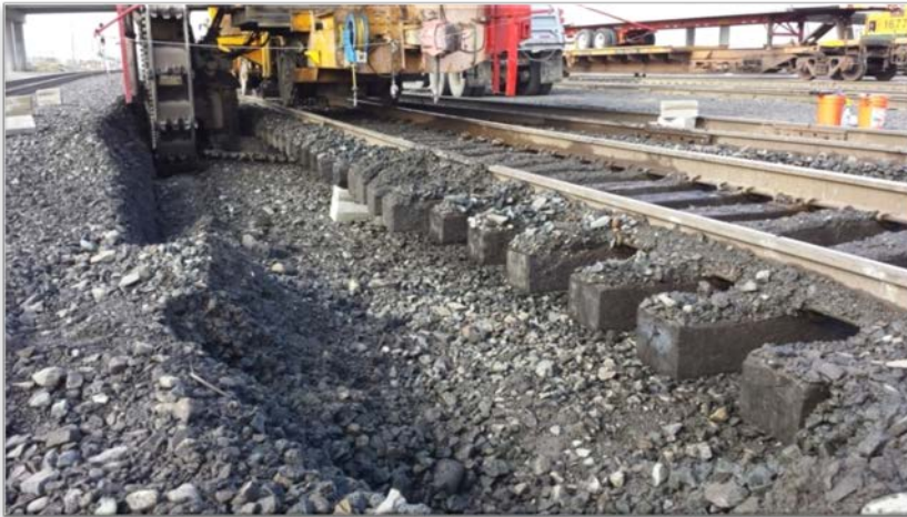
Photograph 5- Undercutter - Looking to west.
