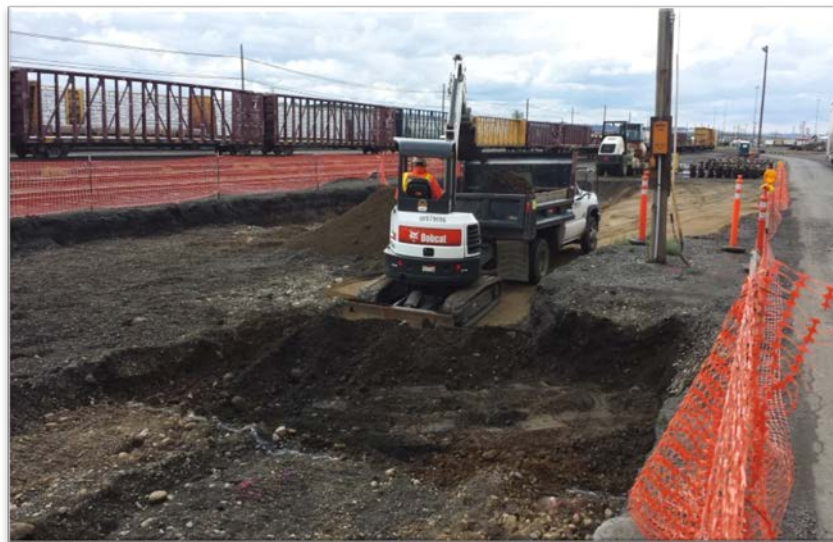
Photograph 6 – Over excavation at WFE-BS21-092513- Looking to southwest.
