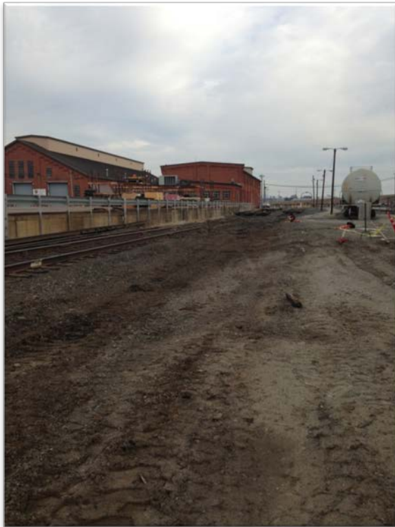
Photograph 1 - West excavation area prior to field activities. Track removal has occurred - Looking to northeast.
