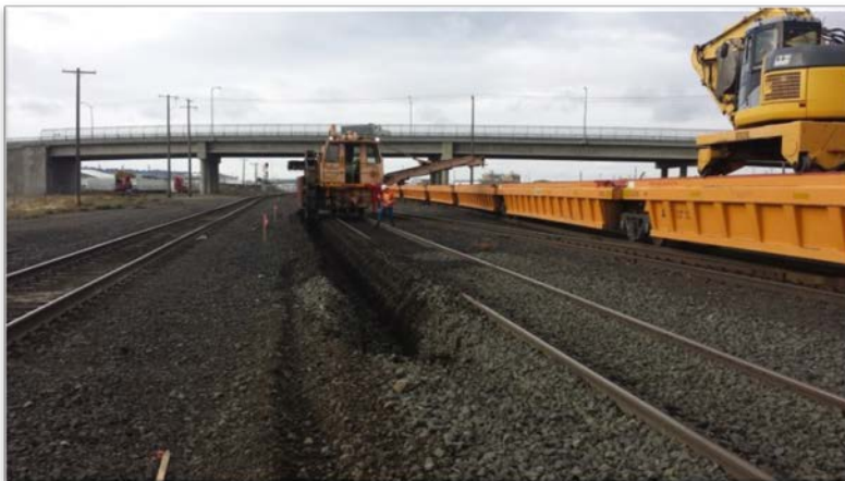
Photograph 2 – Undercutter - Looking to west.
