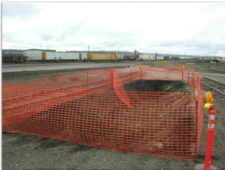
Photograph 5- Over excavation - Looking to southwest.
