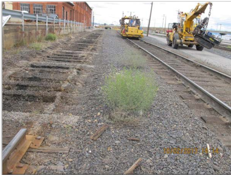
Photograph 1- East excavation area prior to field activities. Track removal has occurred – Looking to northeast.
