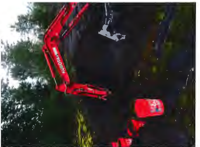
Excavator Digging a pit at EX8, 5-gallon sample buckets in the foreground
