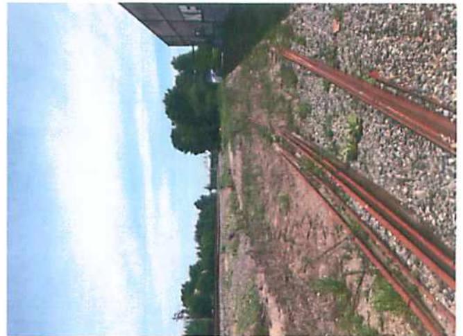
Rusted rails in the vicinity of presumed location of MW3
