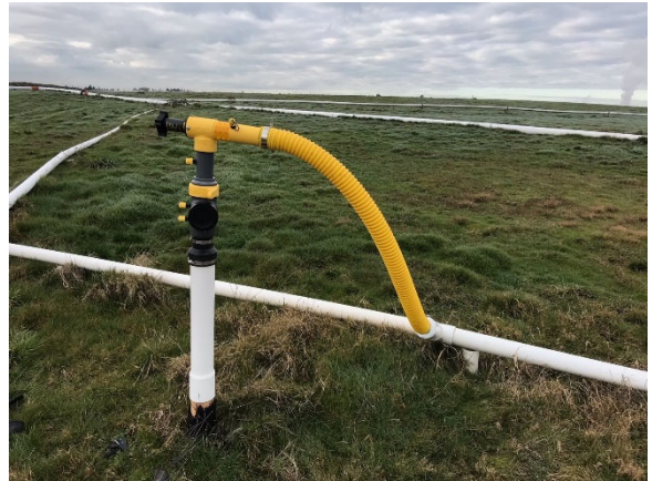
Installed Well Heads at E-41
