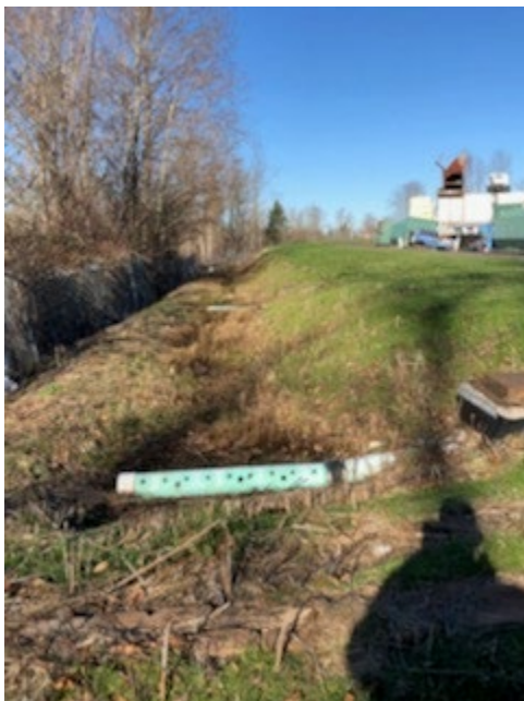
Photo 10: Stormwater discharge pipe extending west of closed ash landfill, view to north
