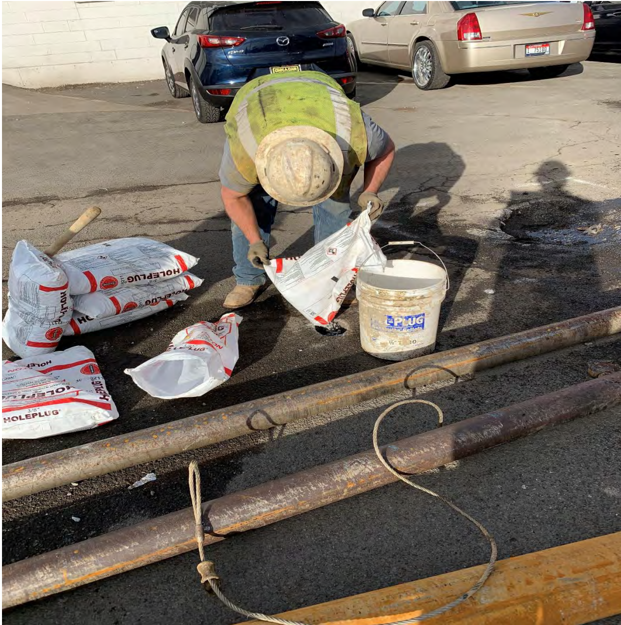
Photograph 12 – Driller’s helper pouring bentonite pellets into soil boring SB2, subsequent to soil sample collection.
