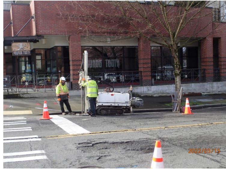
View south of drill rig set up at boring EB03 on the south parking strip of 87 th Avenue.
