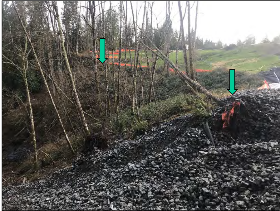
Photograph 1. View of the northeast slope. View is to the southeast. Quarry spalls in foreground are for stabilization of an access route for equipment down to the toe of the landfill. The orange silt fence in the middle-ground of the photo (between the green arrows) approximates the top of the northeast slope.
