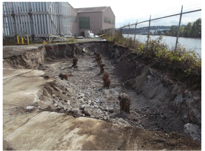
Photograph 4. Overview of the 6-foot-deep excavation for the SB4 Polygon and west sidewall. Photo viewing southeast.
