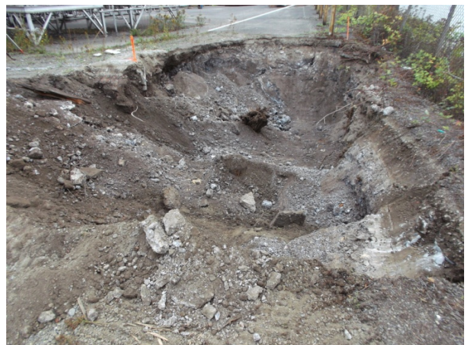
Photograph 6. South end of the 6-foot-deep excavation for the SB4 Polygon, in progress. Photo viewing southeast.
