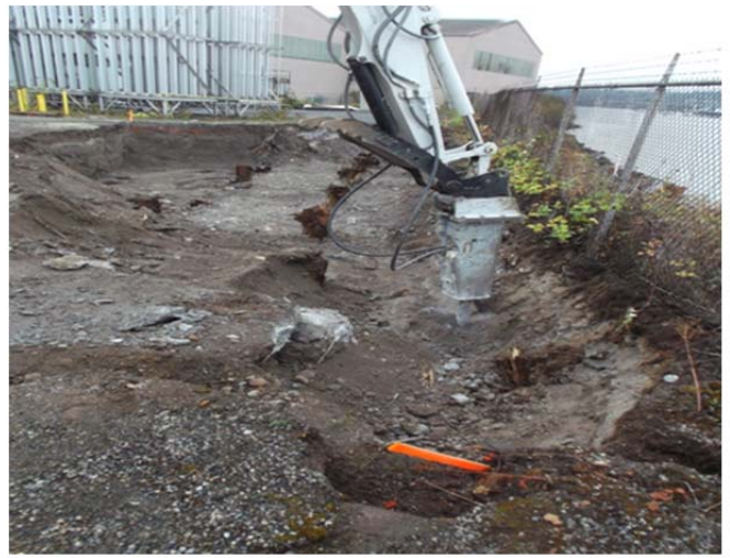
Photograph 8. Jackhammer required to excavate through cemented rubble in excavation for the SB4 Polygon. Photo viewing southeast.
