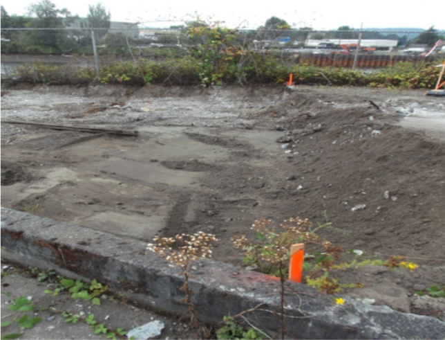
Photograph 9. North end of the 2-foot-deep excavation for the SB3 Polygon. Photo viewing west.
