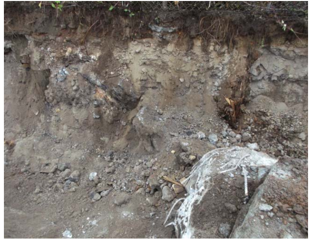
Photograph 10. View of bank material, concrete rubble, and piling exposed in west sidewall of the excavation for the SB4 Polygon.
