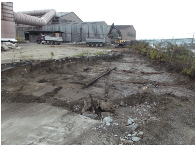
Photograph 3. Overview of the 2-foot-deep excavation for the SB3 Polygon. Photo viewing southeast.
