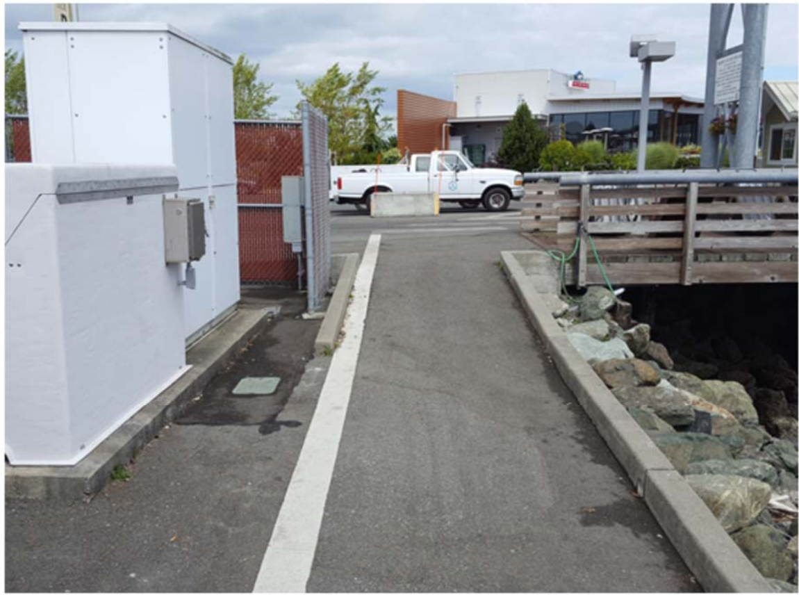
Photo A7: Protective asphalt barrier east of the utilities looking north (see Figure 1).
