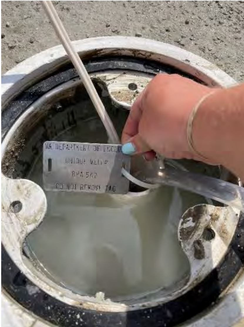
Photo 5. Monitoring wells fitted with Department of Ecology well tags (MW-7D shown here).
