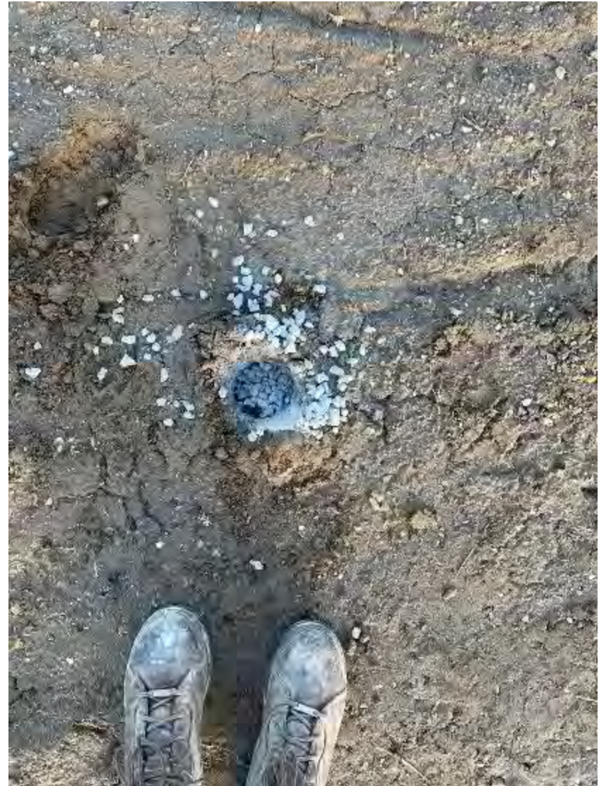
Photo 12. GeoProbe boreholes back-filled with 3/8-inch bentonite chips (cuttings stored onsite in 55-gallon drums).
