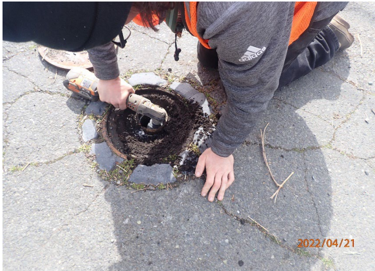
Sentry well MW-8 being repaired using a cut-off tool to level off the broken portion of the 3-inch casing.
