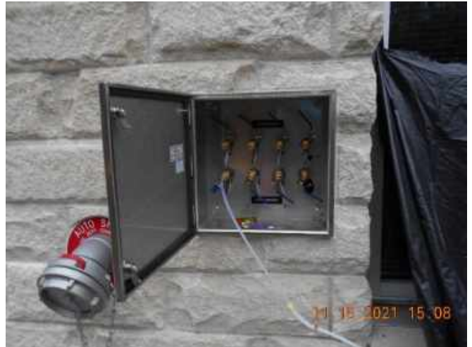
Photograph 2. View of the four above-membrane and four below-membrane VIMS probe outlets.
