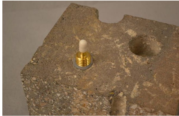
Figure 3. Installed VAPOR PIN® sampling device
