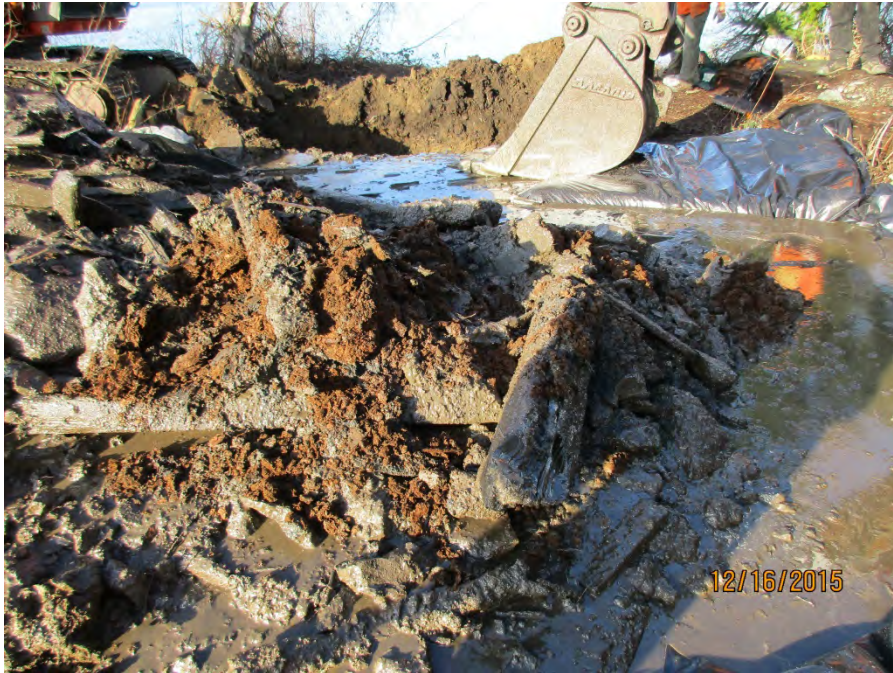
Photo 5: TP-TTWP-S – Wood debris
