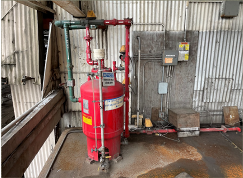
Photo 5: AFFF Tank and Piping on Roof of the 2,500-Ton Press Pump Room (January 2022)
