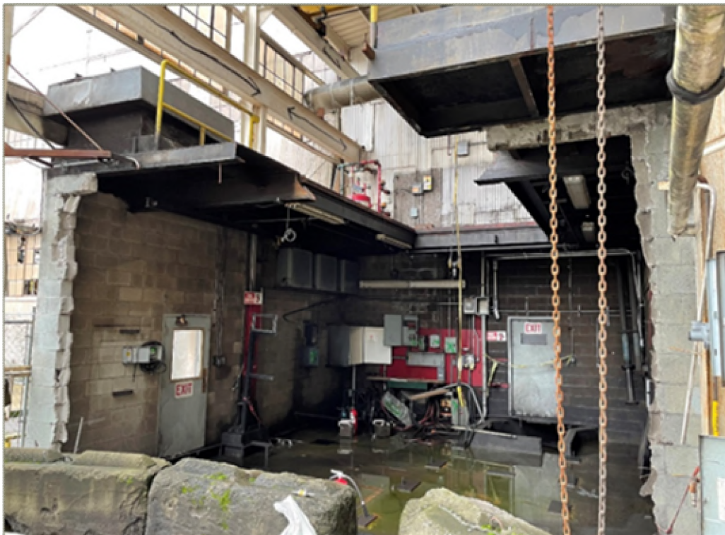
Photo 4: Interior of the 2,500-Ton Press Pump Room (January 2022)
