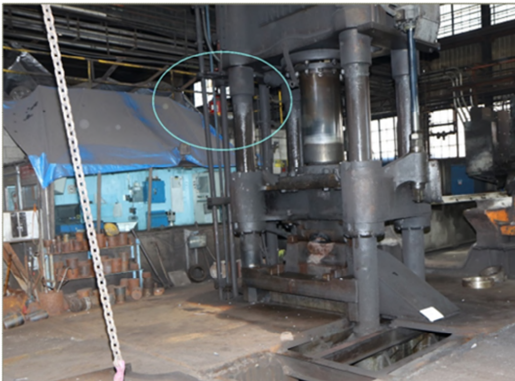
Photo 2: 1,250-Ton Press and Pump Room (September 2018)
