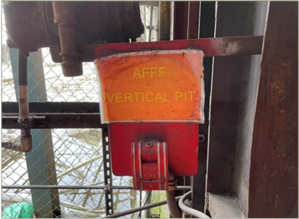
Photo 6: AFFF Placard on Wall Adjacent to Q1/Q2/Q3 Vault (January 2022)
