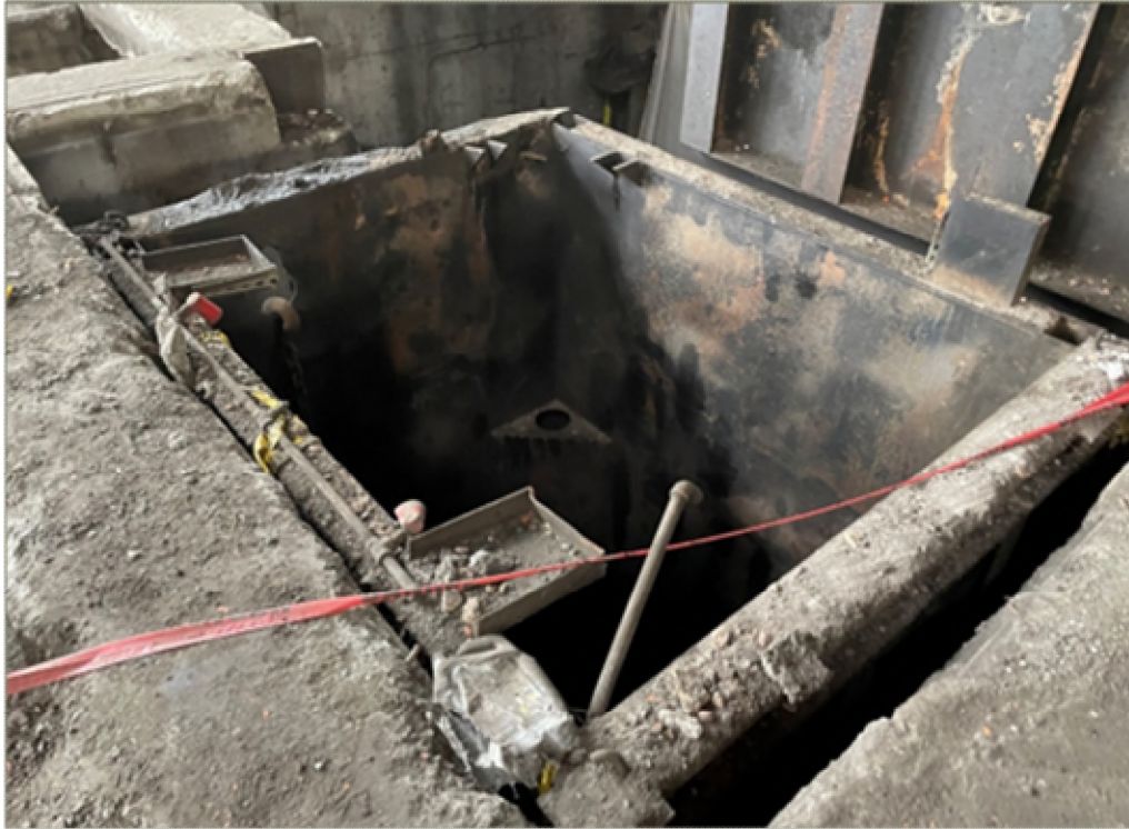
Photo 7: Sprinklers on Westernmost Quench Tank (January 2022)
