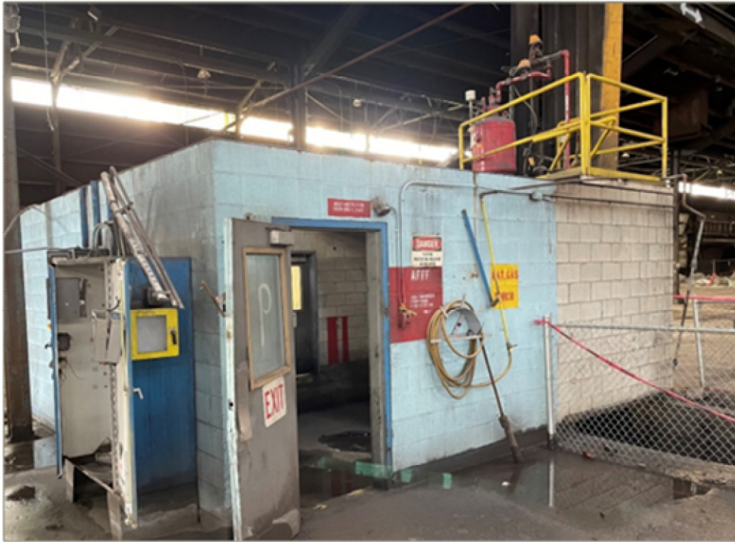
Photo 1: AFFF System at the 660-Ton Press Pump Room (November 2021)
