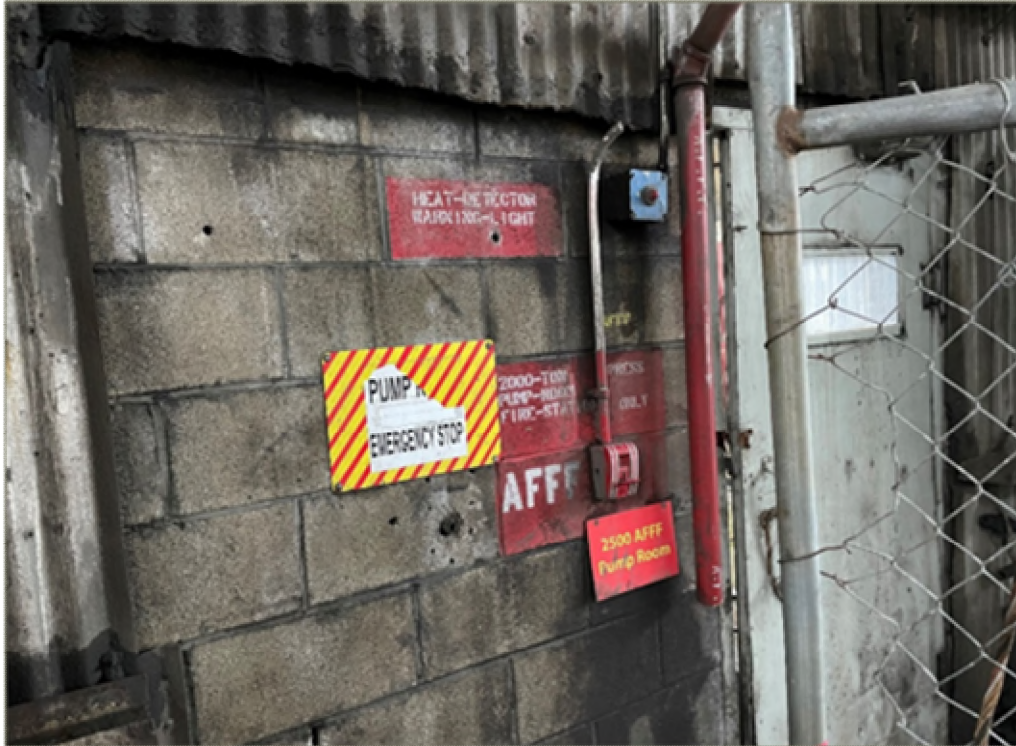
Photo 3: AFFF Wall Decals on the Exterior of the 2,500-Ton Press Pump Room (January 2022)
