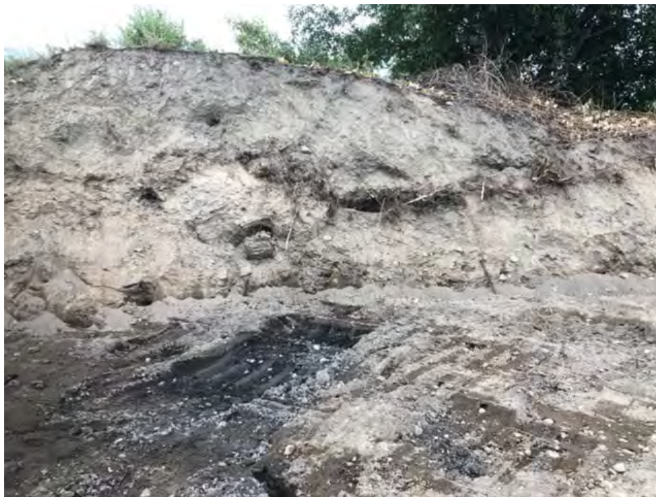
Figure 37: South wall of excavation on Port property. Sand and silt fill with rocks and concrete blocks
