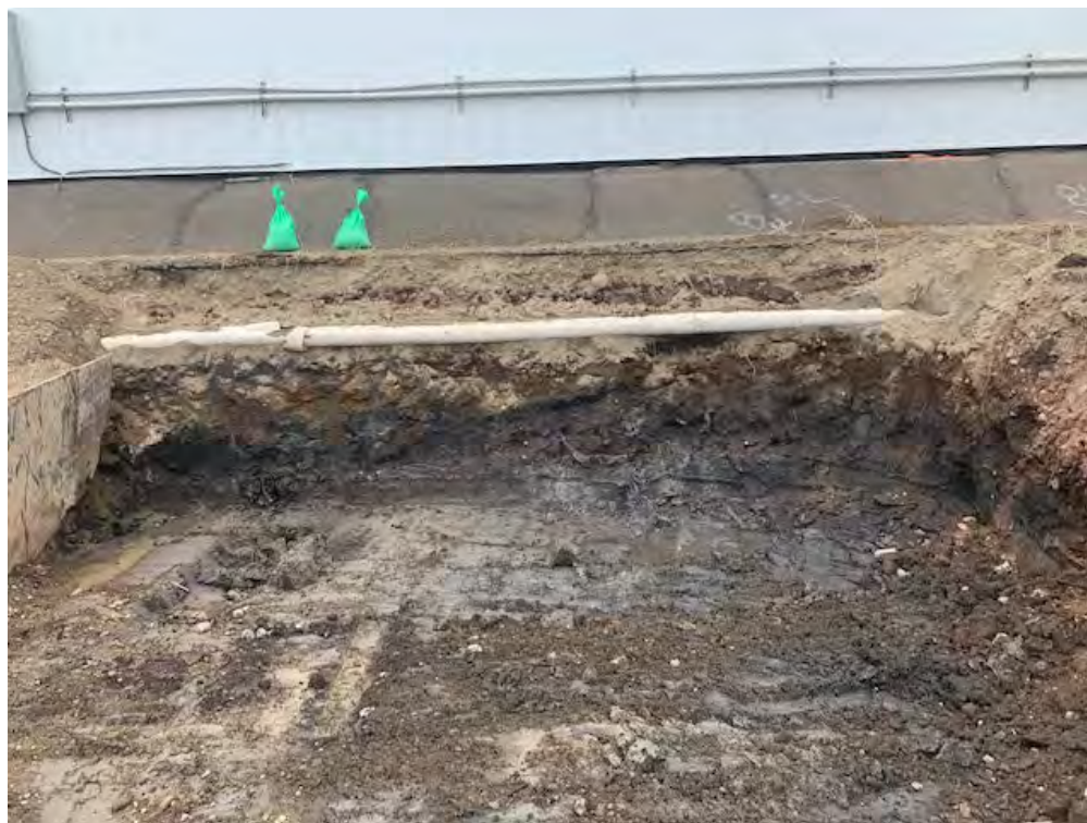
Figure 23: RAU B5: Eastern sidewall at 0-5 feet: Note shot intermixed with soil on the right end of the excavation.
