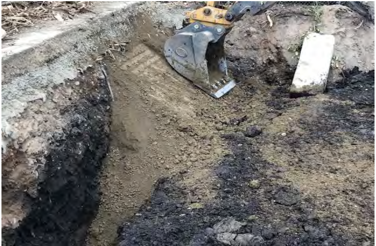
Figure 9: Construction of Clay barrier. Finished product. Note ragged edge of introduced fabric two feet bgs. The fabric was placed below the grade backfill was installed during remediation of the adjacent soils
