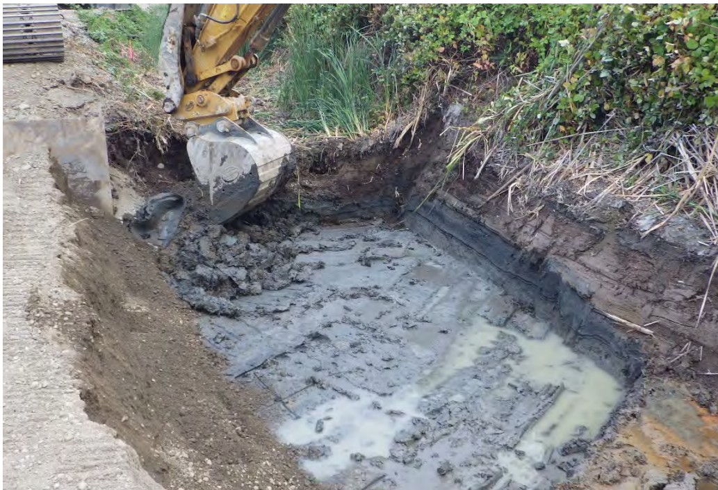
Figure 5-2. Overview of excavation of ditch RAU-D5 at 3 ft below the surface, facing southeast.
