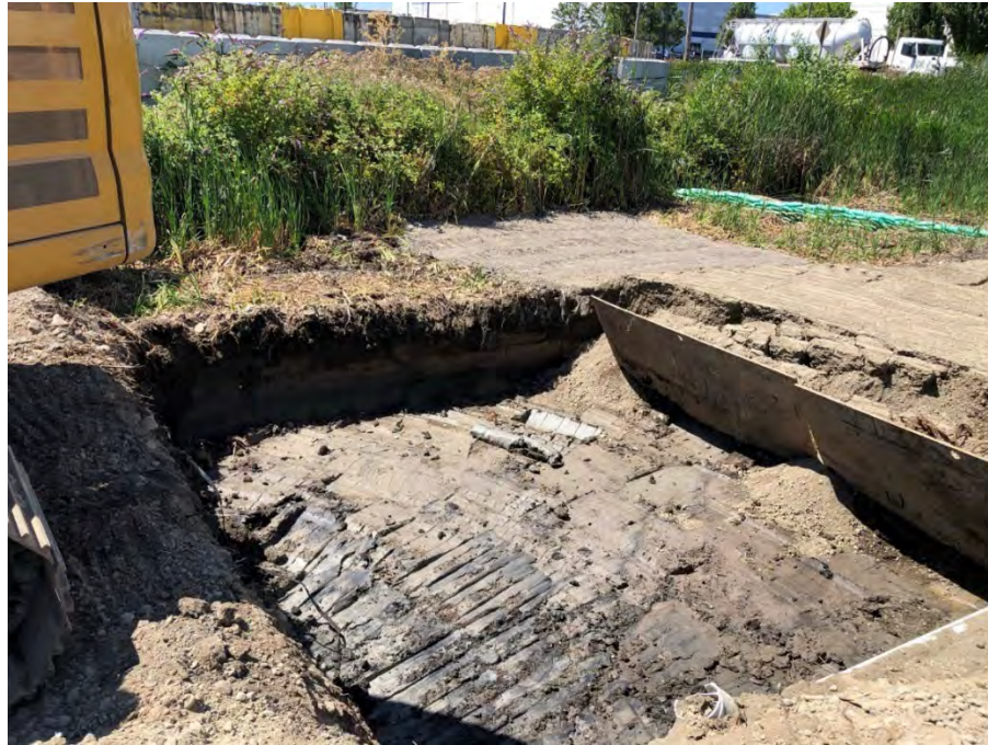
Figure 25: Bottom of RAU B6 – NOTE Steel plates used to prevent sidewall caving
