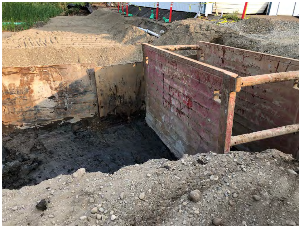
Figure 8: Use of a Trench box and steel sheeting to ensure that all impacted soils are removed and prevent caving.
