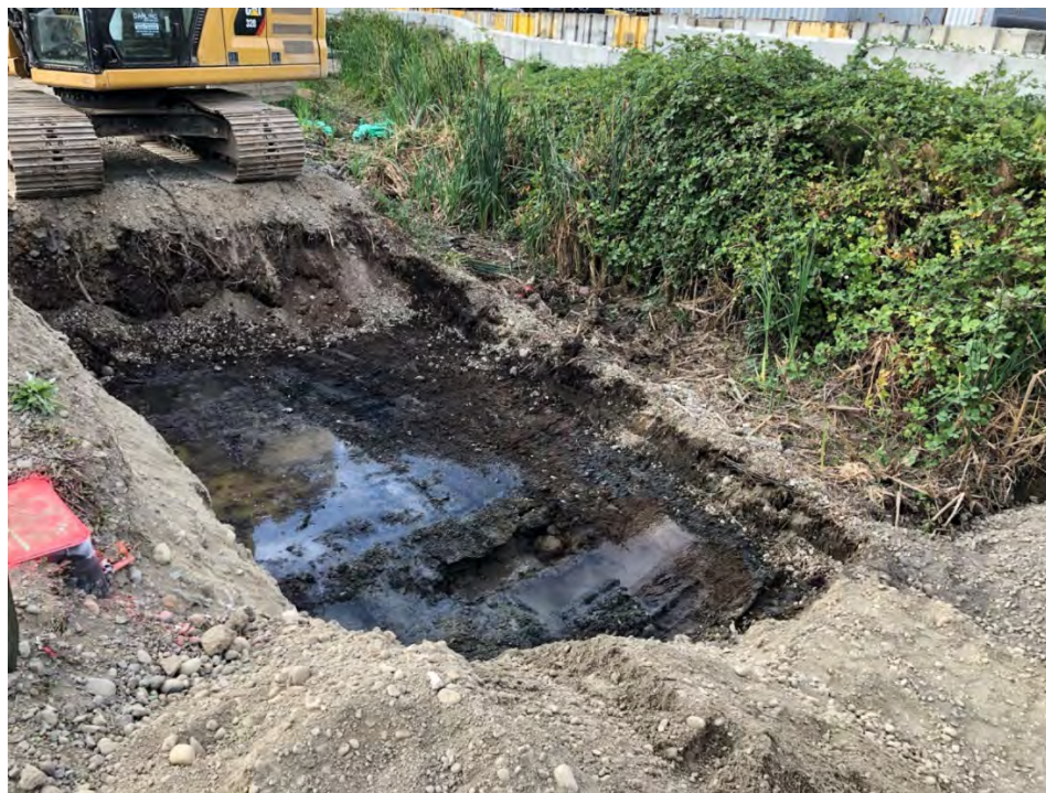
Figure 32: Bottom of RAU B12 - NOTE Narrow width the RAU and oil sheen on water
