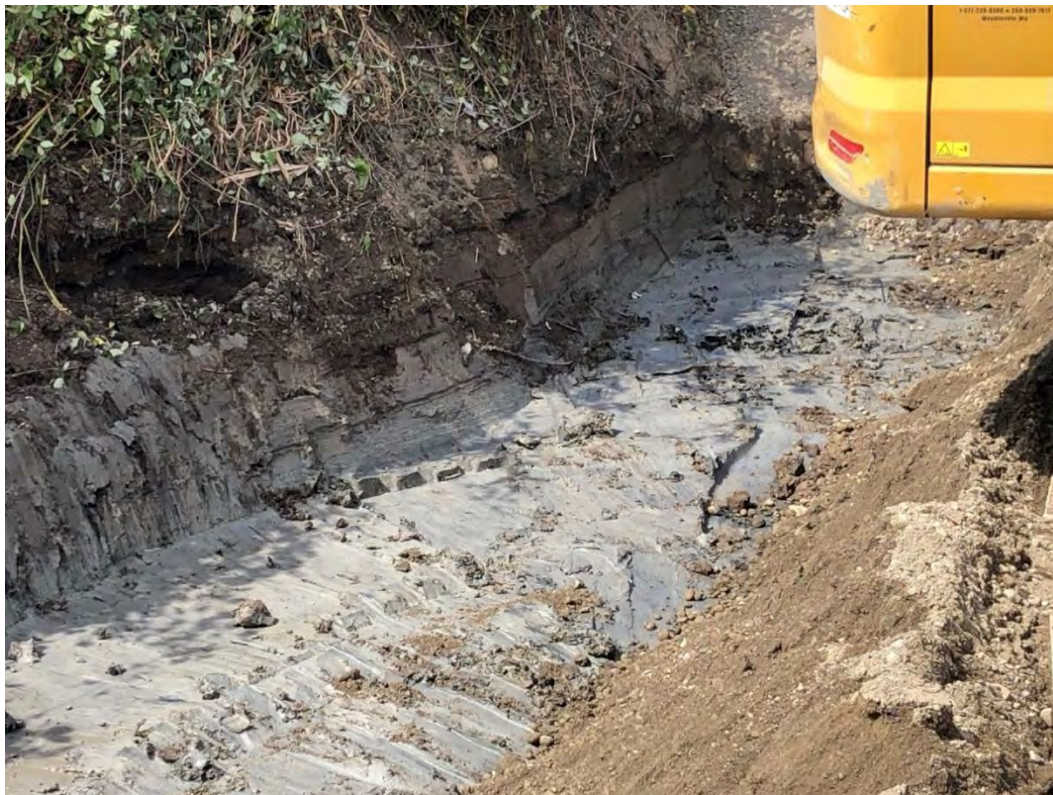
Figure 45: Bottom and western sidewall of RAU D8
