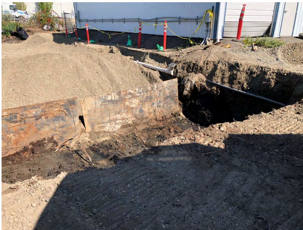
Figure 27: Bottom of RAU B7 – NOTE Steel plates used to prevent sidewall caving
