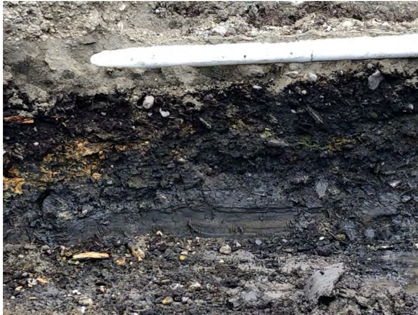
Figure 20: Eastern sidewall of RAU B3 underlying building D on the Superlon property. Note: Drainage line and presence of mixed debris and shot.
