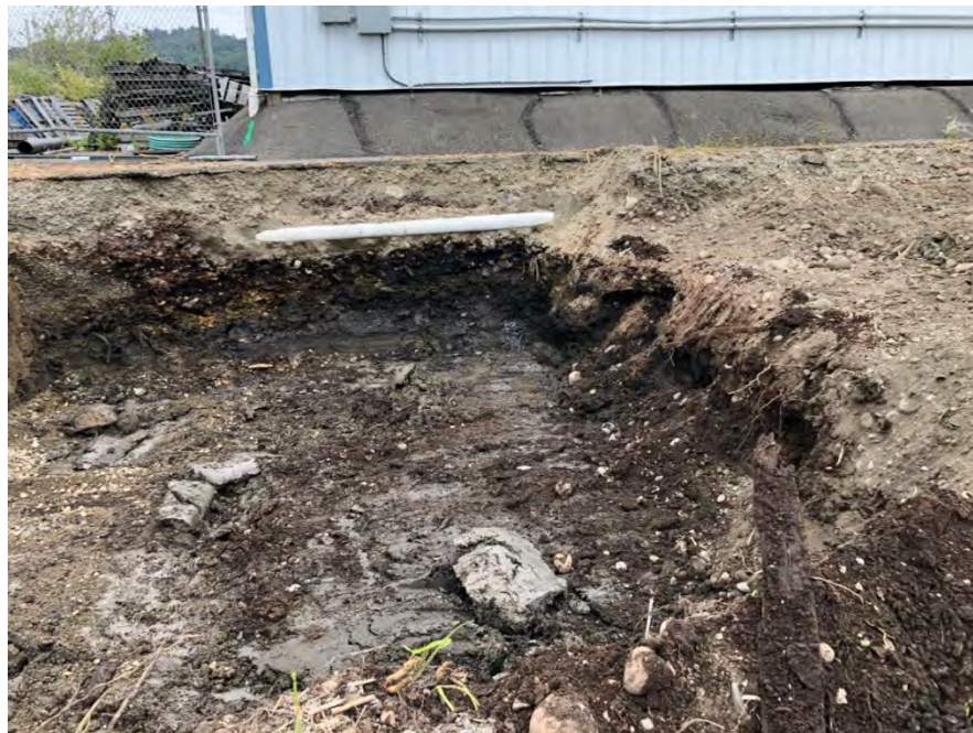
Figure 19: Bottom of RAU B3 - NOTE physical debris and black stained soil in headwall of excavation
