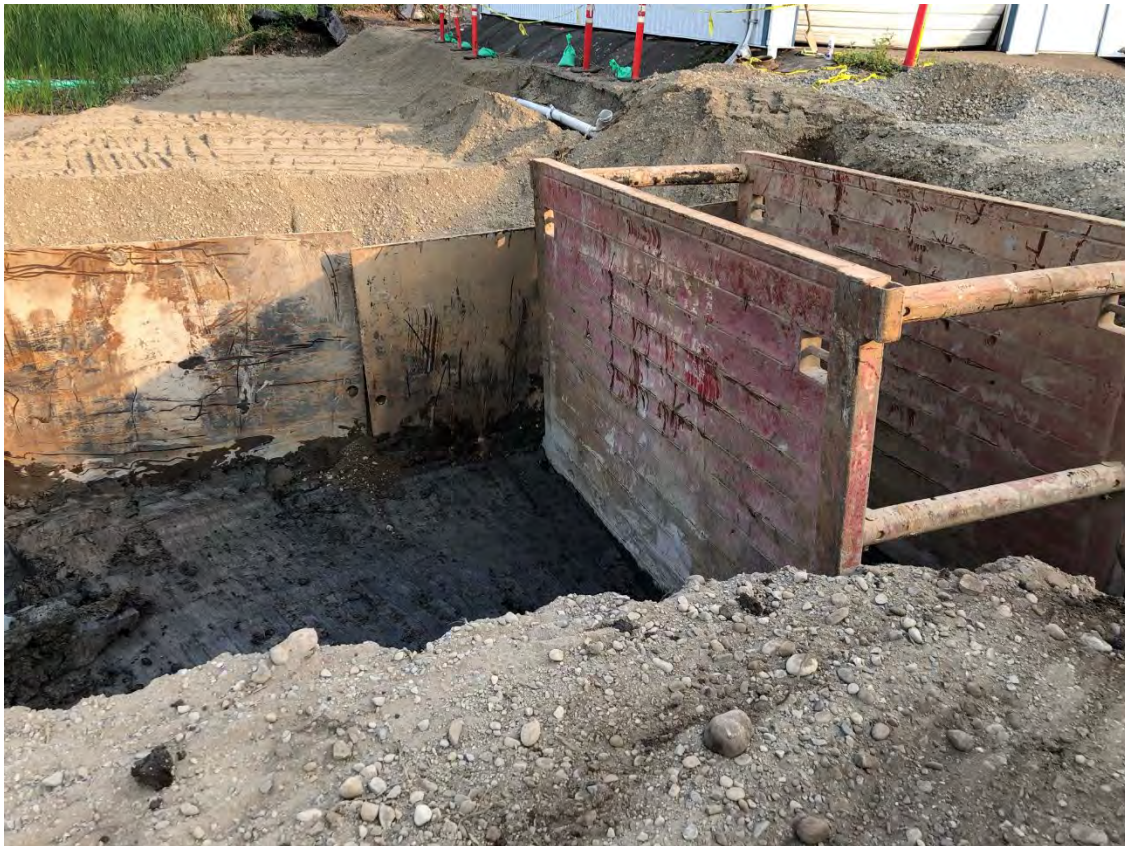
Figure 28: Bottom of RAU B8 – Note use of Trench box and steel sheets to prevent caving
