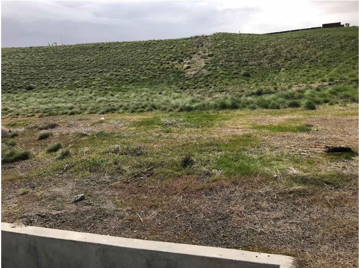
Photo 2 Photo showing condition of cap over part of Area 5 during an inspection for the periodic review.
