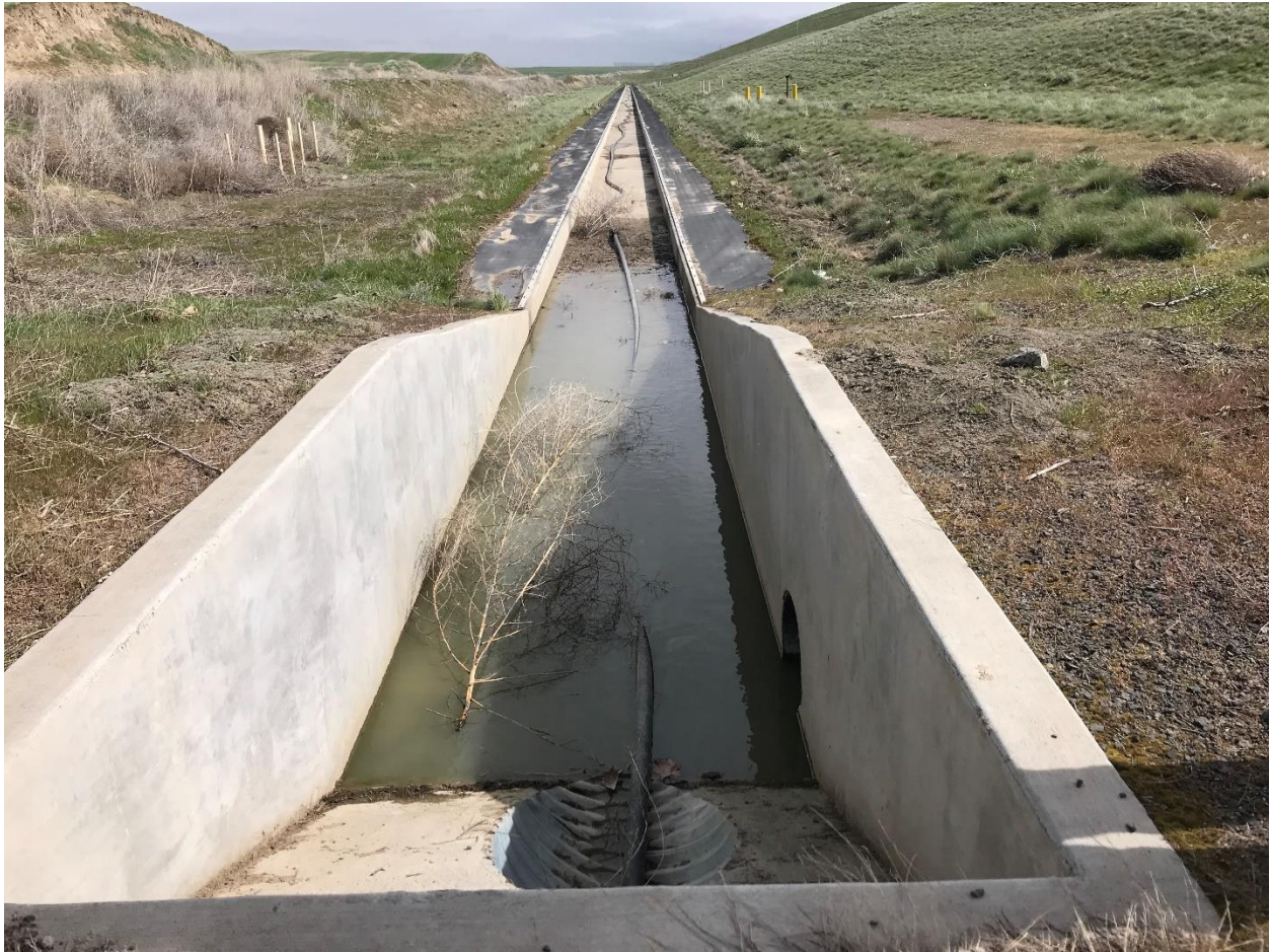
Photo 1 Photo showing condition of north drainage ditch during an inspection for the periodic review.
