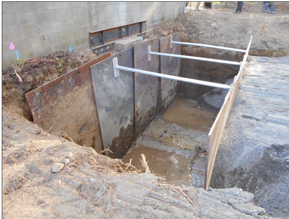
8. Looking east at the Site; groundwater infiltration in Slots A through D.
