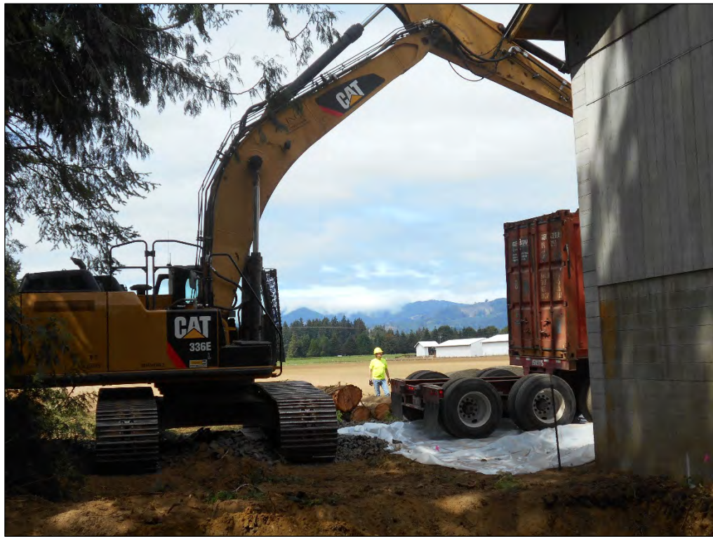
4. Looking west from the Site; direct loading of contaminated soil into awaiting containers.
