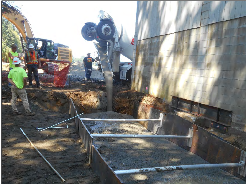
9. Looking west at the Site; placing CDF in Slots A through D.
