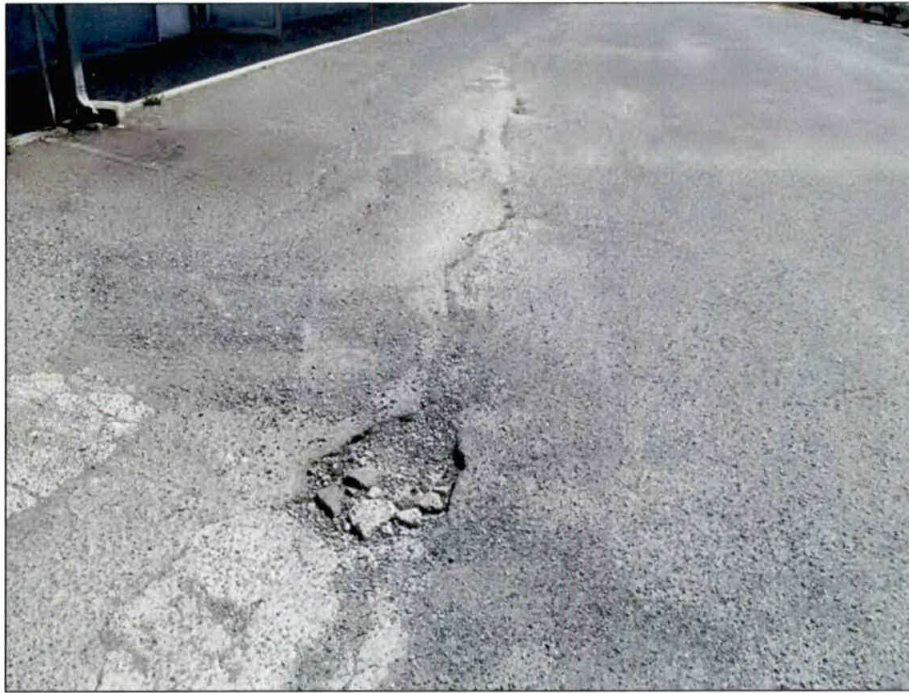
Photograph 15: View of cracks in asphalt parking area west of the building.
