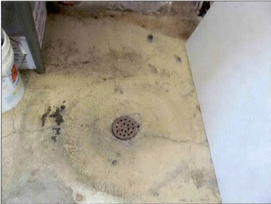
Photograph 10: View of floor drain.
