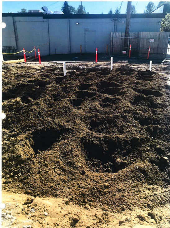
Photo 13 May 12, 2018. Auger mixing Klozur into excavated soil lift at 3 feet. View W
