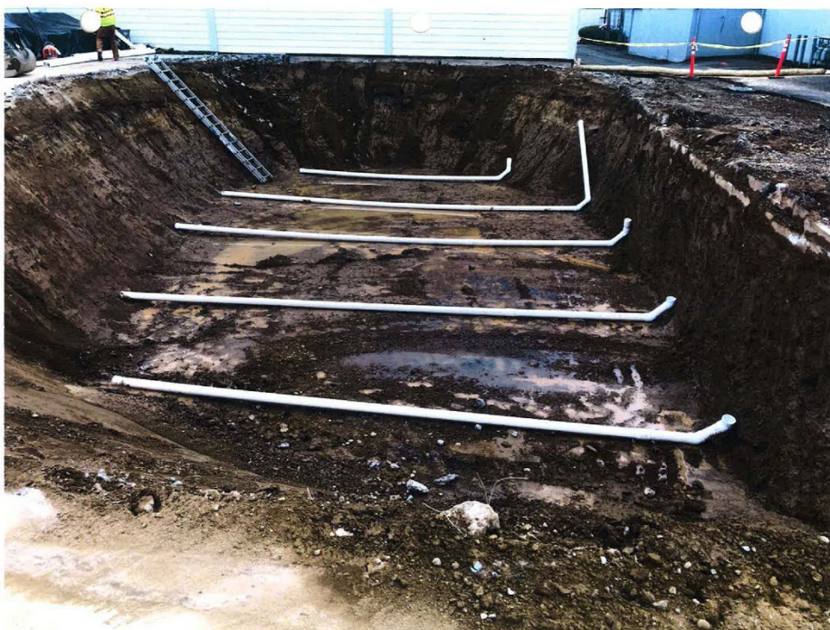
Photo 6 May 11, 2018. 4-Inch PVC pipe runs laid in bottom of excavation. View S
