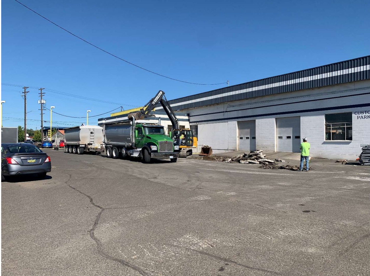
Photograph 8 – Loading contaminated soil in dump truck for disposal on July 12, 2022 (facing NW).
