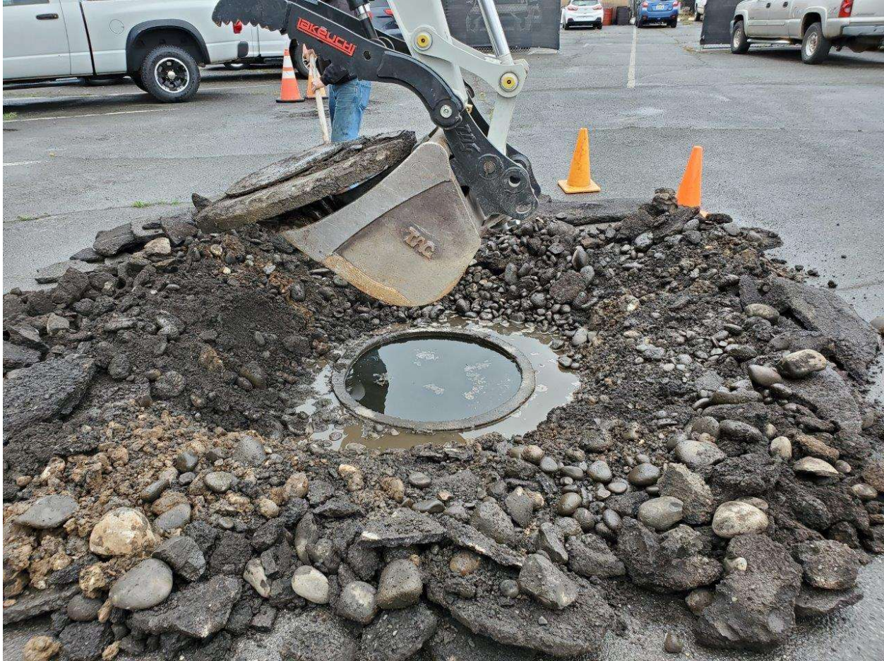
Photograph 1 – Clarke Construction personnel removing lid and assessing Dry Well 2 on July 5, 2022 (facing south).
