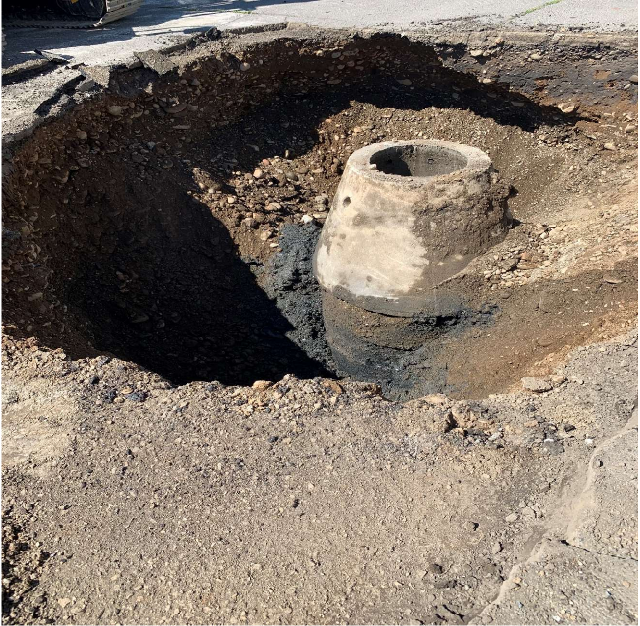
Photograph 12 – PCS depth in vicinity of Dry Well 1 extending to below 5 feet bgs.
