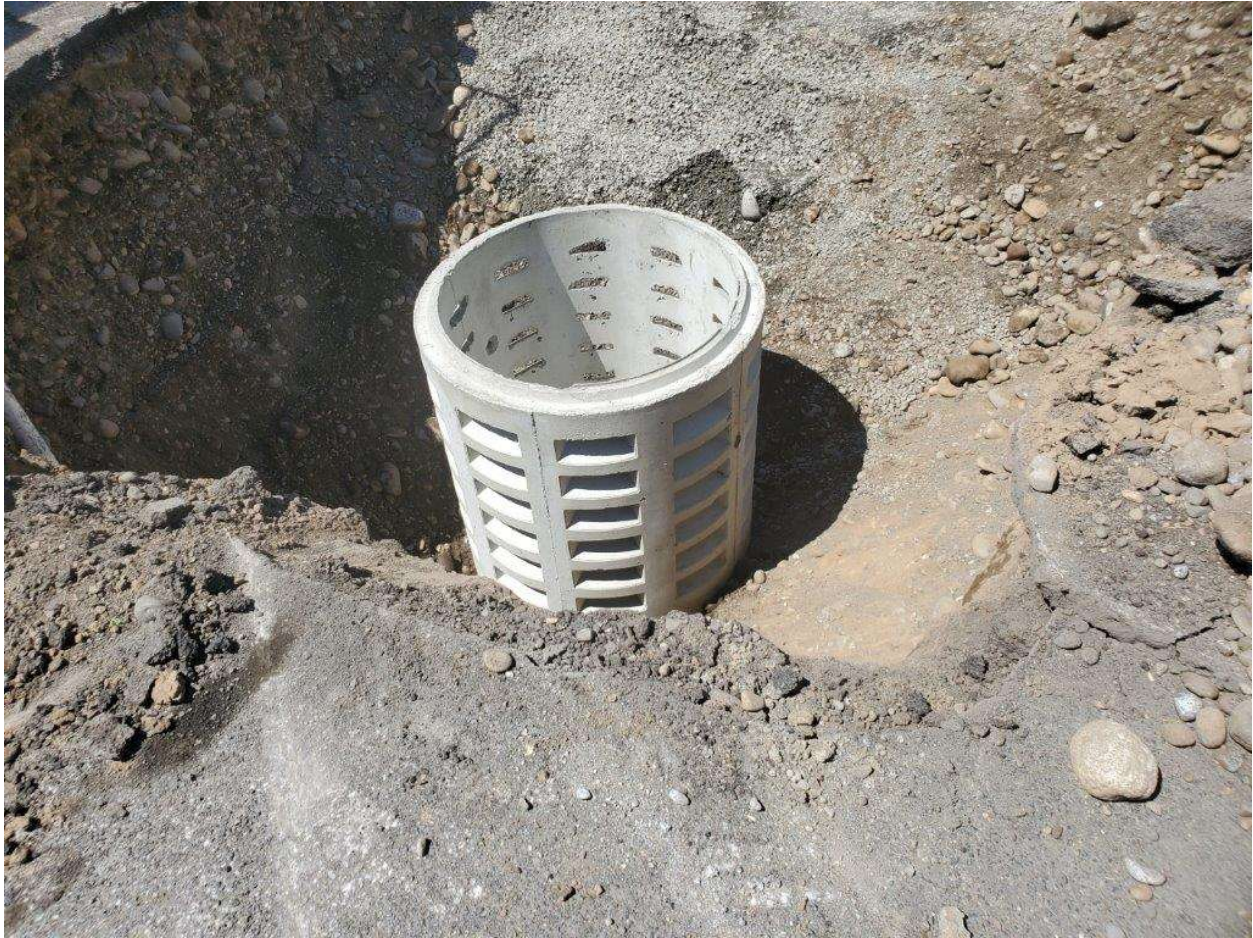
Photograph 20 – New Dry Well being installed near location of former Dry Well 2 on July 14, 2022.
