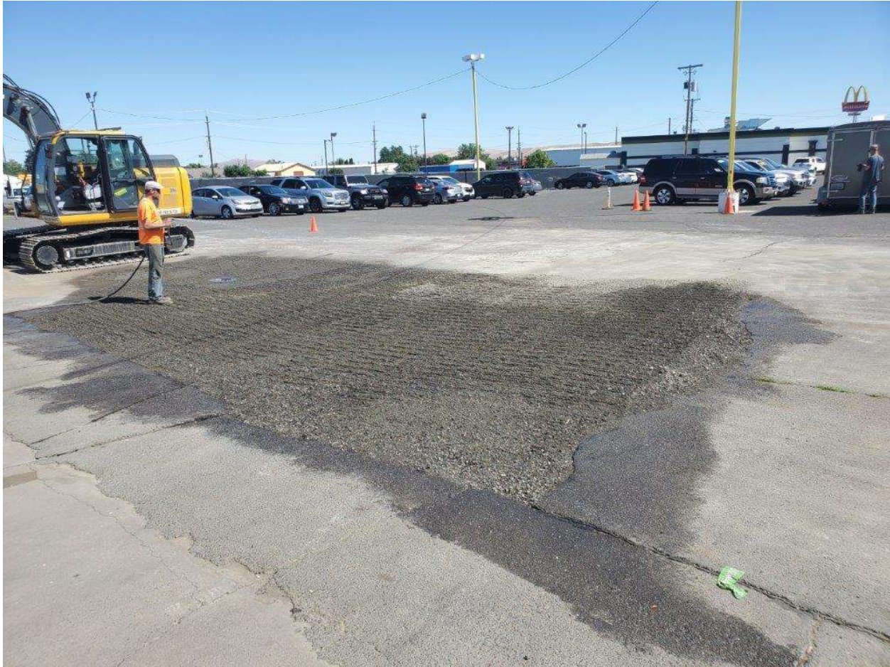
Photograph 21 – View of excavation area after dry well install and backfill, followed by compaction on July 14, 2022 (facing SE).
