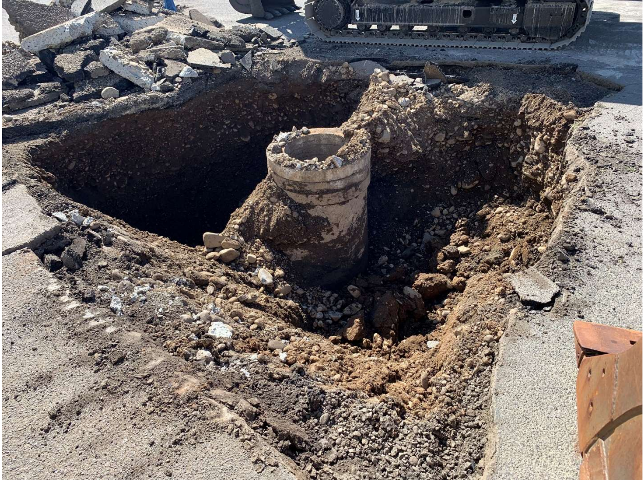
Photograph 9 – Dry well 1 subsequent to soil removal and prior to decommissioning on July 12, 2022 (facing SE).
