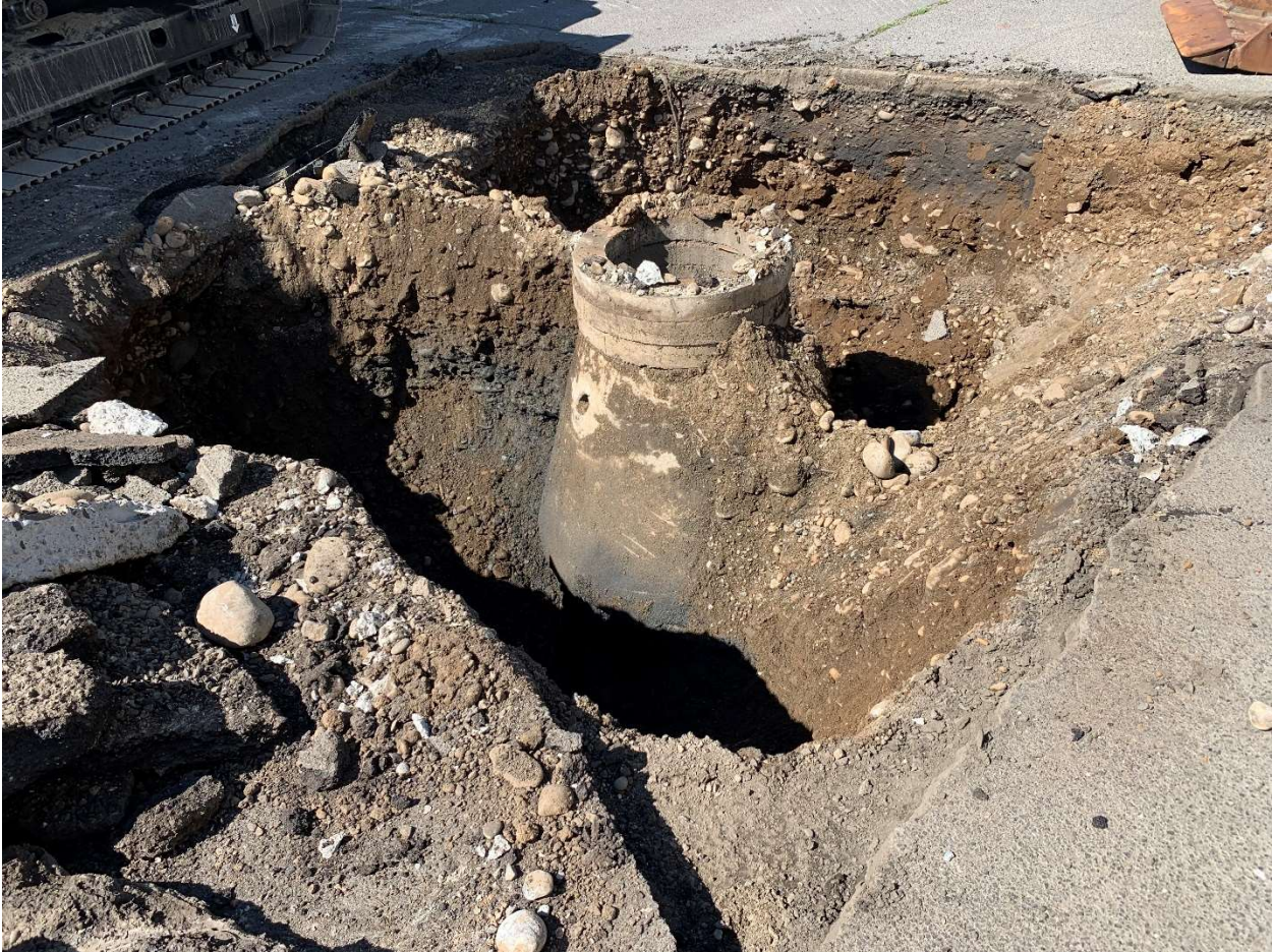
Photograph 10 – Dry well 1 subsequent to soil removal and prior to decommissioning on July 12, 2022 (facing SW). Note dark stained petroleum-contaminated soil (PCS).
