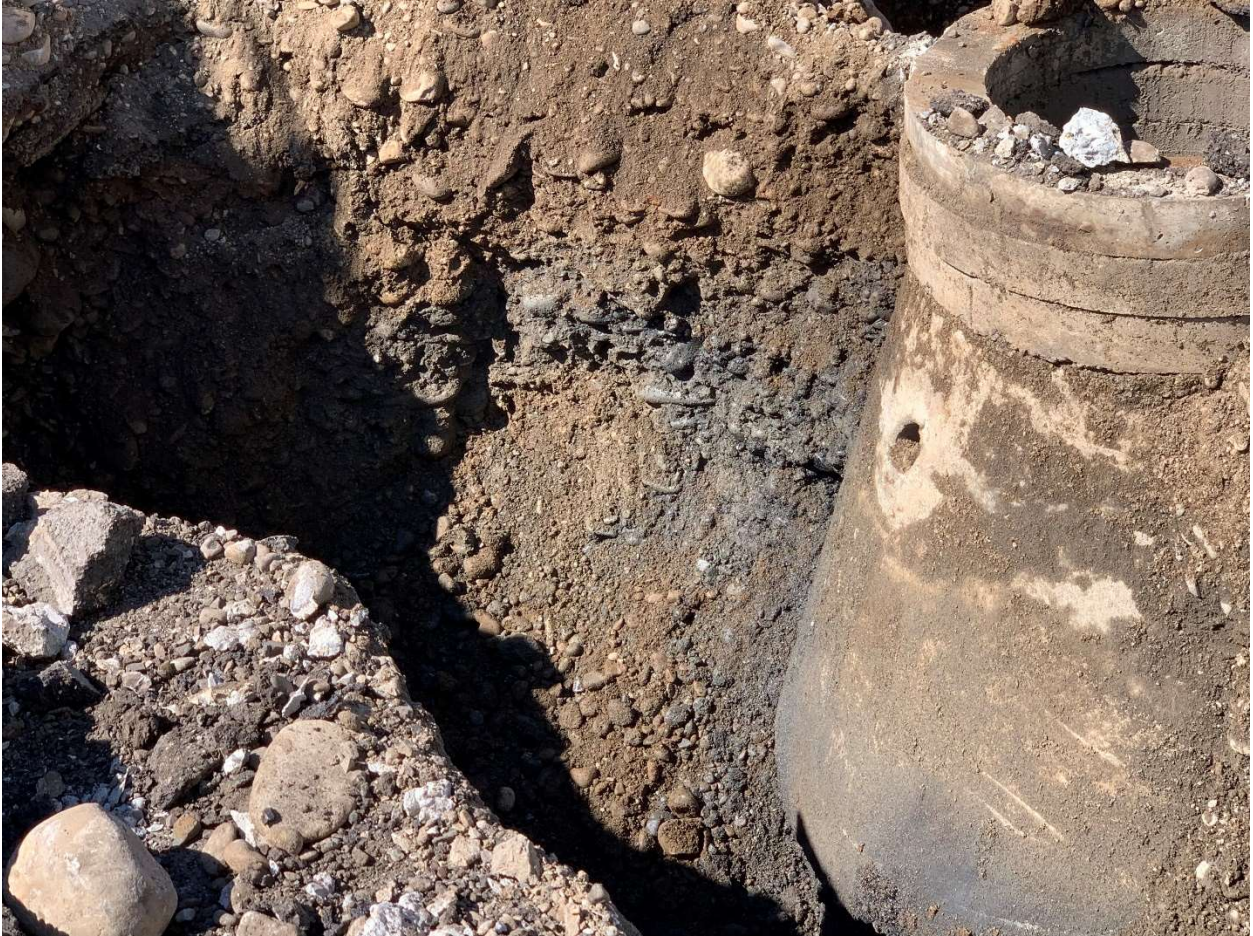
Photograph 11 – Close-up of PCS in vicinity of Dry Well 1.
