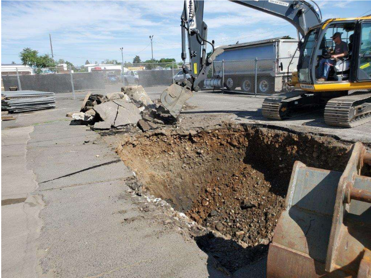
Photogrpah 16 – Clarke Construction continuing excavation to east toward Dry Well 2 on July 12, 2022 (facing east).
