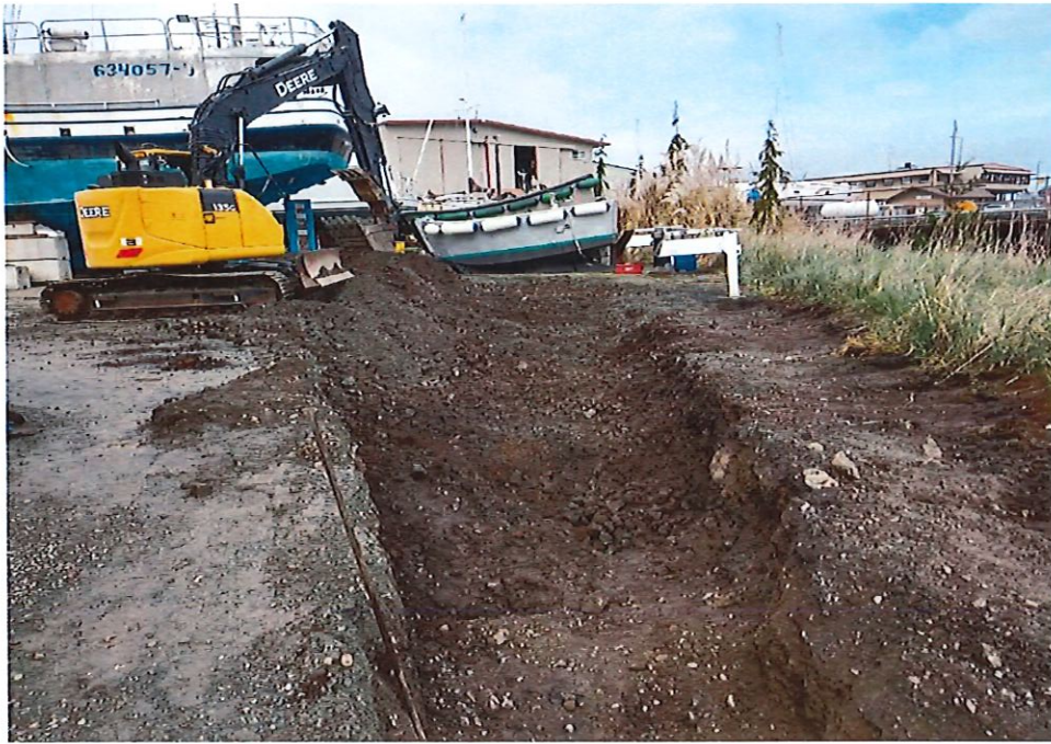
5. Looking north at remediation area. The final northerly 30' of the spill area was limited to an approximate excavation depth of 8" – 12". The original spill occurred during a cold, snowy and frozen February time frame. It is speculated that the spill traveled over the frozen ground. Because of the quick emergency response by Northern Environmental, any fuel puddling was limited to the southern area of the spill.
