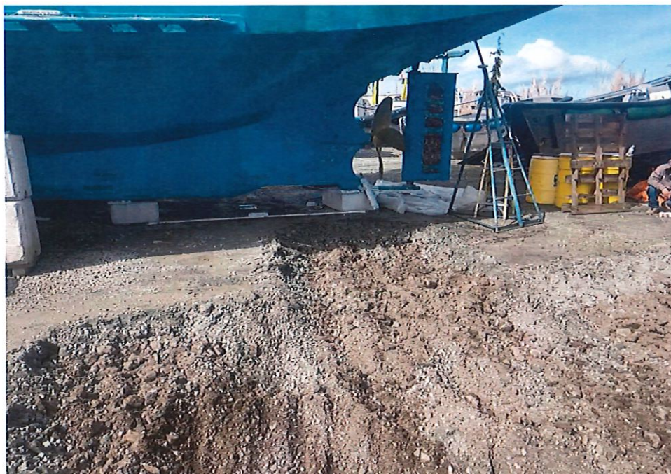
8. Looking north at the excavation area directly under the vessel scuppers (original spill area).
