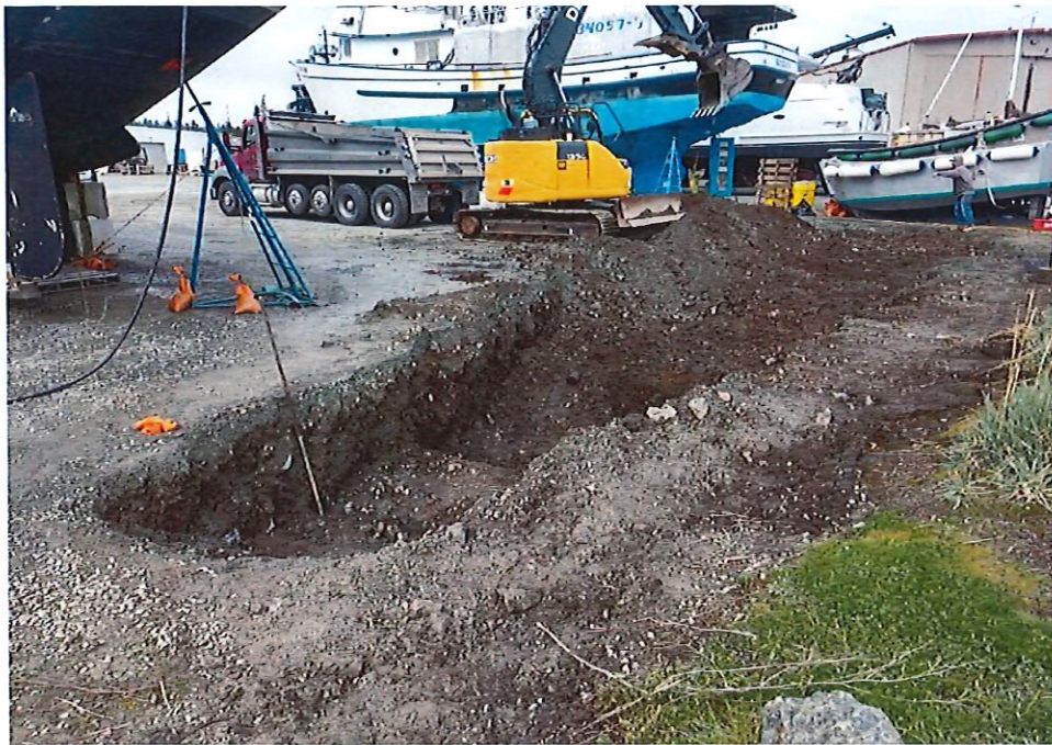
7. All PCS was loaded directly into dump trucks for hauling and disposal at the licensed Cadman thermal desorption facility in Everett, WA.
