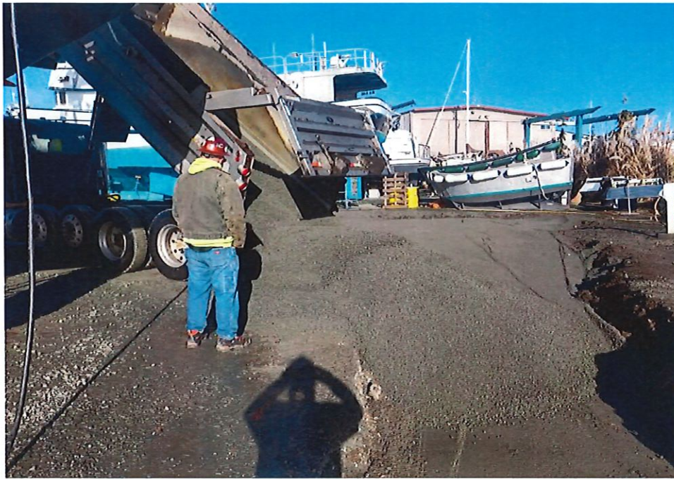
9. Following receipt of confirmation soil sample analytical, the excavation area was backfilled and compacted with clean crushed rock material.
