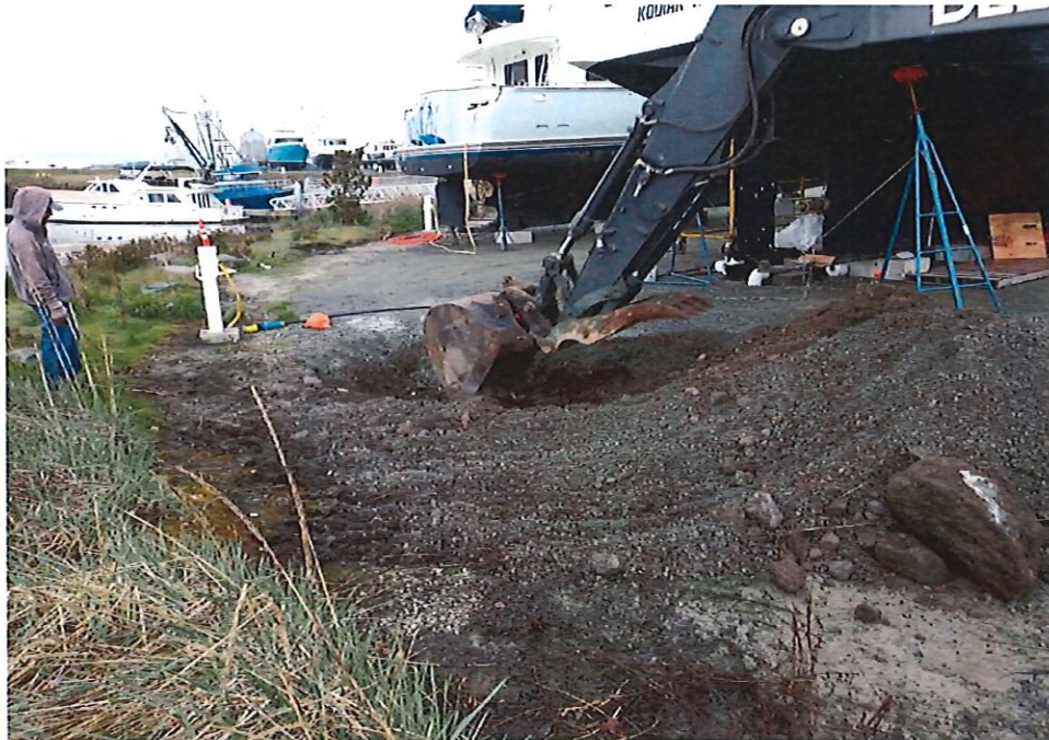
4. Looking south at the approximate middle of remediation area. The southerly 30' dug to an approximate depth of 3 ½'. One area, approximately 16' from south end, excavated to a depth of 6'.
