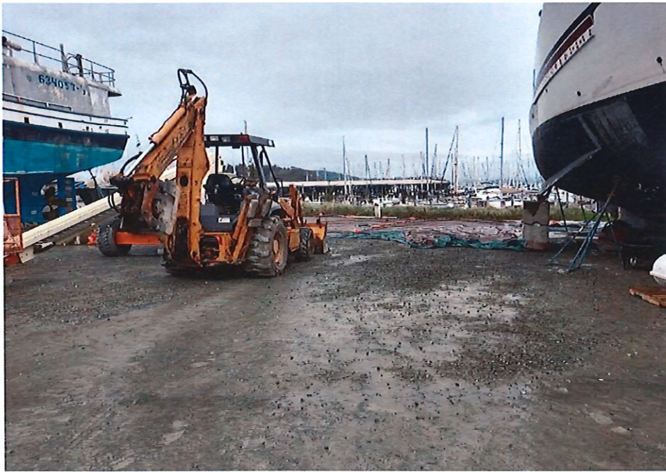
1. Looking east at spill area prior to remediation project. Note the spill area covered with poly sheeting.
