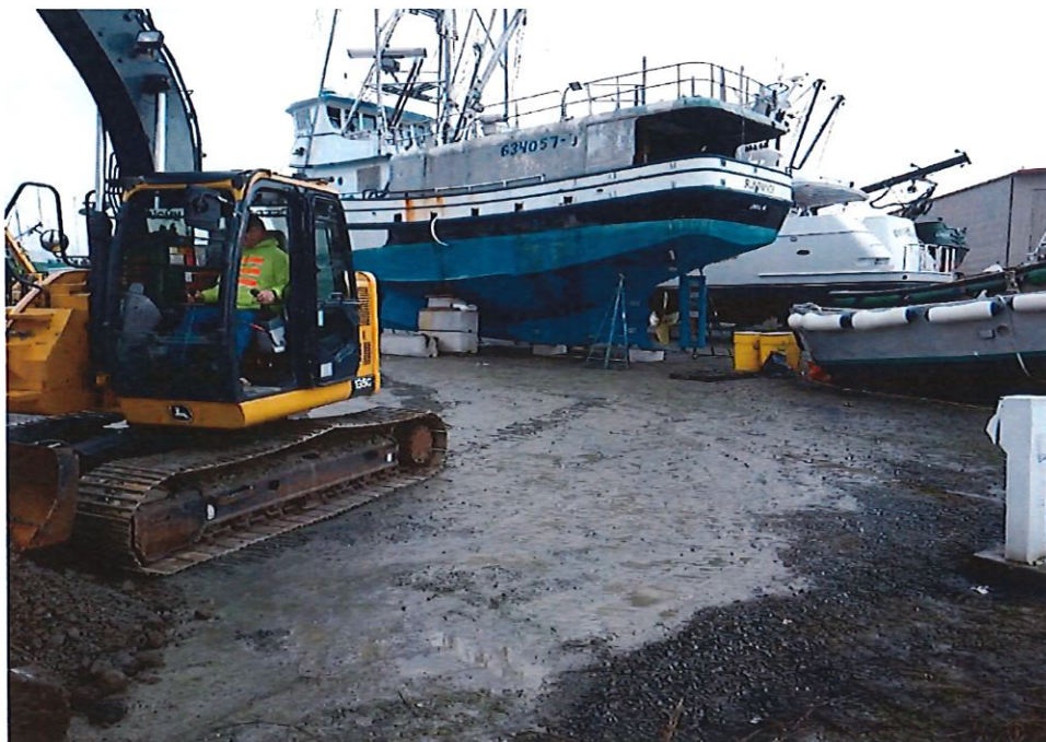
2. Looking north at the start of the PCS excavation in the south end of the spill area. Note the fuel stains on the east end of the Sundance vessel scuppers.
