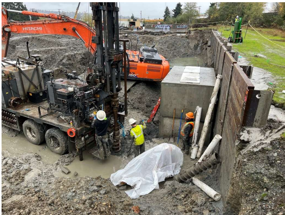
41. CAA-4, hollow stem auger drilling gravity well. View to the east. Photograph taken 11/12/2021.
