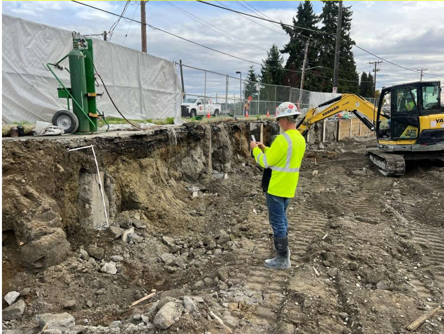
13. CAA-2b ROW area, measuring cut soldier piles for SDOT inspector. View to the northeast. Photograph taken 10/21/2021.
