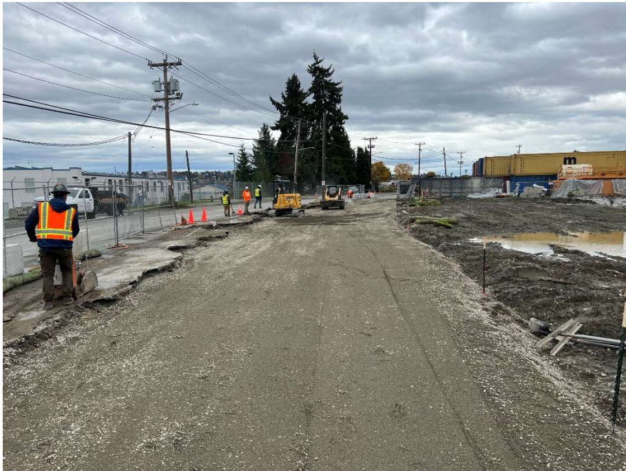
14. CAA-2b ROW area, laying down and grading baserock for asphalt. View to the east. Photograph taken 10/25/2021.
