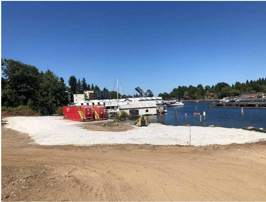
32. Backfilling and grading ballast rock at remediated CAA-7 excavation. View to the west. Photograph taken 7/29/2021.
