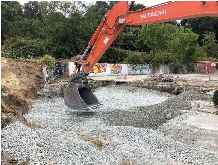
21. Backfilling and compacting CAA-5 with ballast rock. View to the southwest. Photograph taken 8/17/2021.
