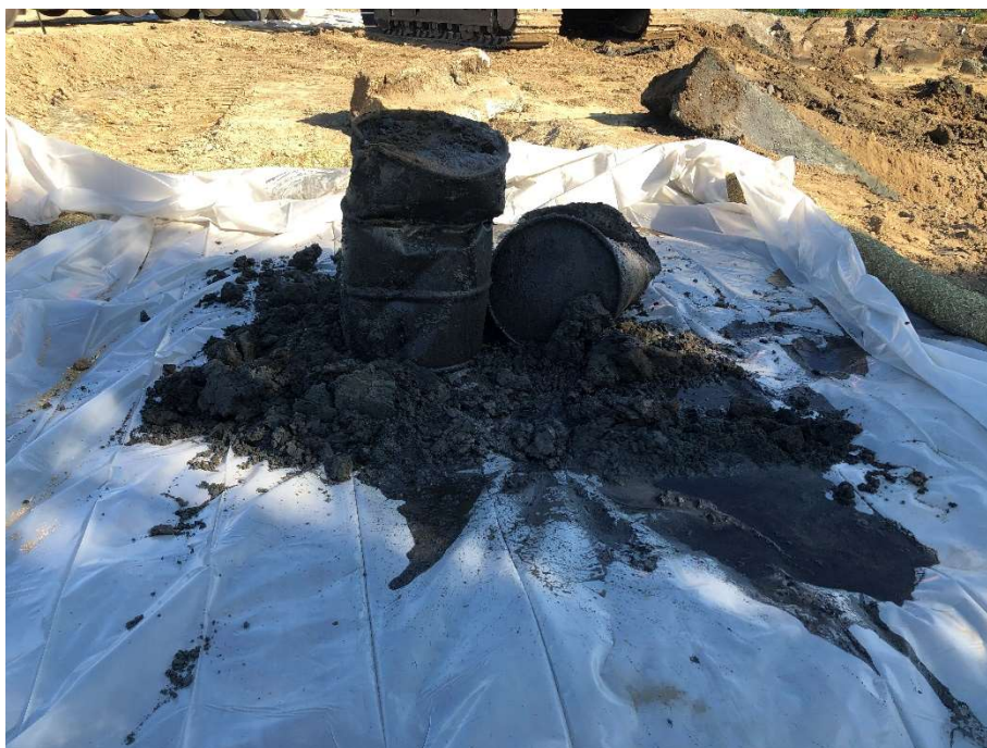
23B. Two 55-gallon drums removed from CAA-6a. Staged on plastic sheeting, bermed, contained in CAA-6a footprint. Photograph taken 7/26/2021.
