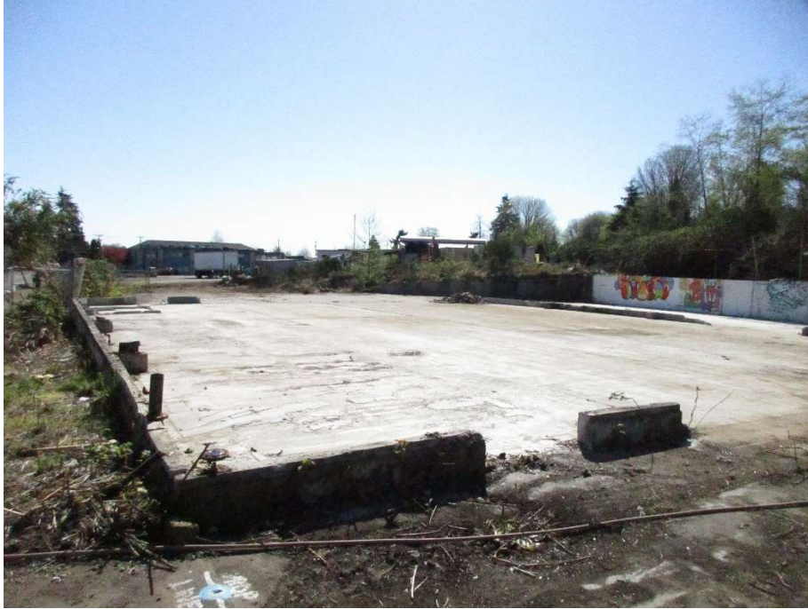
1. ASKO warehouse foundation pad. Warehouse demolition debris and steel hauled off. View to southeast. Photograph from 4/16/21
