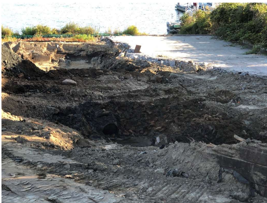
23A. CAA-6a. Two uncovered, buried drums. Shown in-situ. View to the north. Photograph taken 7/26/2021.
