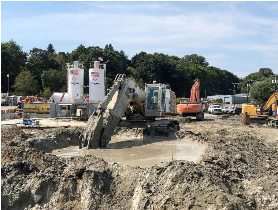
34. Bucket mixing soils and grout at ISS Cell 2-38. View to the west. Photograph taken 9/7/2021.
