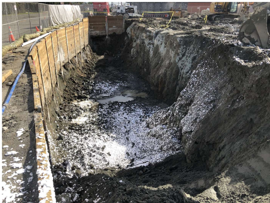
10. CAA-2b, excavation with odor suppressant foam (white foam). View to the east. Photograph taken 10/2/2021.
