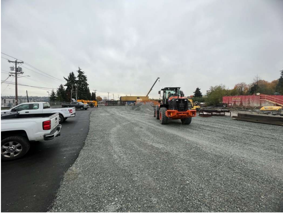
36. CAA-2a completed surface photo. New black asphalt shows CAA-2b ROW. View to the east. Photograph taken 11/2/2021.
