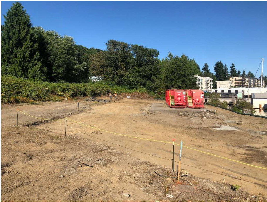
30.CAA-7 post-remedial surfaces. Site conditions at following completion of excavation at CAA-7. View to the west. Photograph taken 7/23/2021.
