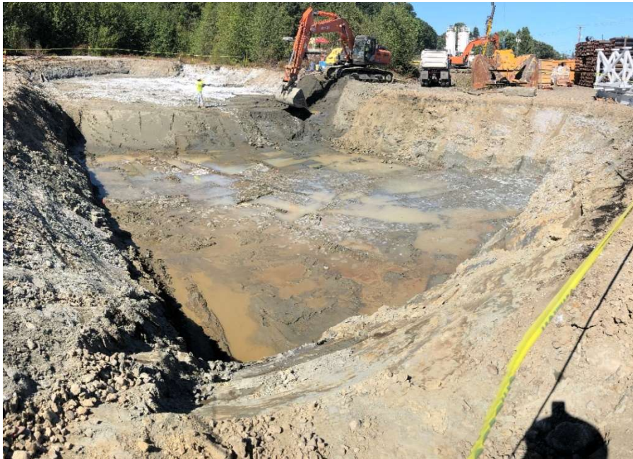
6. CAA-1b excavation progress with odor suppressant foam (white foam) on CAA-1a. View to the southwest. Photograph taken 8/11/2021.
