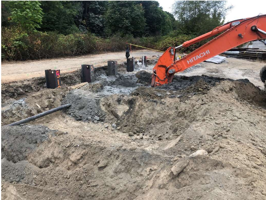
37. Bucket-mixing shallow soils and grout at CAA-4 along southern property line. View to the southwest. Photograph taken 9/10/2021.
