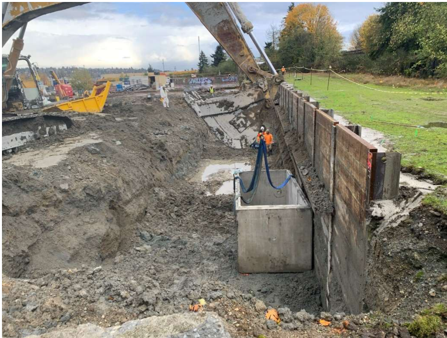
39. CAA-4, positioning concrete vault along interceptor trench. View to the east. Photograph taken 11/9/2021.
