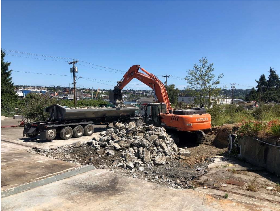
5. Concrete hauling and recycling at CAA-5 (site preparation). View to the northeast. Photograph taken 7/29/2021.
