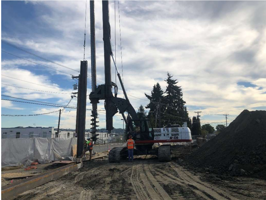
9. Installing soldier pile steel beams at CAA-2b/ROW. View to the east. Photograph taken 9/9/2021.
