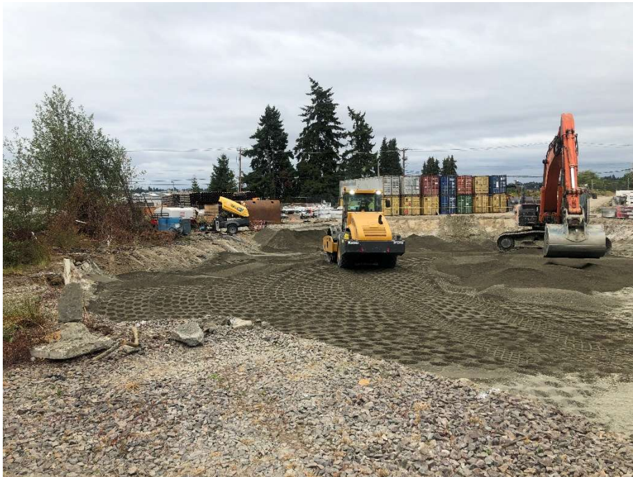
8. CAA-1a - Backfilling and compacting gravel borrow at CAA-1a. View to the northeast. Photograph taken 8/20/2021.
