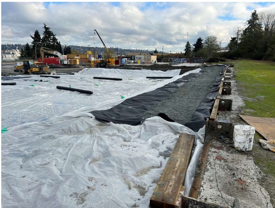
45. CAA-4 interceptor trench area, covered in plastic sheeting as a BMP. Vault in center bottom, trench covered in geotextile and ballast rock. View to the east. Photograph taken 11/23/2021.
