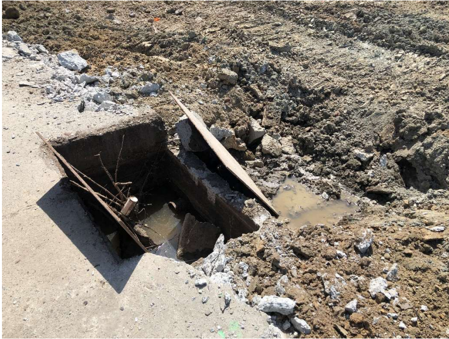
24. Vaults along eastern perimeter of CAA-6a. Inside former building footprint. Photograph taken 7/22/2021.
