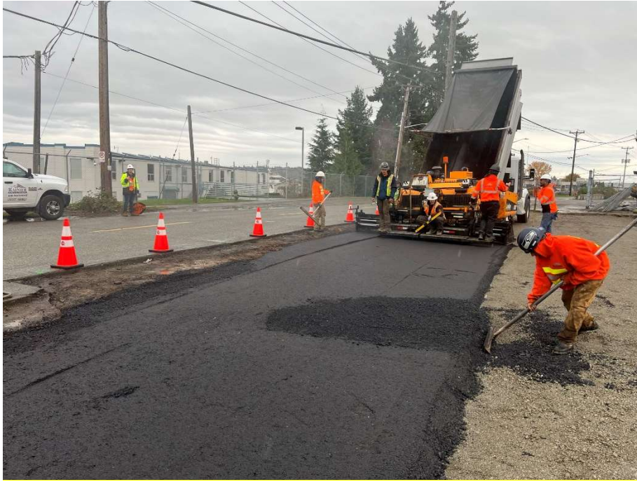
15. Rainer Asphalt & Concrete laying down hot mix asphalt at ROW of CAA-2b. View to the east northeast. Photograph taken 10/26/2021.
