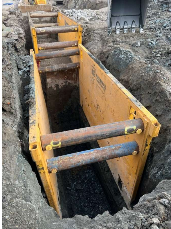
12. CAA-2b trench box area excavation underway. View to the east. Photograph taken 10/16/2021.
