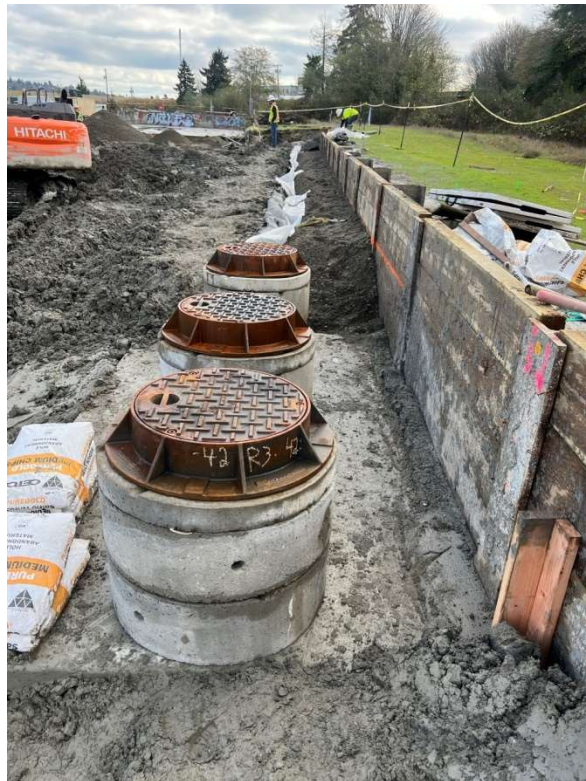
43. CAA-4 top of treatment vault, three manhole pipes in place (to be grout sealed). View to the east. Photograph taken 11/20/2021.
