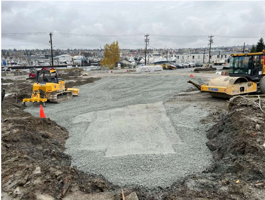
18. CAA-3 largely backfilled, ballast rock at surface. View to the north. Photograph taken 11/13/2021.
