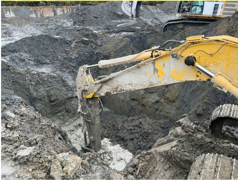
38. CAA-4, ISS bucket-mixing soil and grout at Cell 4-43. View to the southwest. Photograph taken 10/26/2021.
