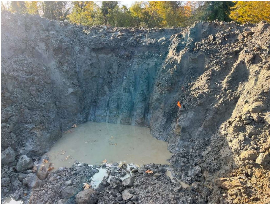
16. CAA-3, pin flag at CAA3-SS-04 confirmation wall sample location (surface water collected at the bottom of the excavation).View to the south. Photograph taken 11/9/2021.
