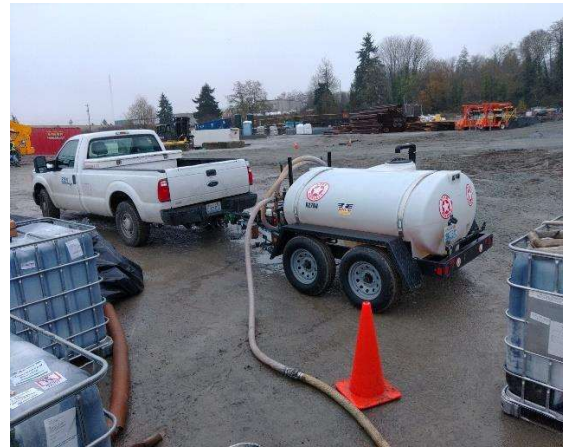
Photo 2: View of 500-gallon water wagon provided by ESN that is connected to RRS injection trailer. Southeast view.
