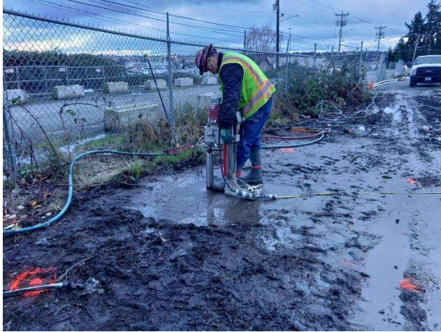
Photo 5: A concrete coring drill was brought out to pre-core IP-31 to IP-35. Northeast view
