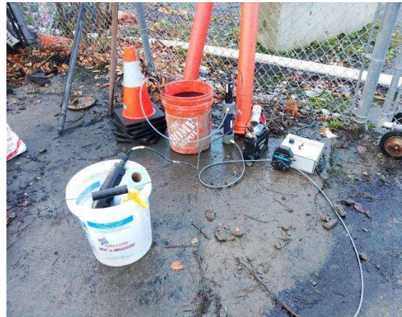
Photo 4: View of Floyd Snider's monitoring well equipment.
