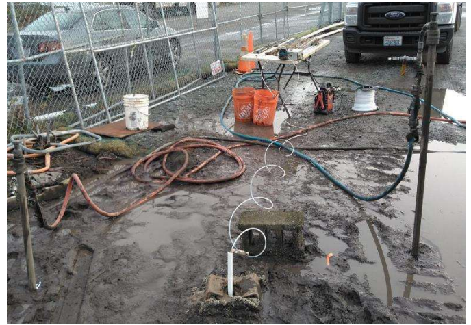
Photo 6: A piezometer was installed between IP-47 (left) and IP-48 (right). Northeast view.
