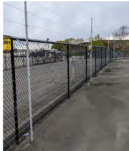
SPPD AC-6: New electric fence
