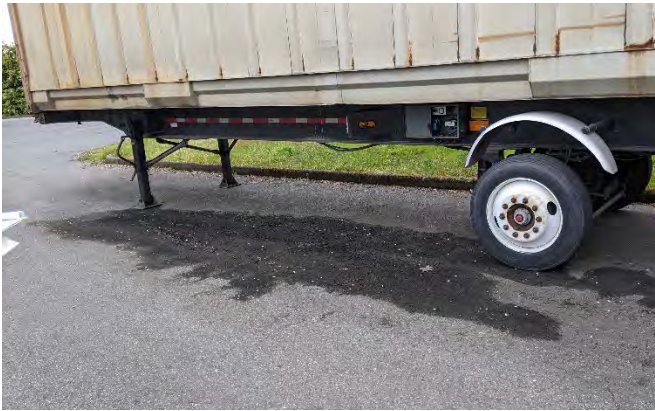
SRDS AC-4: Ponding
