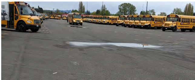
SPPD AC-11: Ponding
