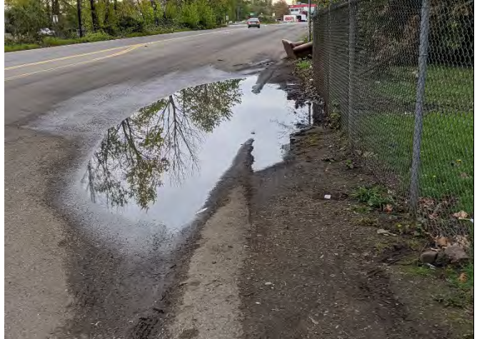
SRDS AC-17: Ponding
