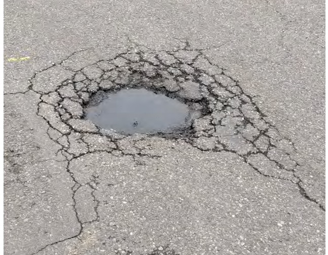
SRDS AC-5: Pothole
