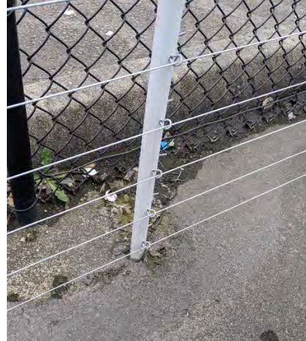
SPPD AC-6: New electric fence
