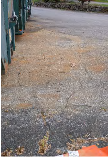
SRDS AC-16: Minor cracking
