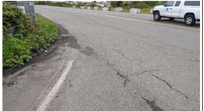
SRDS AC-11: Ponding
