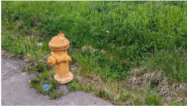
SPPD AC-2: Depression at fire hydrant
