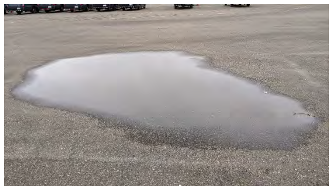
SPPD AC-4: Ponding
