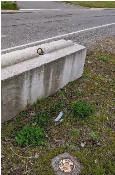
ROW AC-2: Cracking
