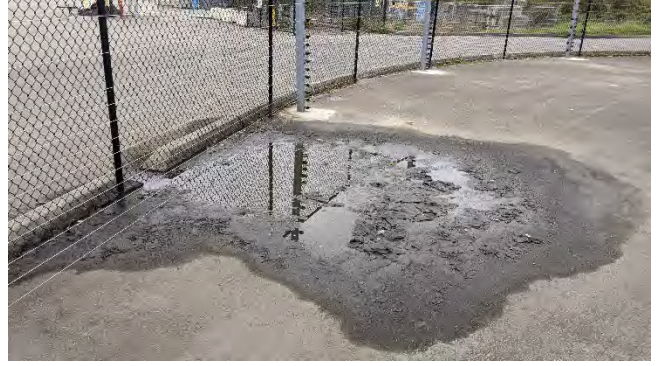
SPPD AC-10: Ponding
