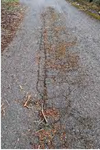
SRDS AC-13: Minor cracking and rutting
