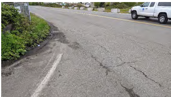
SRDS AC-12: Minor cracking
