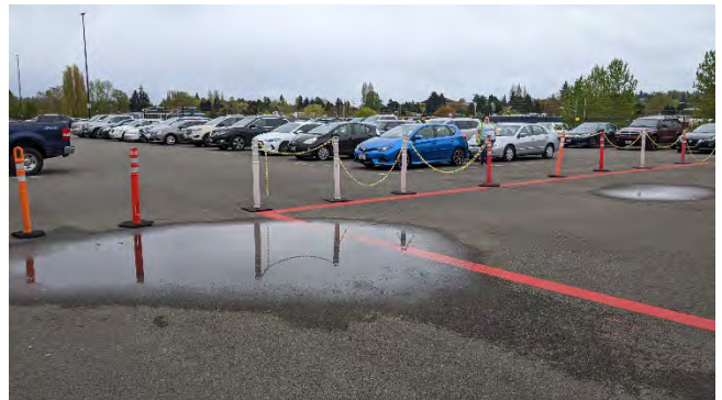
SPPD AC-12: Ponding
