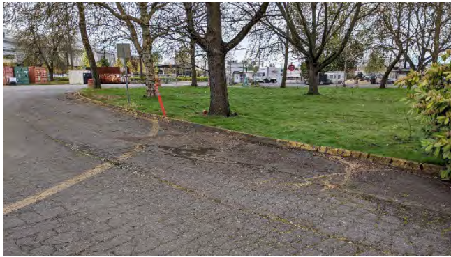
SRDS AC-3: Minor cracking and ponding
