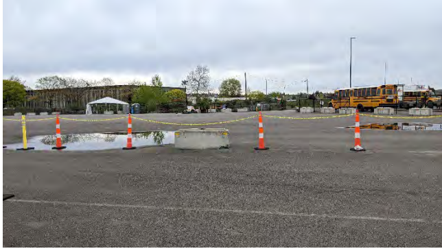
SPPD AC-9: Ponding
