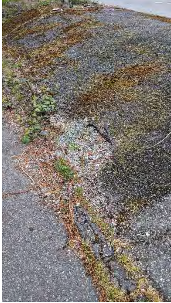
SRDS AC-8: Sinkhole filled with gravel
