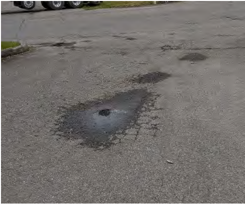
SRDS AC-6: Minor Cracking
