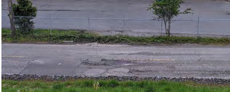
ROW AC-1: Cracks and pavement repair
