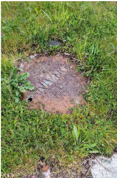
SPPD G-8 Exposed geomembrane around manhole
