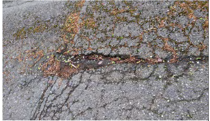
SRDS AC-13: Pavement cracking and rutting
