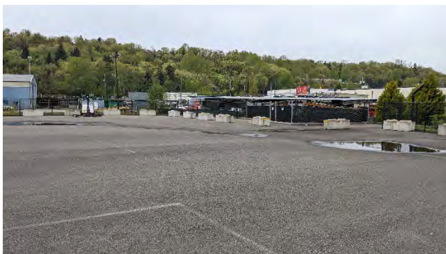
SPPD AC-7: Several areas of ponding
