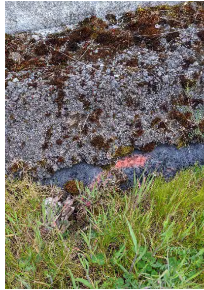
SPPD G-7 Exposed and damaged geomembrane
