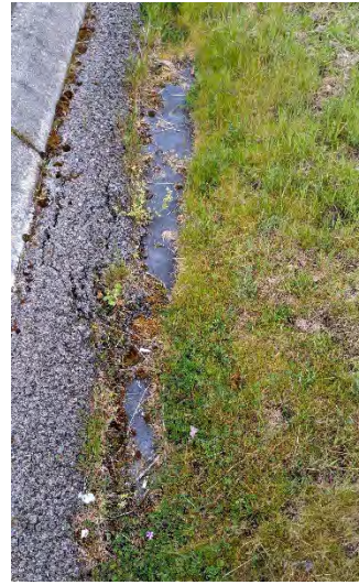
SPPD G-10: Exposed and damaged geomembrane
