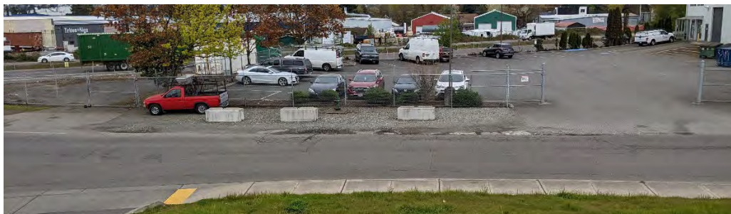
ROW AC-3: Cracking and pot holes
