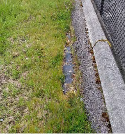
SPPD G-10: Exposed and damaged geomembrane
