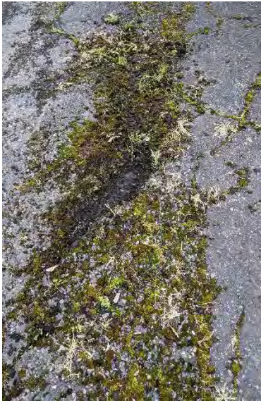
SRDS AC-14: Minor pavement spalling with moss
