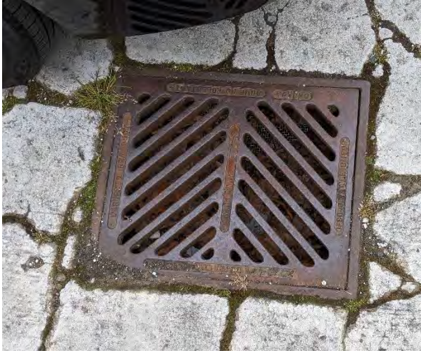
SRDS AC-2: Minor cracking and debris in catch basin
