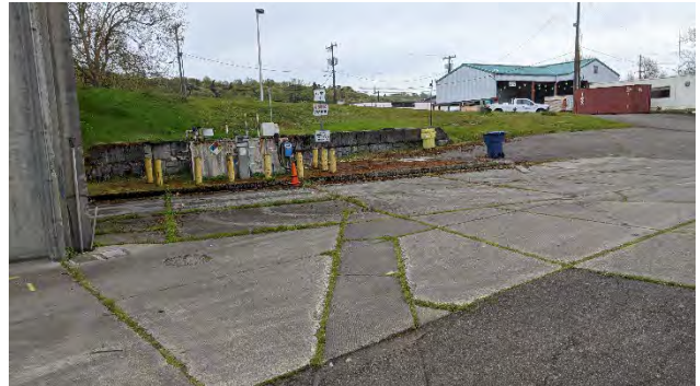
SRDS AC-15: Minor cracking
