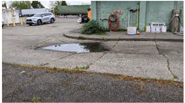
SRDS AC-7: Ponding
