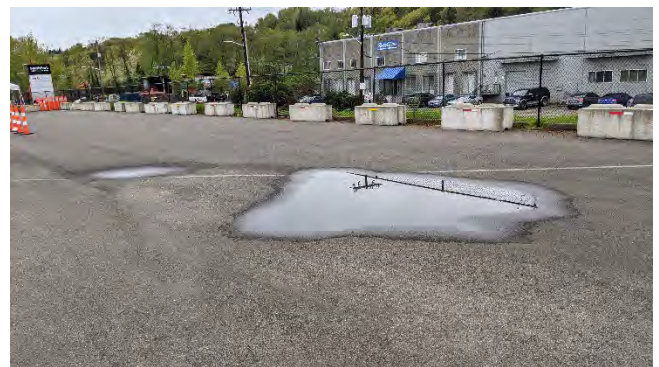
SPPD AC-8: Ponding
