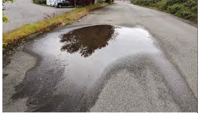
SRDS AC-9: Ponding
