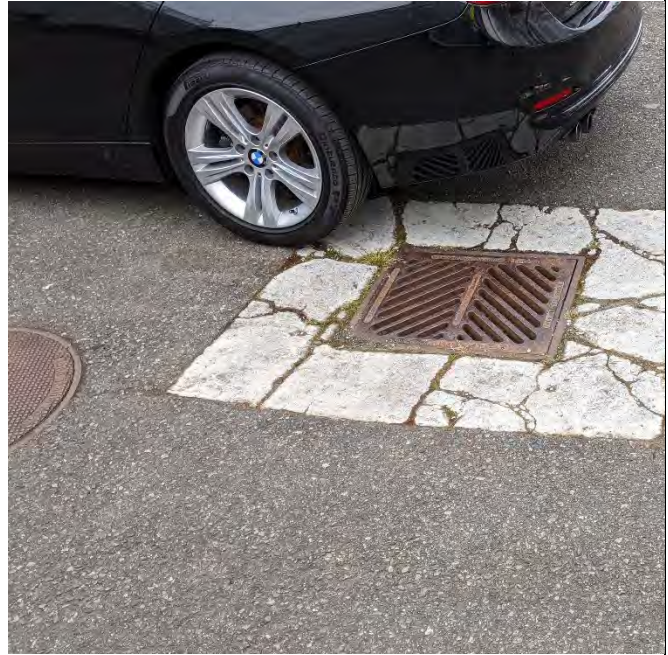
SRDS AC-2: Minor cracking and debris in catch basin
