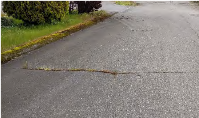
SRDS AC-10: Minor cracking
