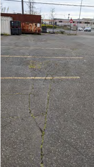
SRDS AC-1: Minor cracking
