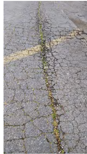
SRDS AC-3: Minor cracking
