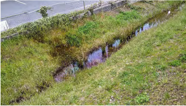
SPPD SW-1: Standing water in north bioswale with sheen
