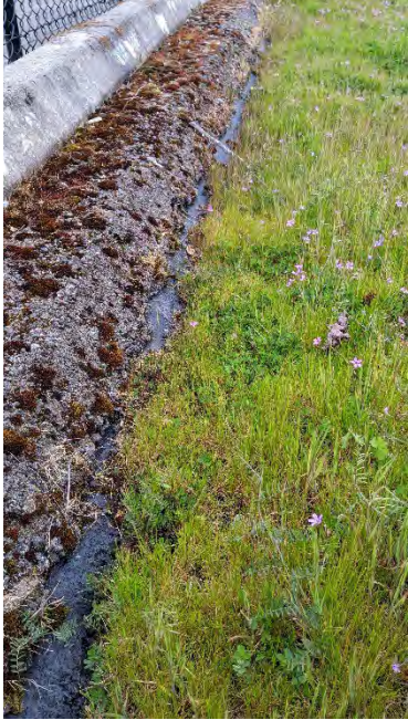
SPPD G-7 Exposed and damaged geomembrane
