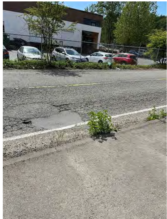
Location 21-20. Open Cracks/Ruts
