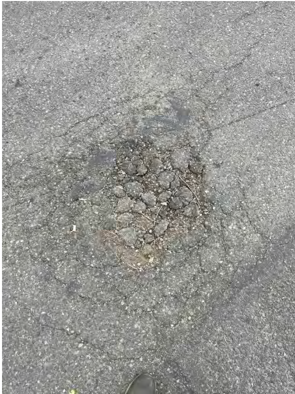
Location 21- 5. Minor Cracking
