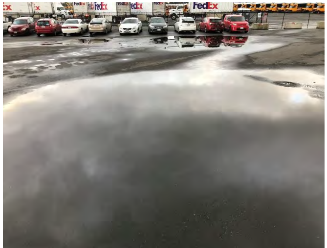
Shallow ponding photographed near 47.5292943, - 122.3321924.
