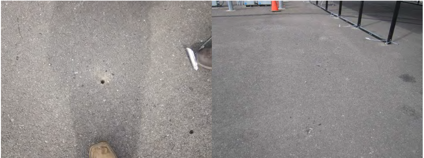
Location 21- 16. Cap Disturbance ( Hole drilled into asphalt to secure tent)
