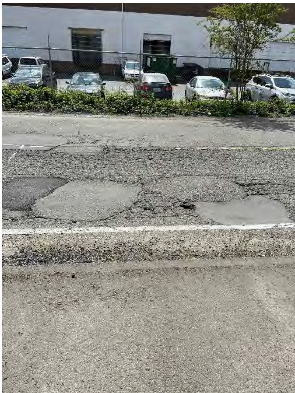
Location 21-20. Open Cracks/Ruts
