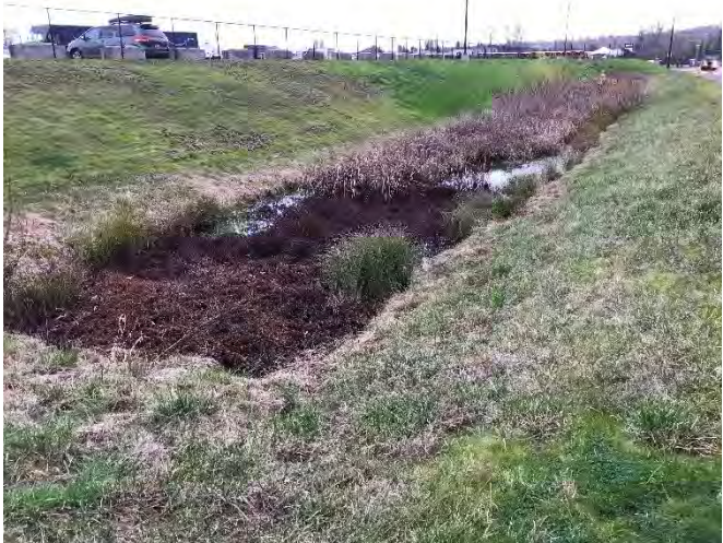
Evidence of swales and conveyance structures flowing as designed. Dredging and removal of sediment accumulation may be recommended. Photographed to the east of GP-11 and MW-12.
