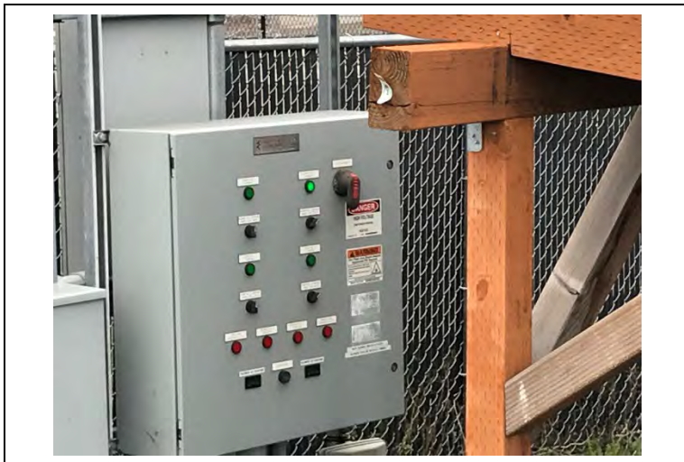
Photo of the gas system control panel taken December 2, 2022. The Blower No. 2 light indicating the system is lit green and the overload light is off.
