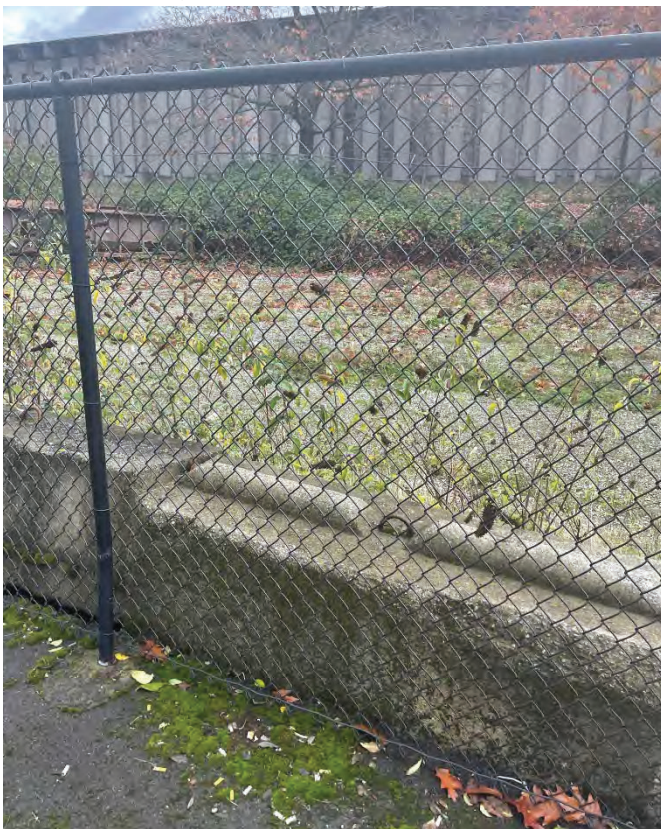
Location 1-3. Fenced area between two parcels View looking East from SPPD towards SRDS
