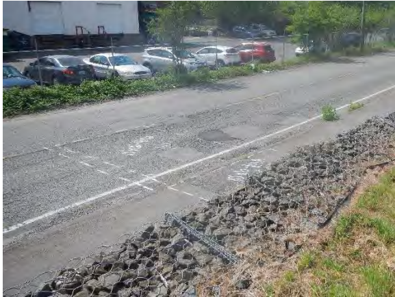
Location 21-20. Open Cracks/Ruts
