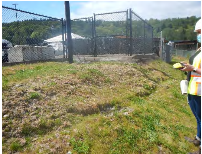
Location 21- 9. Erosion of Soil Cover
