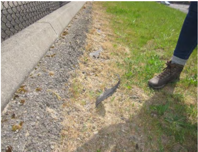
Location 21- 13. Exposed & Damaged Geomembrane
