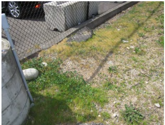
Location 21- 9. Poor Vegetative Cover
