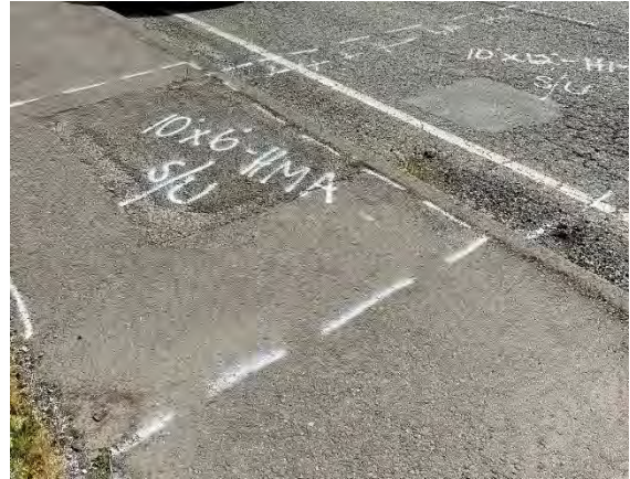
Location 21-20. Open Cracks/Ruts
