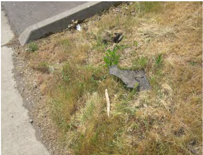
Location 21- 18. Exposed & Damaged Geomembrane
