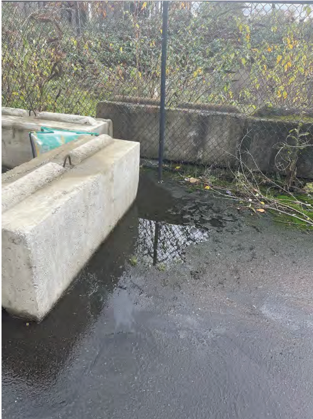
Location 1-1. Pooling/Ponding on Asphalt Concrete View looking East near fenced area with SRDS ahead
