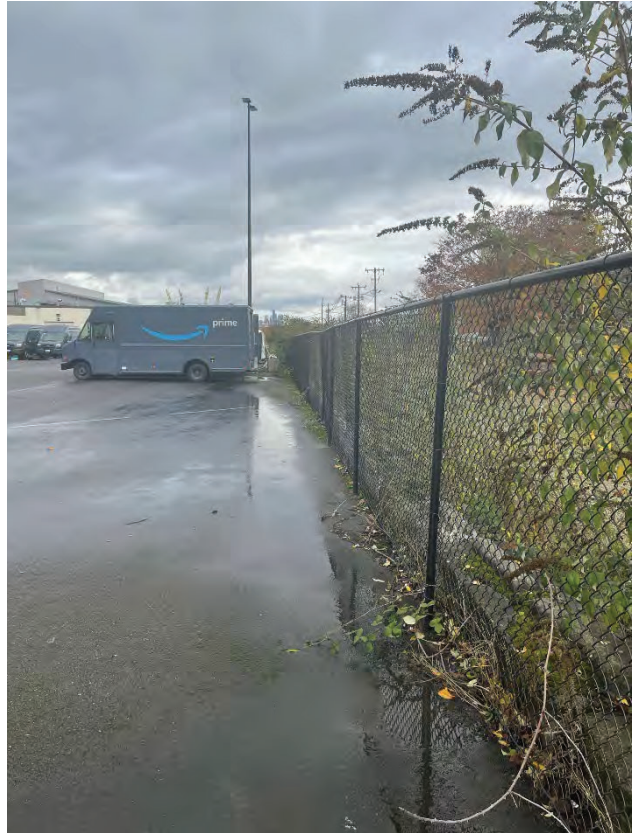
Location 2-1. Pooling/Ponding on Asphalt Concrete View looking North along fenced area, SRDS to right
