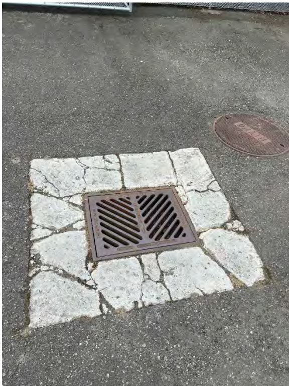
Location 21- 3. Concrete Cracking at Catch Basin
