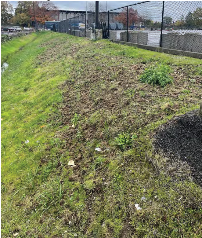
Location 5-2. Poor vegetative cover Zoomed in view of North swale
