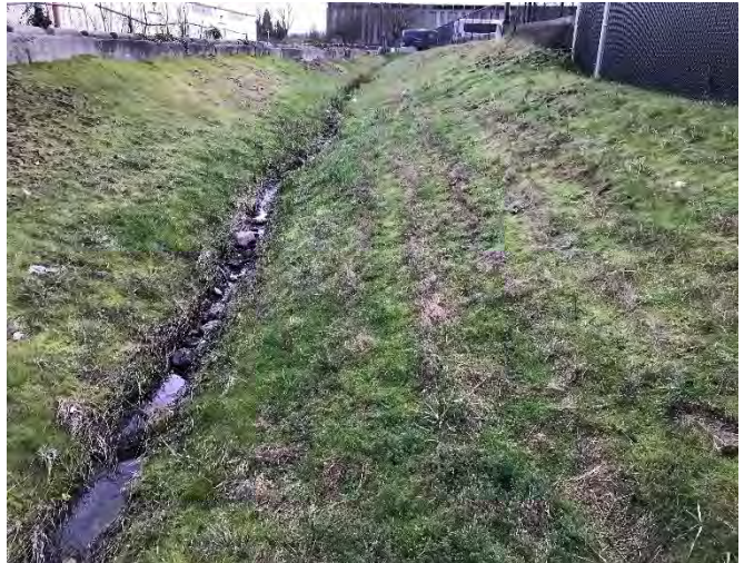
Evidence of swales and conveyance structures flowing as designed. This stormwater feature is experiencing minor erosion and downcutting. Photographed to the east of GP-11 and MW-12.
