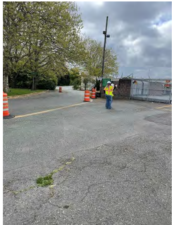
Location 21- 4. Minor Cracking
