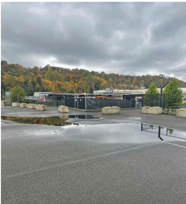
Location 3-1. Pooling/Ponding on Asphalt Concrete View looking North-West from SPPD north swale
