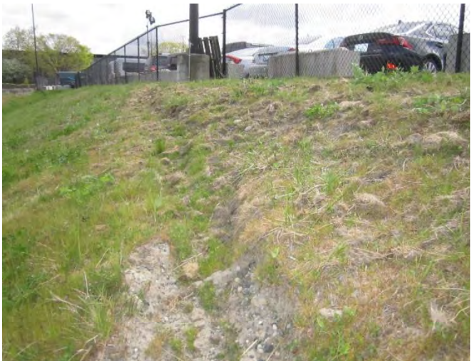
Location 21- 9. Erosion of Soil Cover
