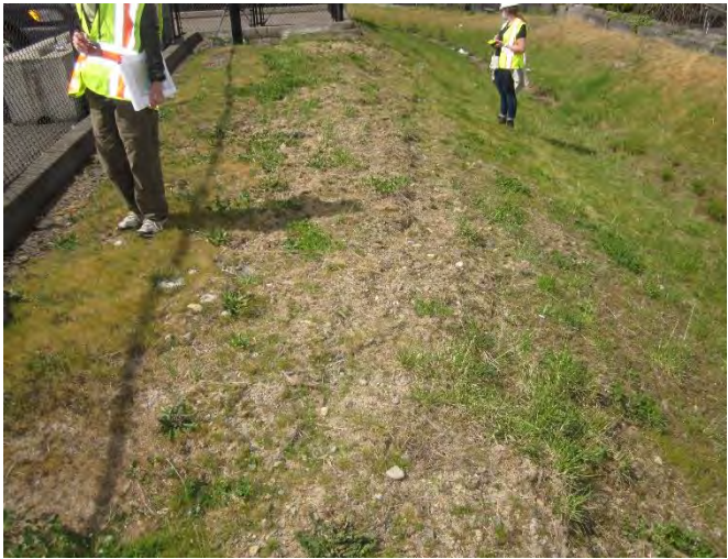
Location 21- 9. Erosion of Soil Cover
