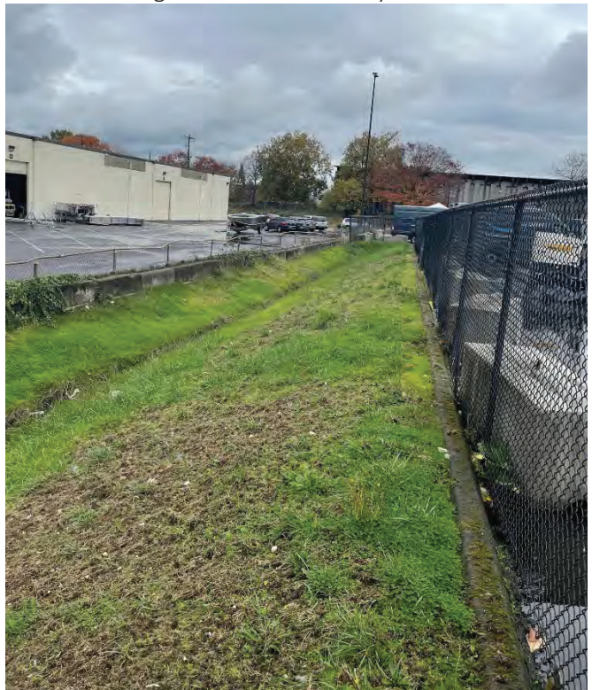
Location 5-3. Poor vegetative cover Zoomed in view of North swale
