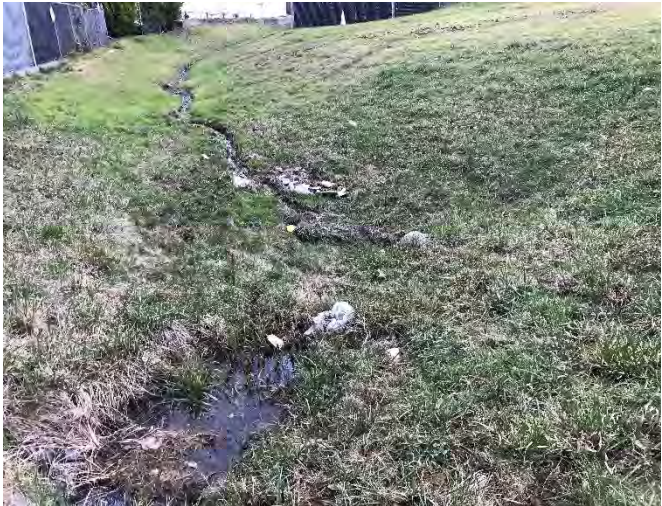
Evidence of swales and conveyance structures flowing as designed. This stormwater feature is experiencing minor erosion and downcutting. Photographed to the east of GP-11 and MW-12.
