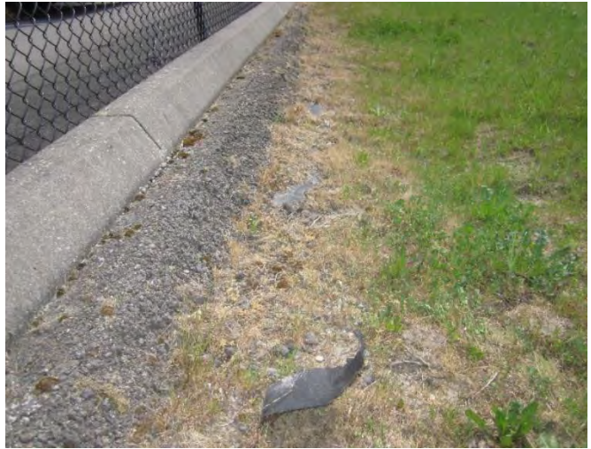
Location 21- 13. Exposed & Damaged Geomembrane
