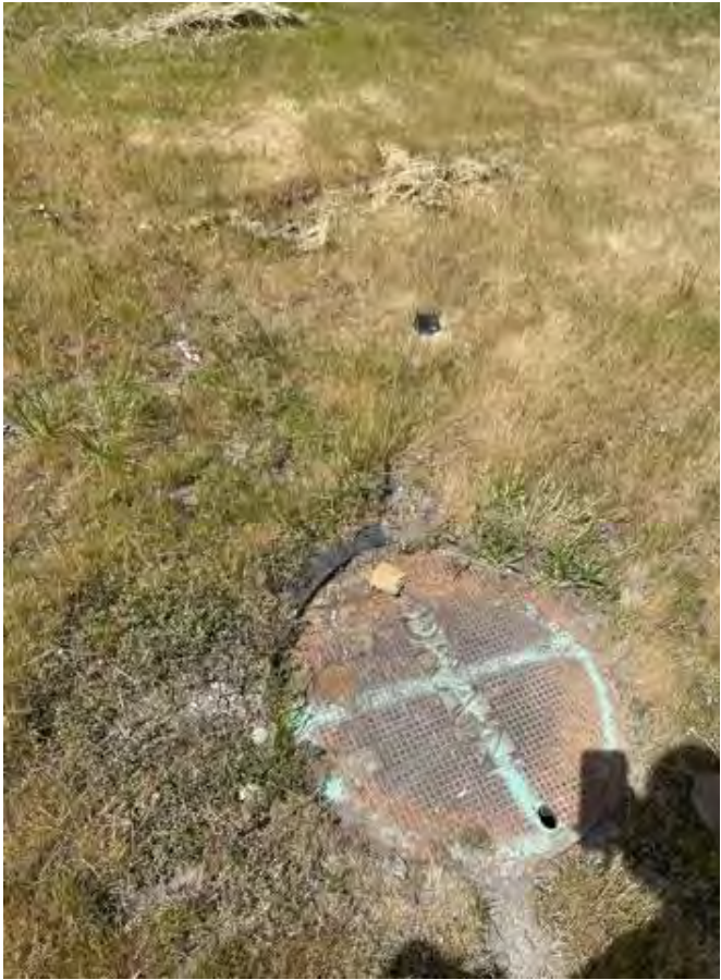
Location 21- 18. Exposed Geomembrane at storm drain structure
