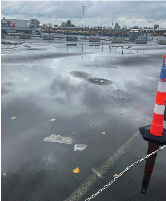
Location 4-2. Pooling/Ponding on Asphalt Concrete View looking South-West from SPPD towards bus lot
