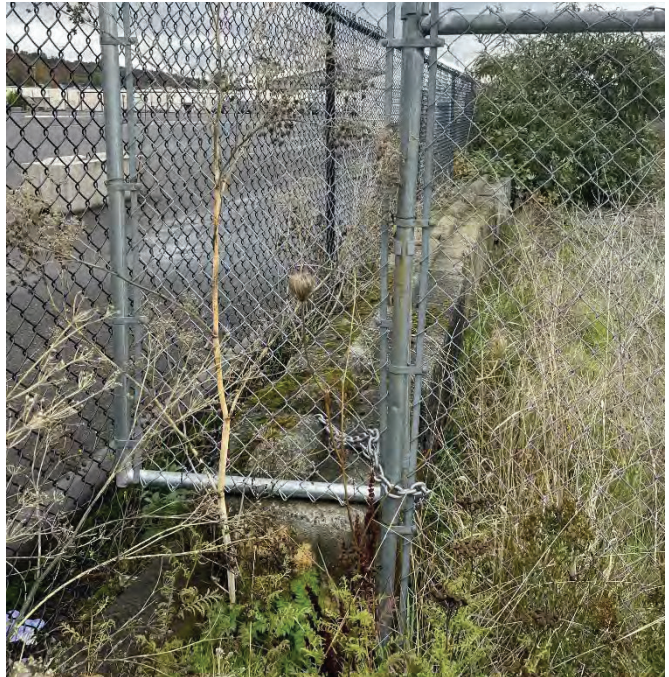
Location 1-2. Fenced area between two parcels Ecology block wall on SPPD side
