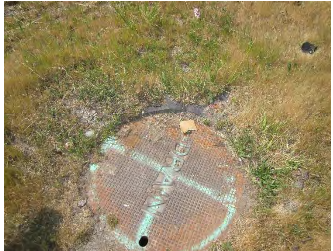
Location 21- 18. Exposed Geomembrane at storm drain structure
