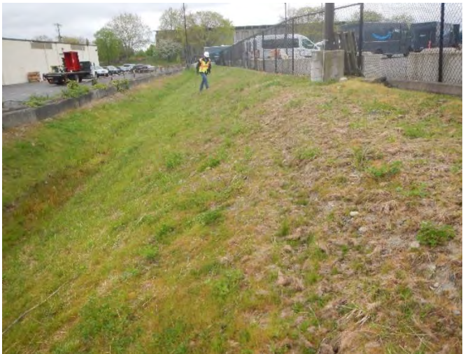
Location 21- 9. Poor Vegetative Cover
