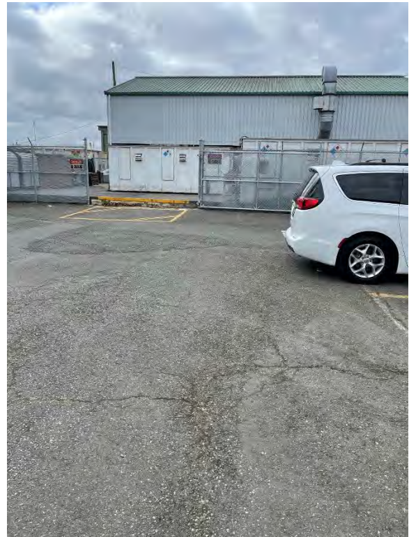
Location 21- 2. Minor Cracking
