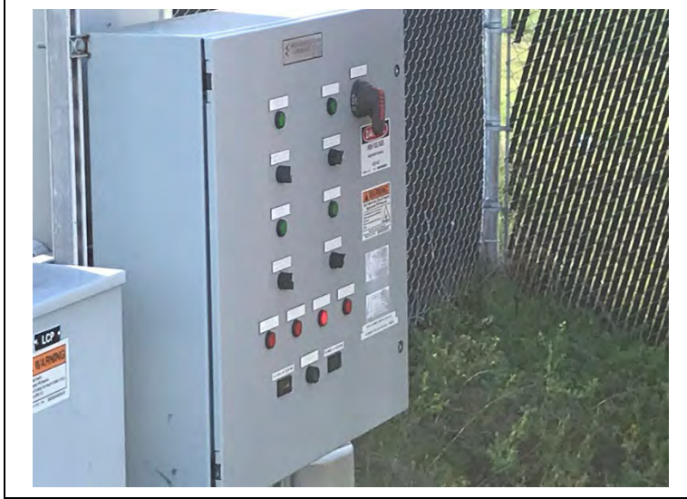
Photo of the gas system control panel taken November 29, 2021. The Blower No. 2 overload light is lit red.
