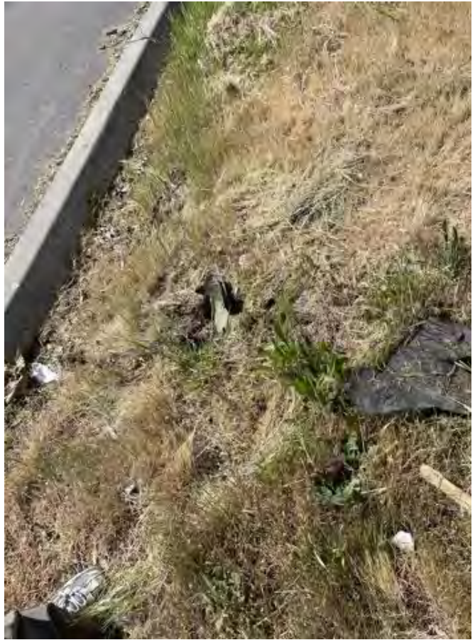
Location 21- 18. Exposed & Damaged Geomembrane
