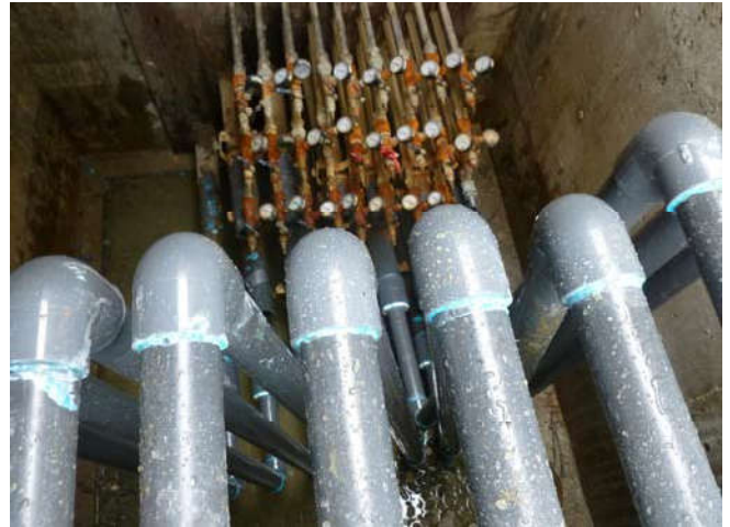
Photo 20 9-6-13: 2" PVC SVE piping is connected to existing 2" PVC SVE well-piping in Mercer Vault. Stainless piping is the existing AS
