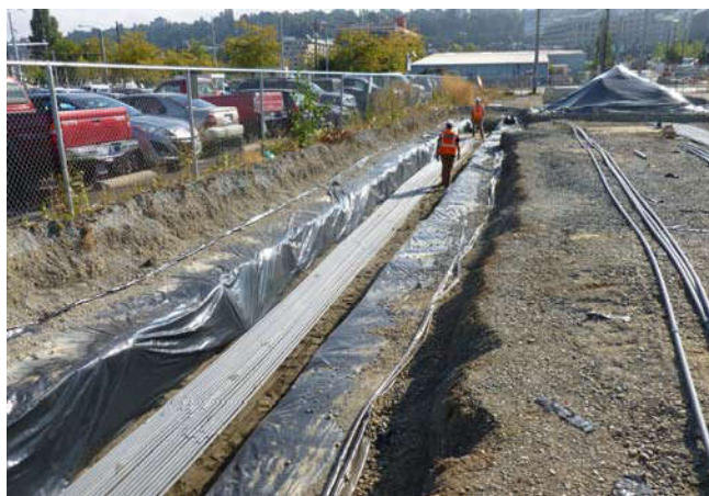
Photo 23 9-10-13: 1" PVC piping for Westlake Avenue AS well-piping being laid in trench, facing east.
