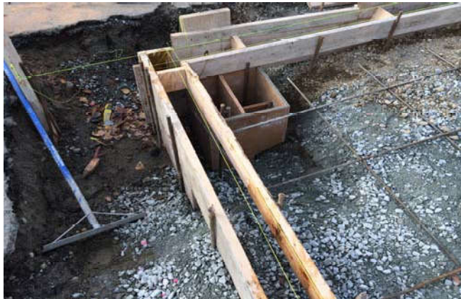
Photo 93 11-4-13: Wood framing around proposed sump area in southwest corner of concrete pad.
