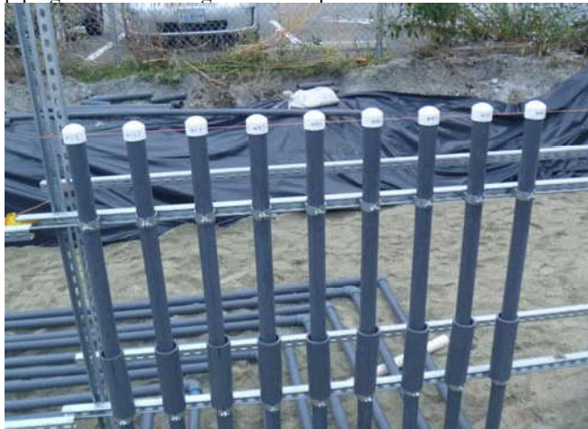
Photo 79 10-18-13: 2" PVC SVE well-piping stub-ups from Westlake Avenue attached to manifold connection area metal framing. Stub-up piping is labeled during connection process.
