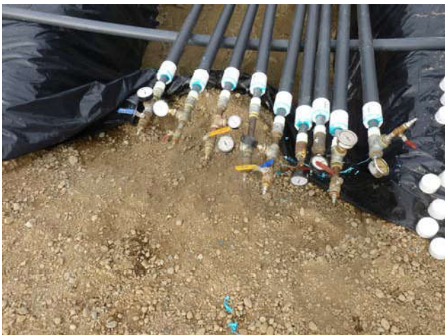
Photo 11 9-3-13: Pressure testing of 2" PVC piping before connecting to existing SVE well piping.
