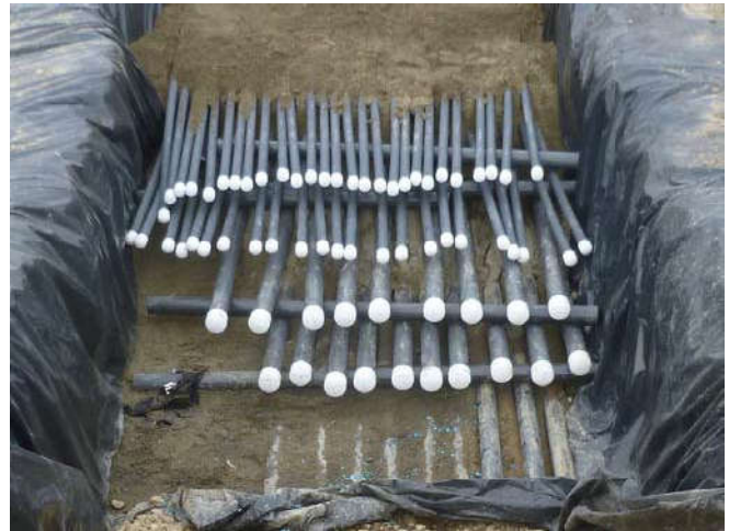
Photo 34 9-12-13: 2" PVC SVE well-piping from Westlake and Mercer Vault is layered beneath 1" PVC AS well-piping from Westlake and Mercer Vault. Sand bedding according to specifications between each layer.
