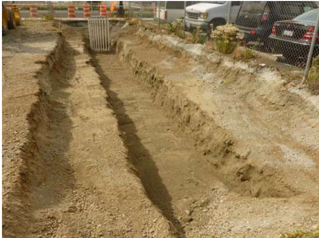
Photo 3 8-27-13: Typical benching of trenches during piping installation activities. View of SVE/AS well piping stub-ups from Westlake Avenue, facing west.
