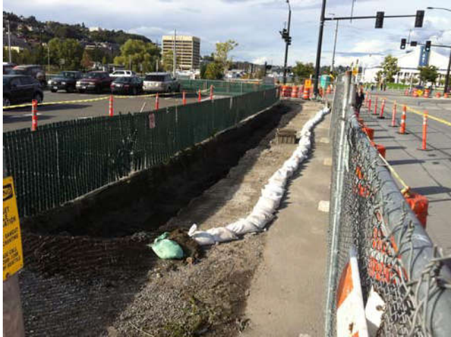
Photo 52 9-24-13: View of erosion control and fencing around Terry Avenue trench, facing north.
