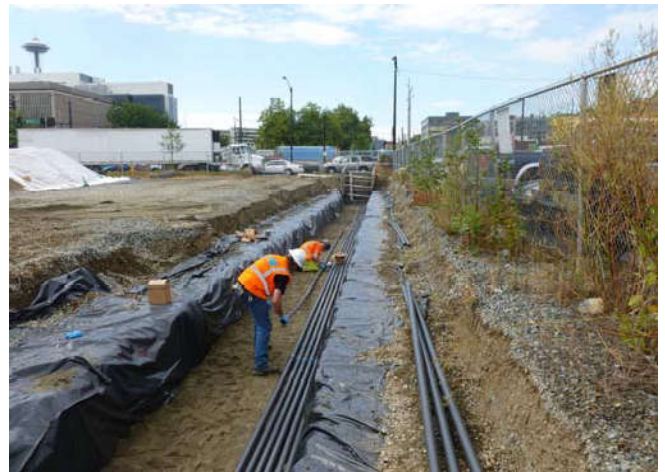
Photo 10 9-3-13: 2" PVC SVE piping being installed on sand bed in trench to connect to existing Westlake Avenue well piping, facing west.
