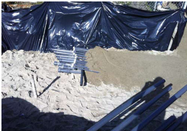
Photo 69 10-7-13: 1" PVC piping is connected to 1" stainless AS piping and pressure tested, labeled and covered in sand bedding.
