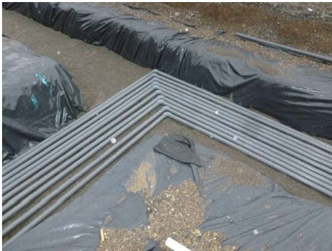
Photo 15 9-6-13: 2" PVC SVE piping from Mercer Vault at T-junction overlaying SVE piping from Westlake Avenue.
