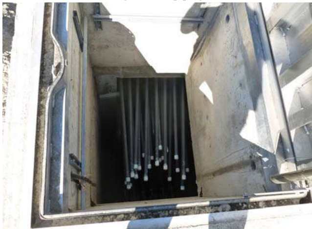
Photo 29 9-10-13: AS piping through concrete form before connecting to existing Mercer Vault AS well-piping.
