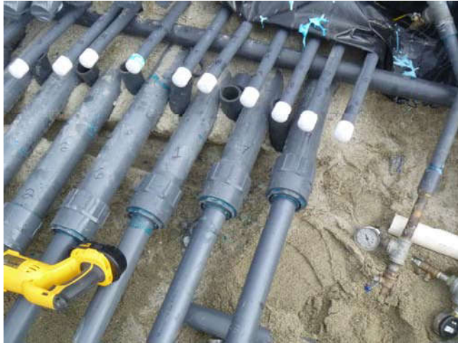
Photo 77 10-17-13: Connecting 2" PVC stub-ups for manifold connection to existing 2" PVC SVE well-piping from Terry Avenue. Stub-up piping is labeled during connection process.
