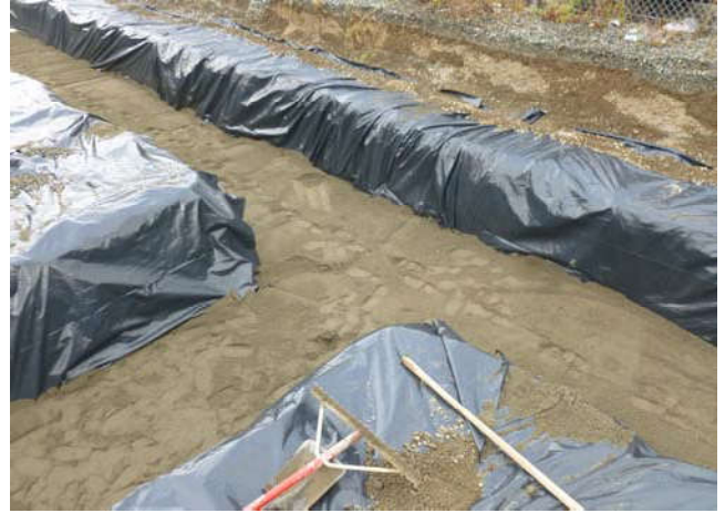
Photo 8 9-3-13: View of typical polyethylene liner with sand bed at T-junction of Westlake and Mercer Trenches on north side of Project Site, facing northwest.
