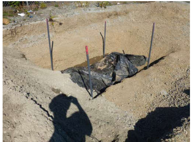
Photo 40 9-12-13: Temporary termination point of installed well-piping, wrapped and demarcated, to be connected to system manifold area.
