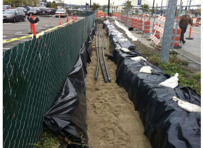
Photo 53 9-25-13: View of Terry Avenue trench lined with poly and bedded with sand. Pedestrian walkway delineated, view facing north.
