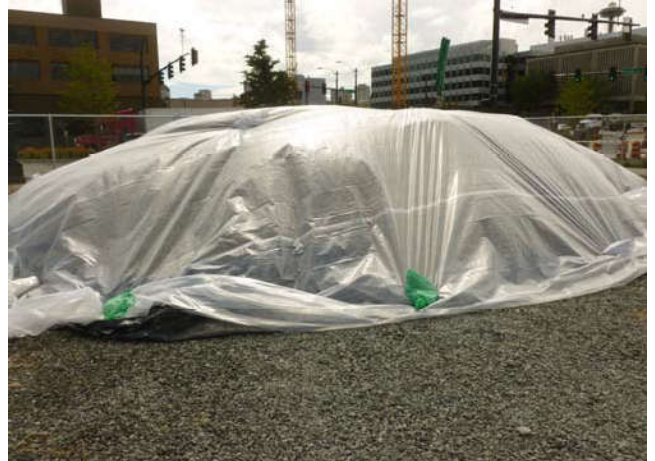
Photo 2 8-27-13: Typical storage of excavated soils covered and stored on polyethylene liner until hauled off site or backfilled.
