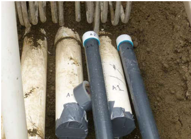
Photo 9 9-3-13: Labeling of new 2" PVC piping in preparation for pressure testing and connection to existing 4" PVC SVE well piping from Westlake Avenue.
