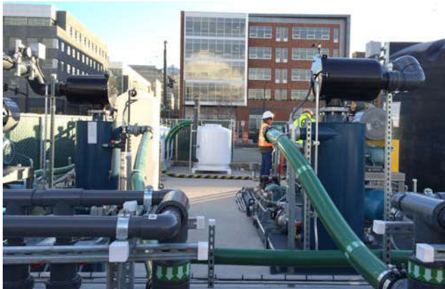
Photo 111 12-2-13: System equipment being connected by Cardno ERI.
