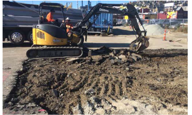
Photo 86 10-28-13: Removal of existing asphalt area to create foundation for system equipment pad.
