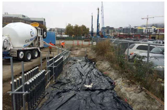
Photo 82 10-24-13: After all AS/SVE piping has been connected, labeled and double checked with Cardno ATC documentation stub-up/manifold connection area is wrapped with poly-liner and backfilled with CDF.
