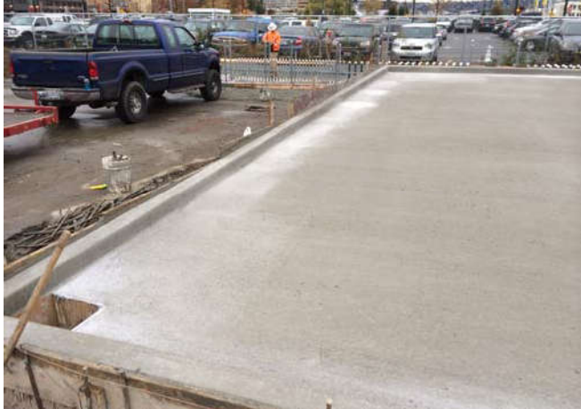
Photo 95 11-5-13: Concrete pad, after pouring and spreading, waiting to dry, view facing north.
