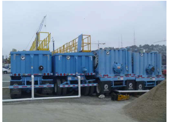
Photo 74 10-17-13: GLY Construction places storm water tanks on site west-adjacent to system installation area.
