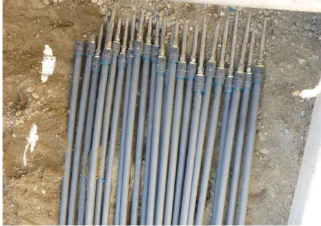
Photo 25 9-10-13: 1" PVD AS piping connected to existing 1" stainless AS well-piping from Westlake Avenue.
