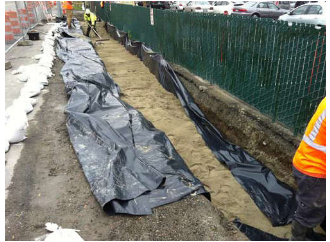
Photo 60 9-27-13: AS and SVE piping is covered in sand and wrapped in poly-liner after connected to existing well-piping.
