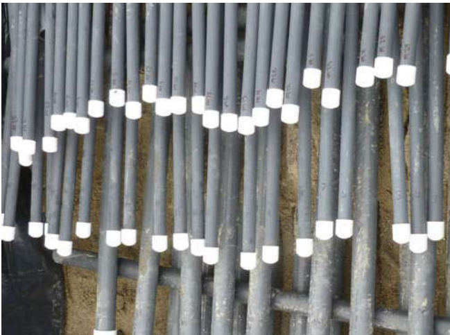
Photo 35 9-12-13: All installed piping is labeled as it is connected to existing well-piping.
