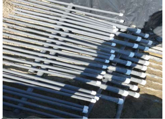
Photo 26 9-10-13: Westlake Avenue and Mercer Trench well-piping layered with sand bedding and labeled during connection to existing well-piping.
