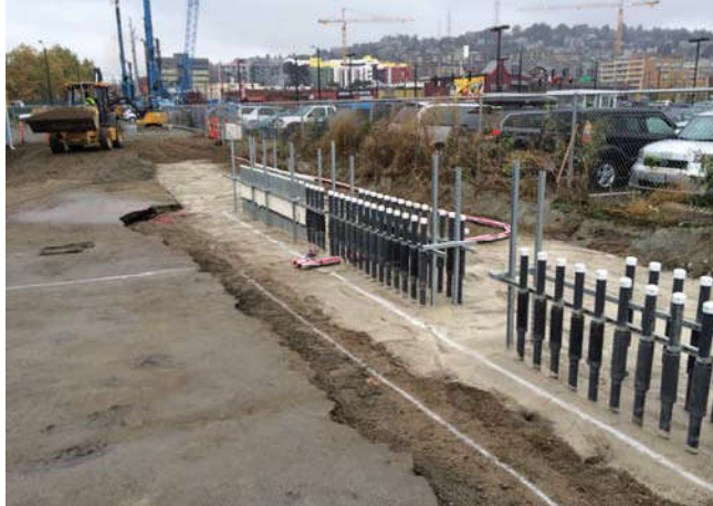
Photo 83 10-25-13: Stub-up area backfilled with CDF. Electrical conduit for remediation system installed above CDF, facing west.
