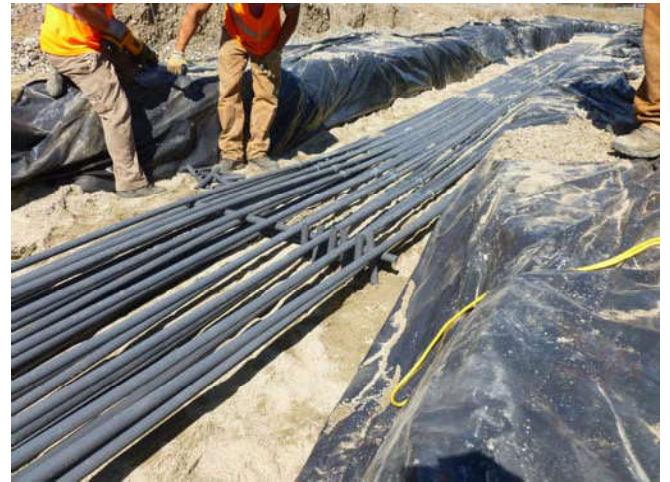
Photo 28 9-10-13: AS piping from Mercer Vault layered and organized during connection and pressure testing.
