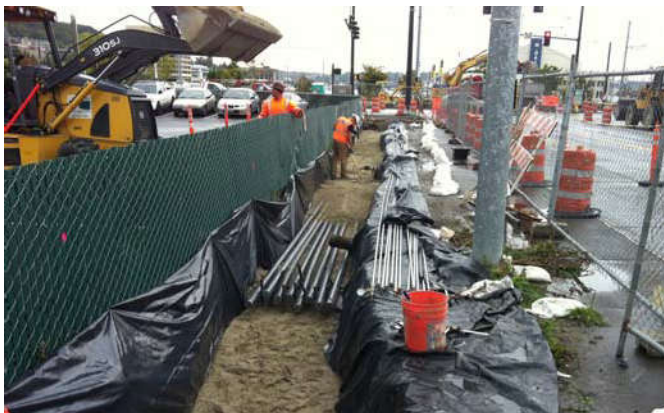
Photo 56 9-27-13: SVE piping covered with sand in preparation for installation of 1" stainless AS piping.
