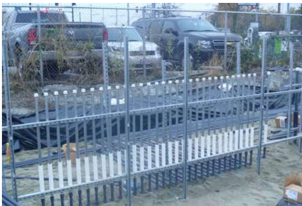
Photo 81 10-22-13: 1" PVC AS piping is connected to 1" stainless steel stub-up piping in manifold connection area.
