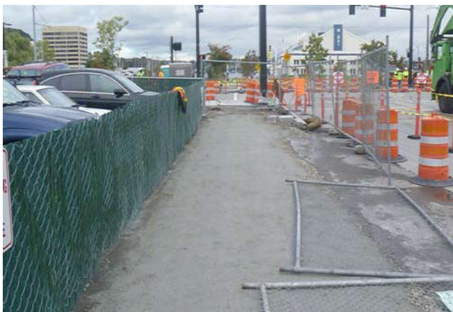
Photo 63 10-1-13: Exclusion zone fencing is moved south along Terry Avenue in anticipation of trenching activities.
