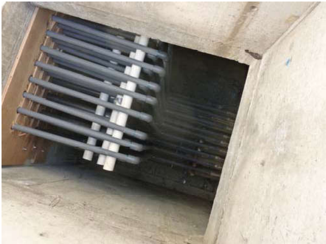
Photo 33 9-11-13: 1" PVC AS piping connected to 1" stainless well-piping inside Mercer Vault.
