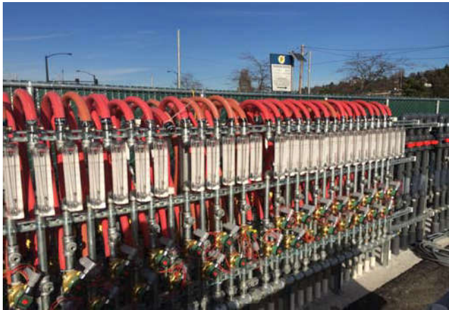
Photo 109 11-22-13: AS manifold and flow meters connected to AS conveyance piping.
