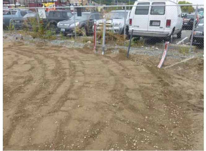
Photo 44 9-17-13: View of compacted fill over well-piping and electrical conduit, view facing northwest.
