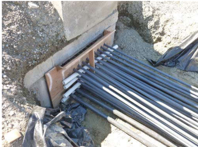
Photo 27 9-10-13: Mercer Vault AS piping is organized through concrete form to connect to existing AS well-piping.
