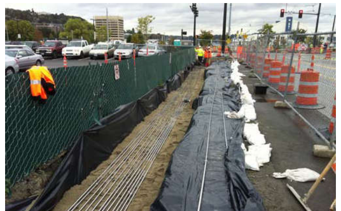
Photo 57 9-27-13: AS piping layered on top of sand bed over connected SVE piping.
