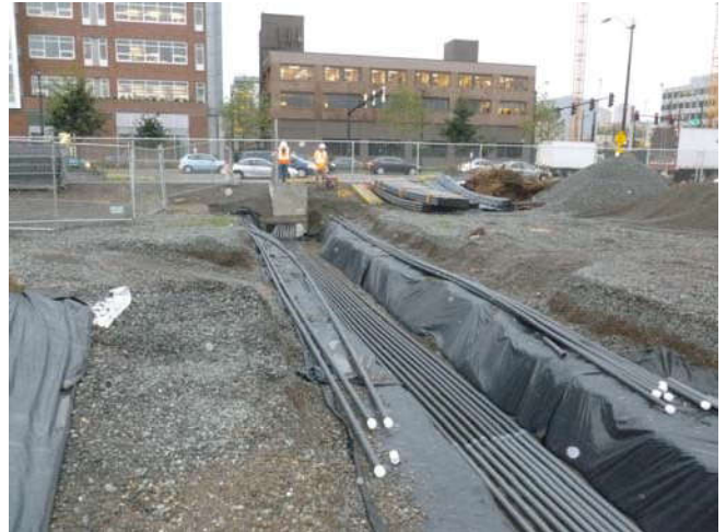
Photo 14 9-6-13: 2" PVC SVE piping from Mercer Vault layered over sand bed in trench.
