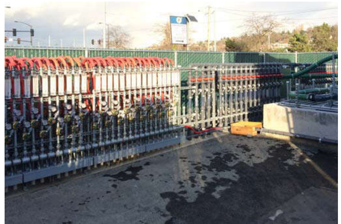
Photo 110 12-2-13: AS and SVE manifold connected to remediation system.
