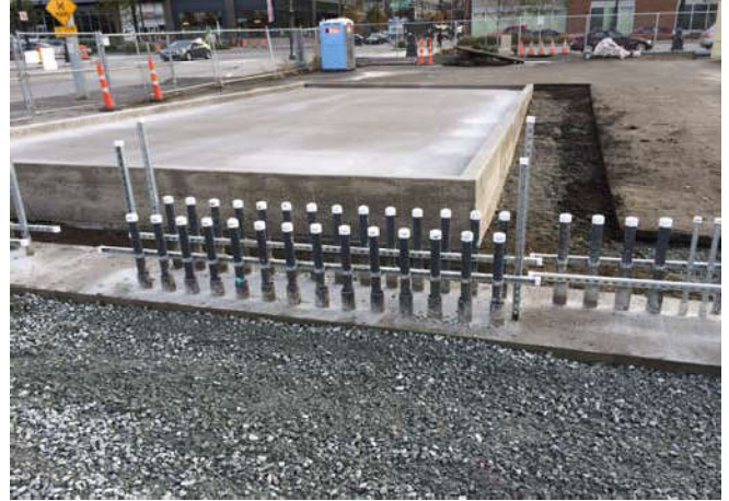
Photo 96 11-5-13: Concrete equipment pad and concrete pad around well-piping stub-ups, view facing south.
