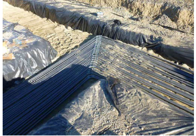
Photo 32 9-11-13: Final layout of AS piping from Mercer Vault layered over sand-bedded Westlake piping at T-junction.
