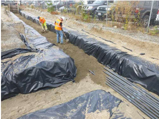
Photo 13 9-4-13: Connected 2" PVC SVE well piping is covered in sand bed after being attached to existing well piping.
