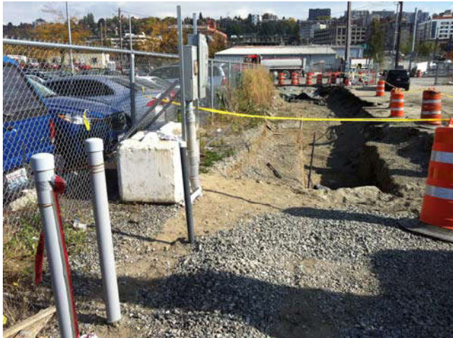
Photo 73 10-10-13: View of electrical box and manifold area trench, facing east.
