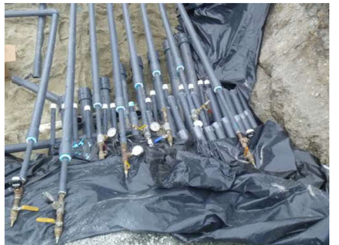
Photo 76 10-17-13: Pressure testing of 2" PVC stub-up piping for before connecting to 2" PVC SVE well-piping from Terry Avenue
