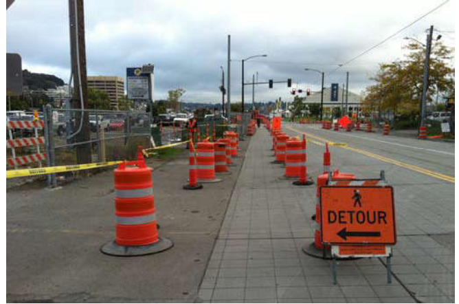
Photo 47 9-23-13: Traffic control and delineation around work area in Terry Avenue right-of-way, facing north.
