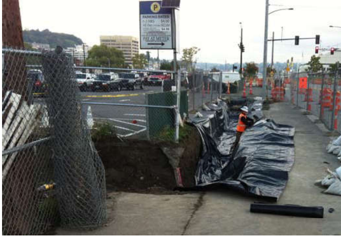
Photo 65 10-3-14: Terry avenue trench is continued onto east side of project site. Trench is lined with poly-liner.
