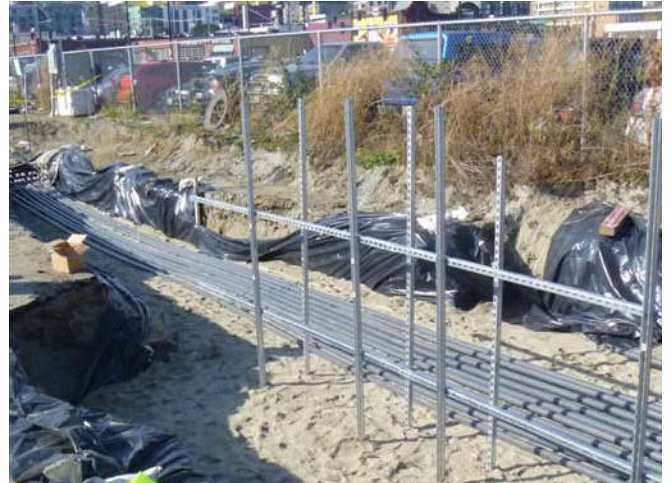
Photo 78 10-17-13: 2" PVC SVE well-piping from Westlake Avenue extended to stub-up manifold connection area.
