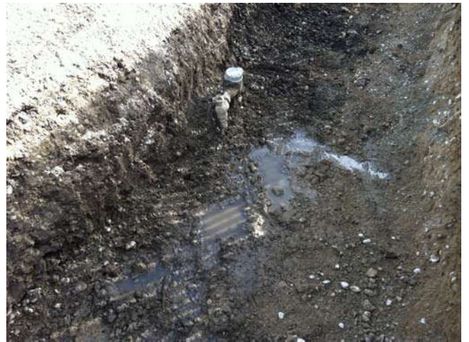
Photo 51 9-24-13: Unearthed historically leaking City of Seattle water line. City of Seattle is contacted for repairs.
