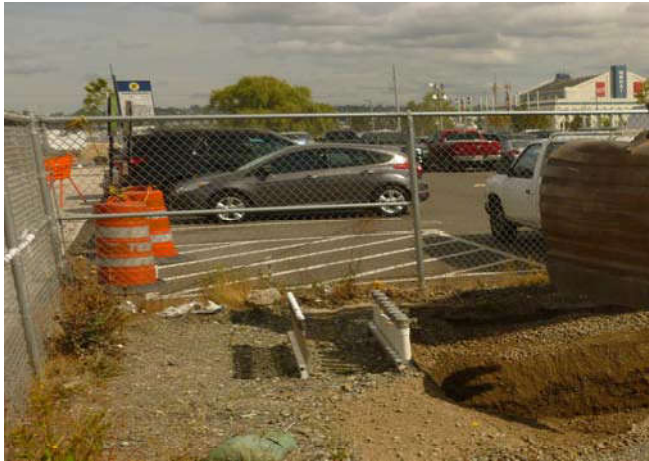
Photo 1 8-27-13: SVE and AS stub-ups from existing Westlake Avenue well piping during beginning of excavation activities in the northwest corner of Project Site. View facing north.
