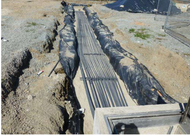
Photo 31 9-11-13: Final layout of AS piping from Mercer Vault after pressure testing and connecting to existing well-piping.
