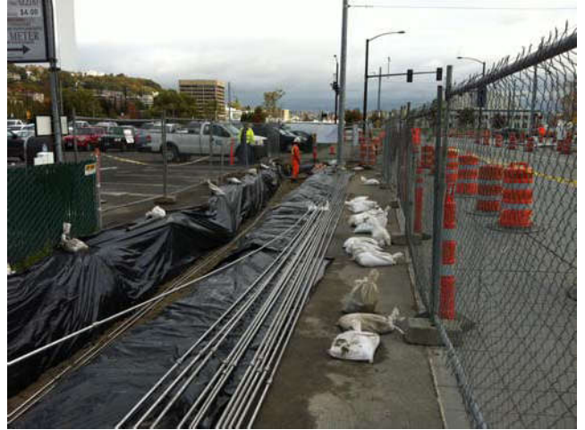
Photo 68 10-7-13: 1" stainless AS piping is installed in trench above sand bed and SVE piping.
