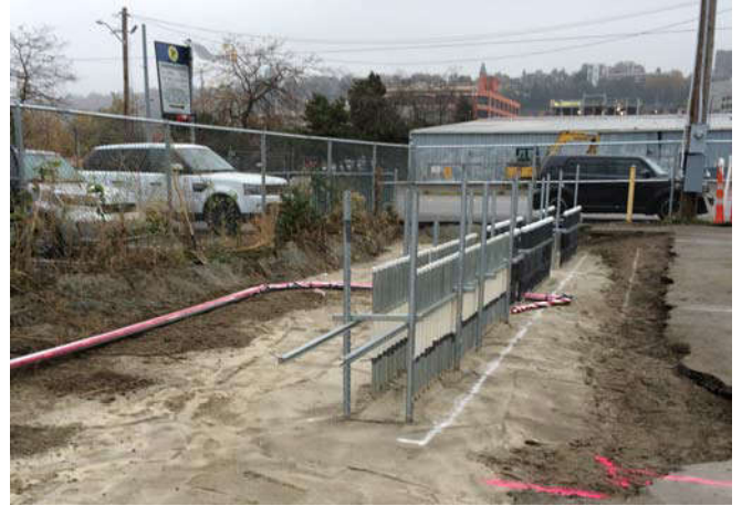
Photo 84 10-25-13: Stub-up area backfilled with CDF. Electrical conduit for remediation system installed above CDF, facing east.
