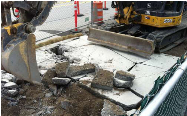
Photo 48 9-24-13: Breaking up concrete slab at south end of Terry Avenue to unearth existing remediation well-piping and begin trenching activities.
