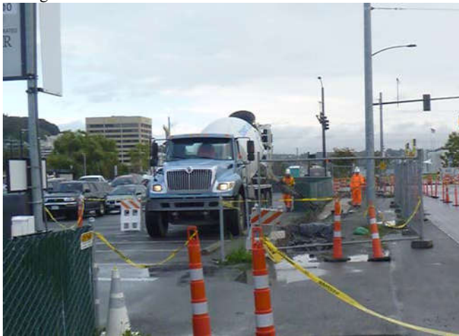
Photo 61 9-30-13: CDF is poured over installed piping, view facing north along Terry Avenue.
