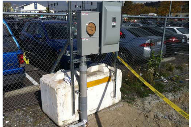
Photo 72 10-10-13: Power junction box is installed by Seattle City Light at north side of site connected to previously installed electrical conduit.
