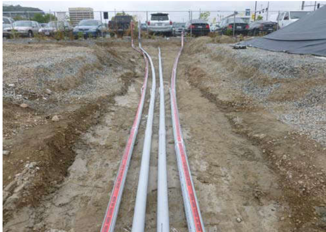
Photo 41 9-13-13: Electrical conduit with detection/hazard tape installed on top of CDF in trench north-adjacent to Mercer Vault, view facing north.
