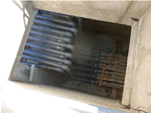
Photo 19 9-6-13: Pressure tested 2" PVC SVE piping is attached to SVE well-piping inside Mercer Vault.
