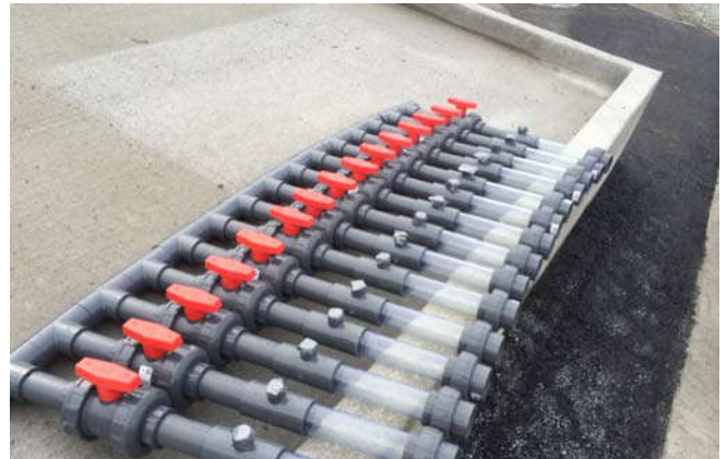
Photo 100 11-7-13: PVC SVE manifold.
