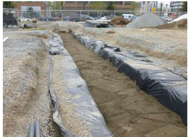
Photo 36 9-12-13: Trenches are backfilled with sand after AS and SVE well-piping has been installed and connected.
