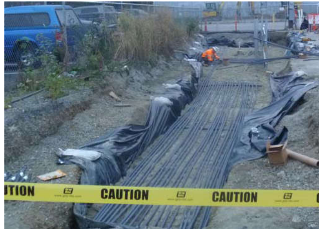
Photo 80 10-22-13: 1" PVC AS well-piping from Westlake Avenue is connected to stub-up piping at manifold connection area.
