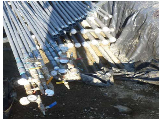
Photo 30 9-10-13: Mercer Vault AS piping being pressure tested before connecting to existing AS well-piping.
