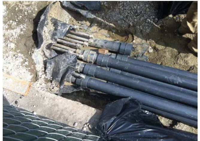
Photo 55 9-26-13: 2" PVC SVE piping being connected to 2" PVC existing SVE well-piping after pressure testing. 1" stainless AS well-piping located above.
