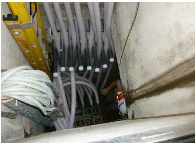
Photo 17 9-6-13: Confined space entry into Mercer Vault to attach pressure tested PVC piping to existing SVE well piping.
