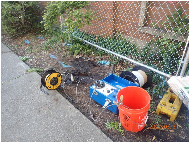
New monitoring well EMW01 being developed on June 2, 2022.
