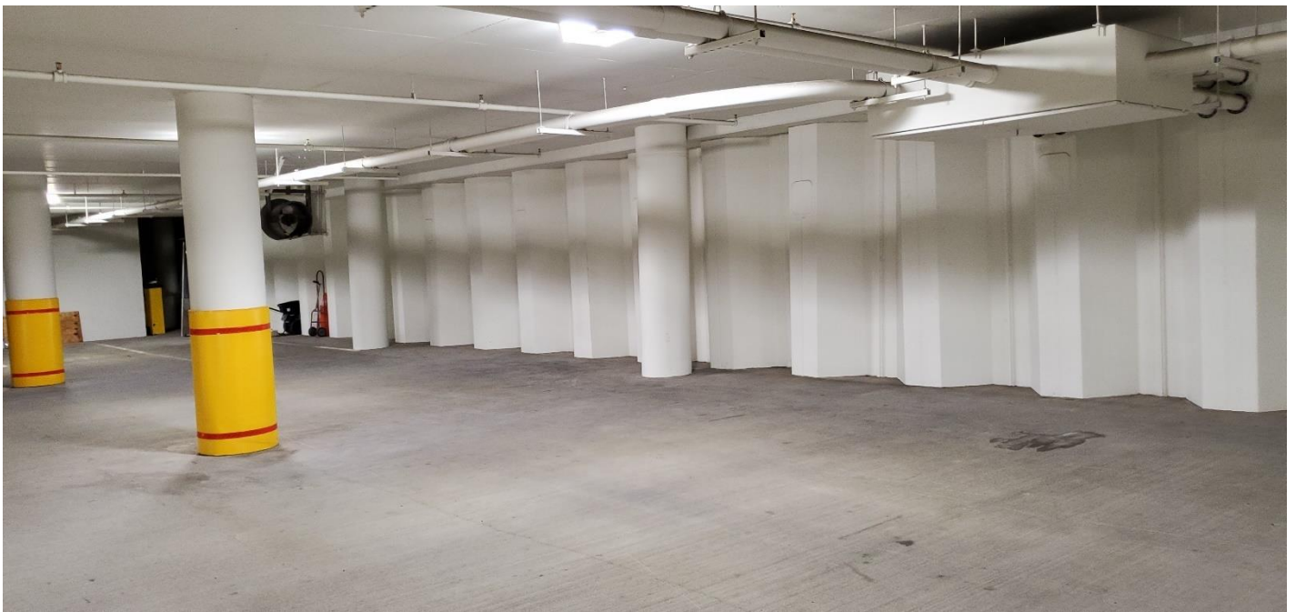
Photograph 4. Steel sheet pile walls in the parking garage. No damage or areas of concern were observed.
