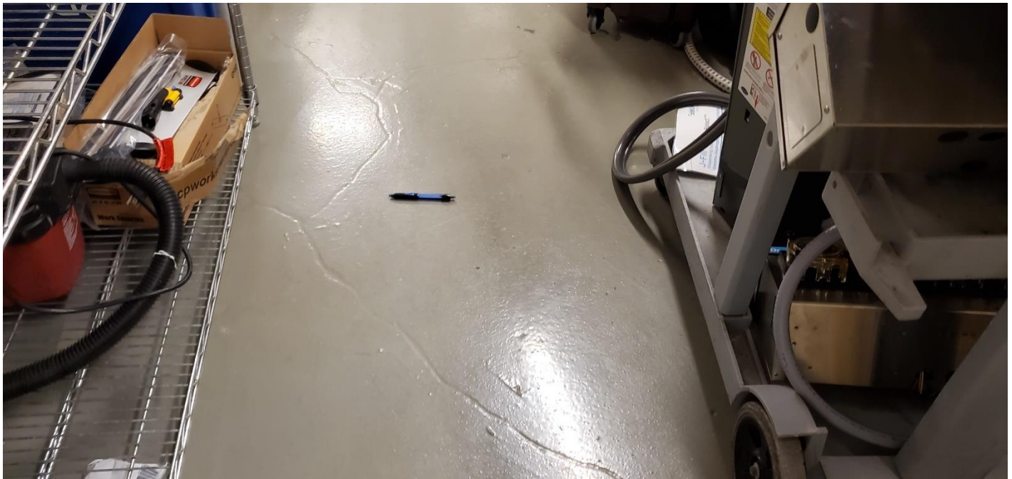
Photograph 5. Nonstructural cracking within the maintenance areas sealed by epoxy paint.
