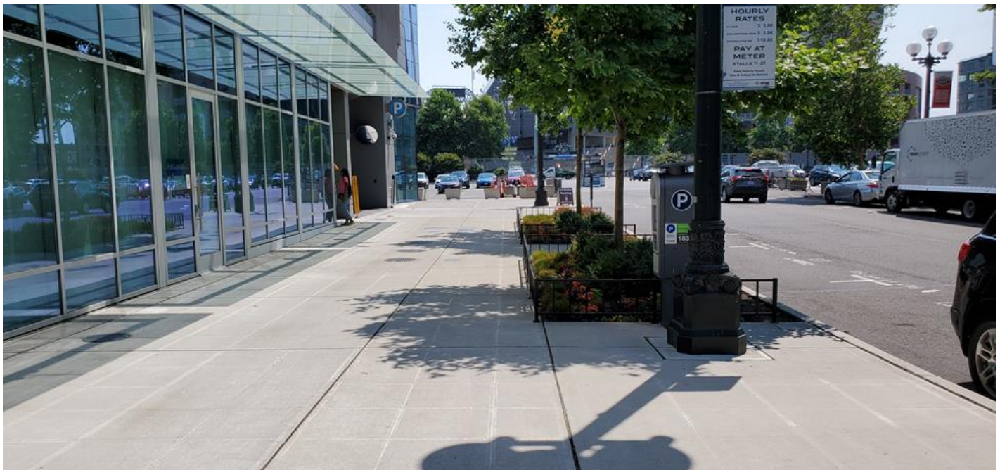
Photograph 2. Western concrete path surface conditions.
