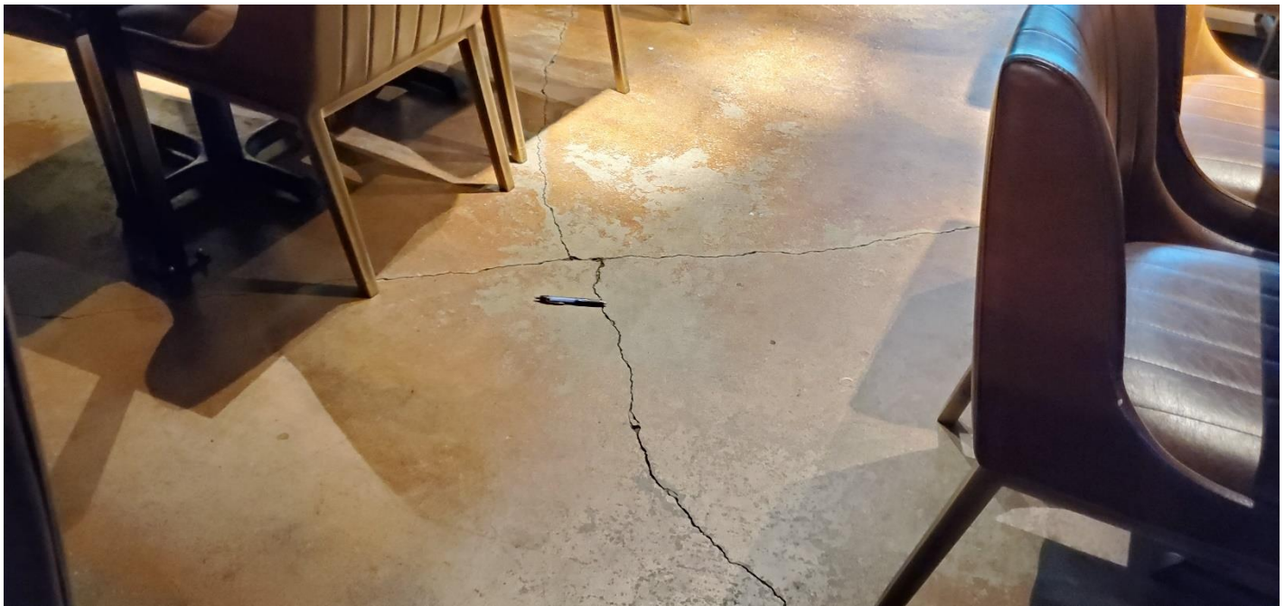
Photograph 6. Significant cracking in the northwestern portion of the 13 Coins Restaurant on the King Street property.
