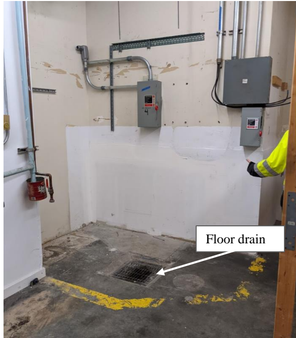
Photograph 3. Floor drain identified in C-1 Building near in office areas near sample location IA-9. No strong odors were observed.
