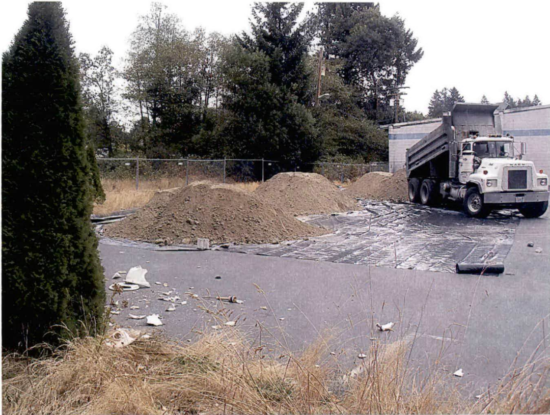
Photo 7. View looking to the northeast showing the temporary soil stockpiling area. Four separate stockpiles (each from a different portion of the excavation) were kept over plastic containment pending characterization and disposal.
