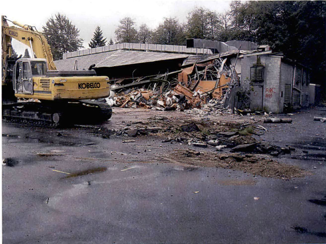
Photo 2. View looking south immediately after the demolition of the northern section of the supermarket building. The northwest building extension was previously situated immediately to the west (right) of the excavator.
