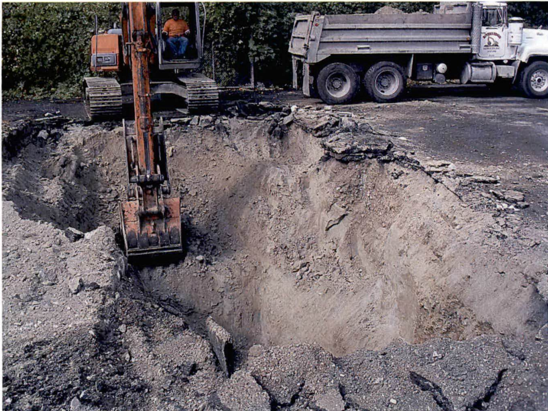
Photo 6. View looking west showing soil removal along the western end of the remedial excavation. The excavated soils were hauled to an adjacent stockpiling area.
