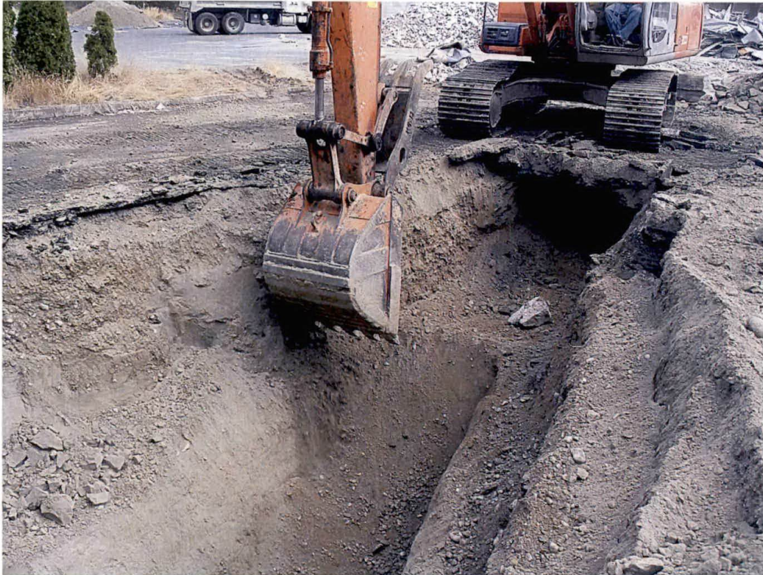
Photo 5. View looking northeast during the excavation of the deeper (6-9 feet bgs) horizons of the remedial excavation.
