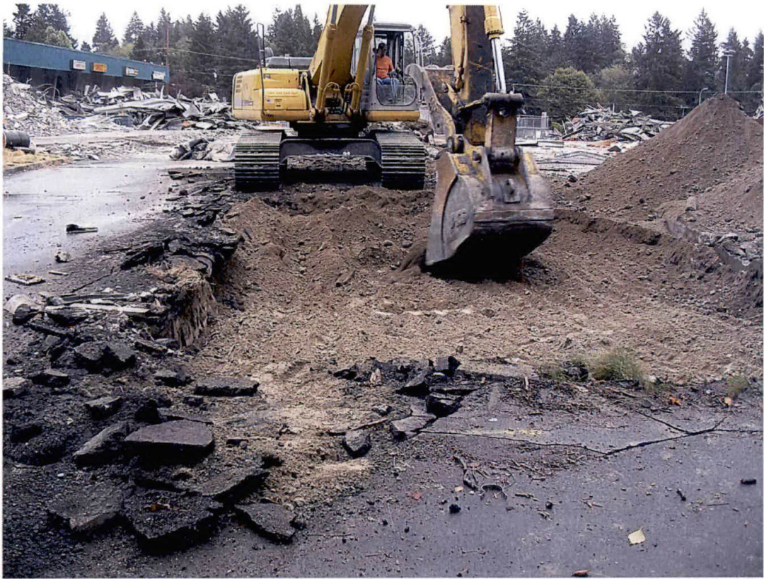
Photo 3. Easterly view showing the removal of the covering asphalt and the shallow overburden soils from the remedial excavation.
