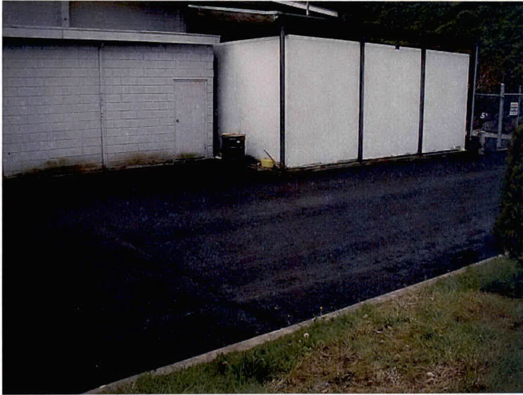
Photo 1. View towards the southwest showing the structural extension attached to the northwest corner of the former supermarket building.
