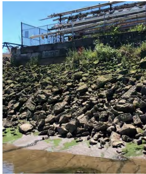
Photograph 2. Ecology block wall and riprap at SPM southeast corner, lower-low tide stage.
