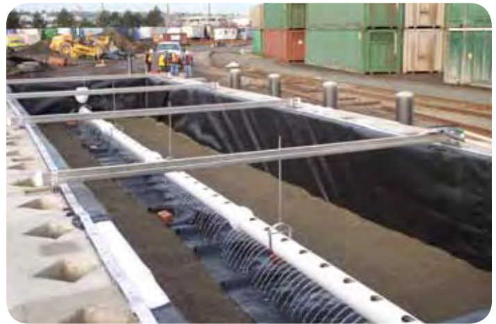
View of Aquip inlet distributor
