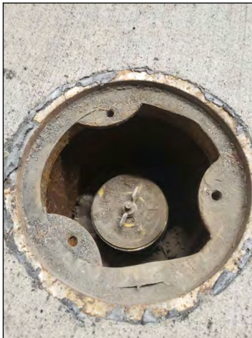
Photograph 8: View of RW2 well casing.
