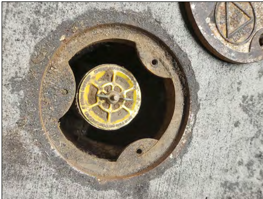
Photograph 6: View of RW1 well casing.
