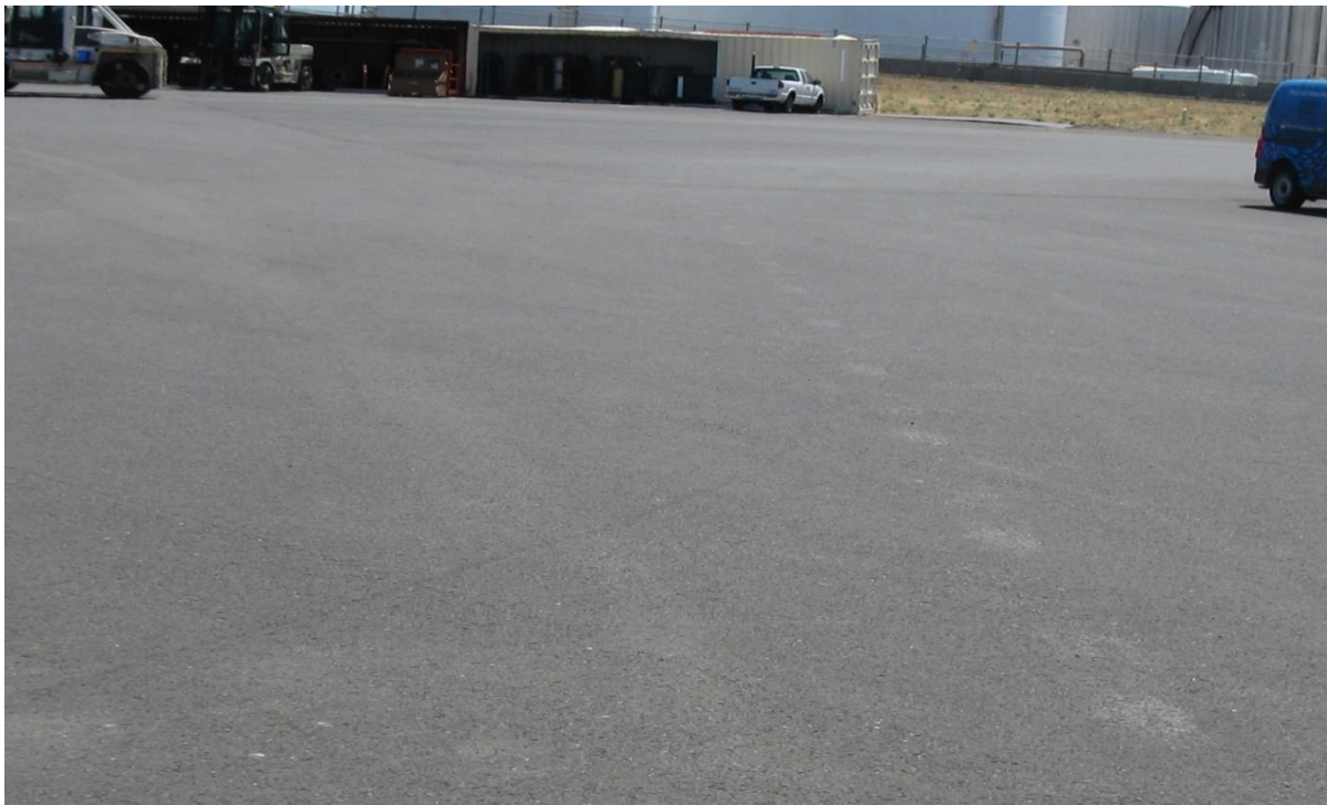
Photo 4: Former pond area and engineered asphalt cap and new building—from the Southeast.
